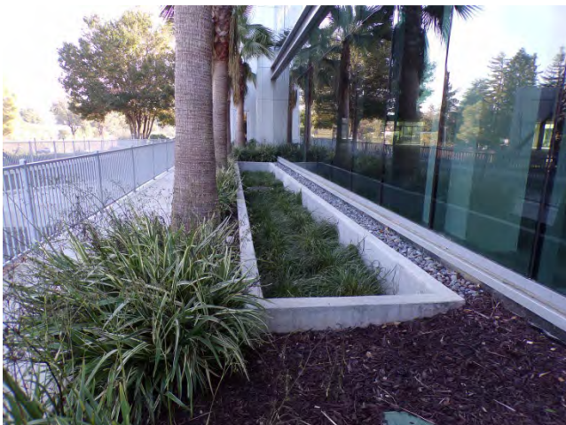
17. Storm water runoff is filtered by biotreatment areas located in treatment planters.
