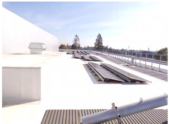
30. The raised platform for the elevator machine equipment is shown at left.
