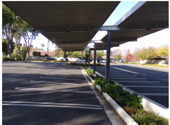
22. Eight steel-framed canopies are provided; each has a solar array on its roof.
