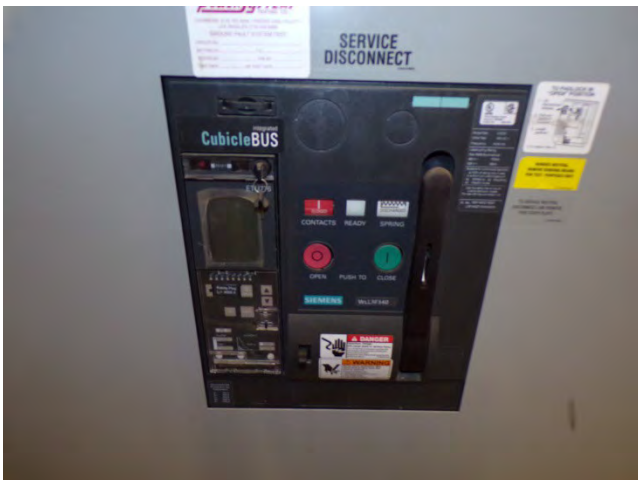
77. The main circuit breaker is rated at 4,000 amps.
