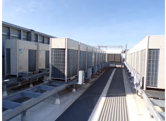
68. Twenty-seven Daikin rooftop VRV heat recovery compressor units are installed.
