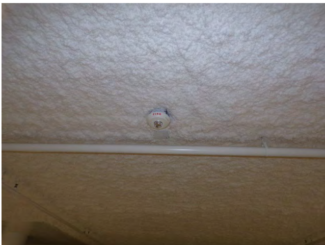
59. Basement: Interior finishes and fixtures. Horn/strobe alarm device shown.
