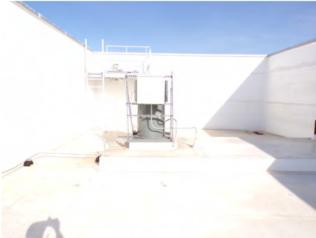
73. The second Loren Cook garage exhaust fan is located on the roof near the north stairwell.
