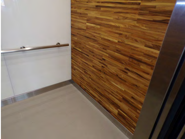
61. Interior finishes in elevator cars.
