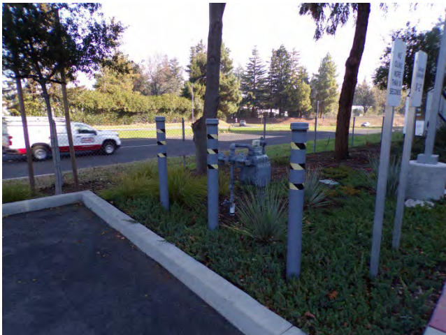
83. An automatic seismic shut-off valve is not installed on the gas service line.
