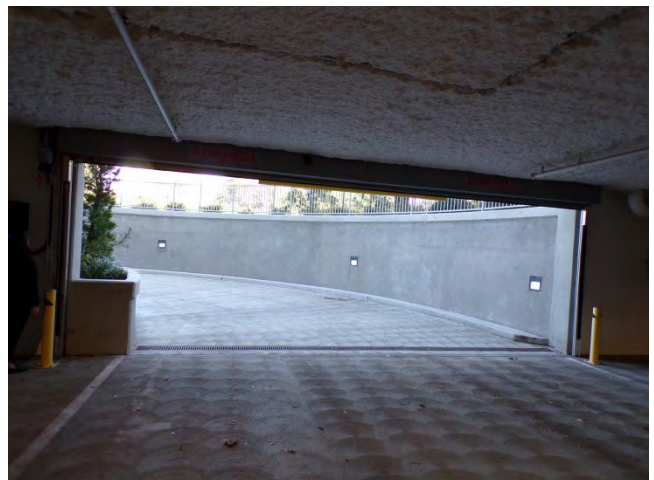
60. The overhead coiling door at the garage entrance was stuck in the raised position at the time of our site visit.
