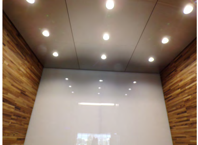
62. Interior finishes and fixtures in elevator cars.
