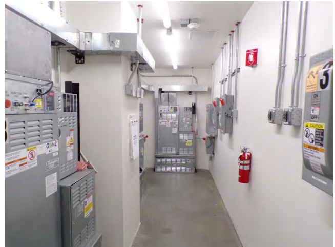
82. The elevator control room is accessed from the electrical service room.
