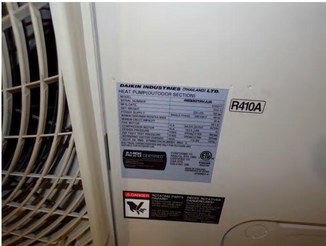
75. Three Daikin heat pumps are installed in the basement and provide dedicated conditioned air to the restrooms, lobby, and electrical room.
