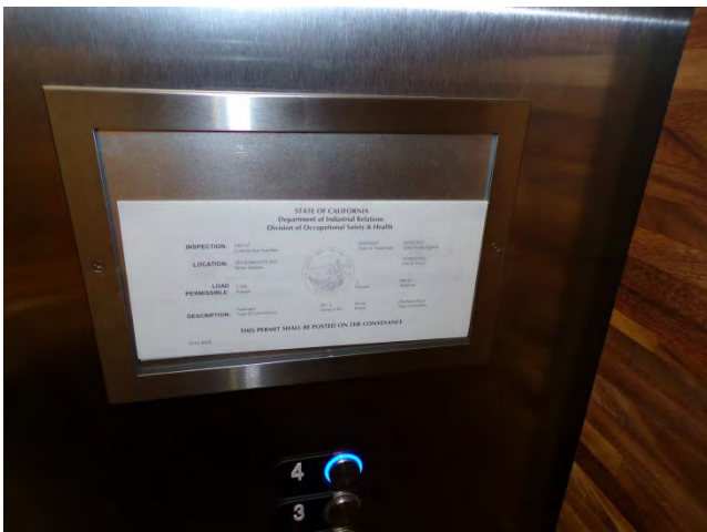
65. All elevator permits expired on March 3, 2022.
