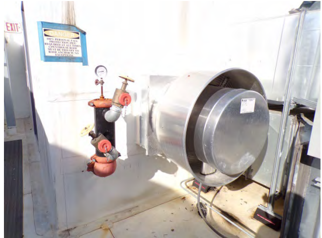
74. A larger Greenheck exhaust fan serves the restrooms. Rooftop FDCs at left.
