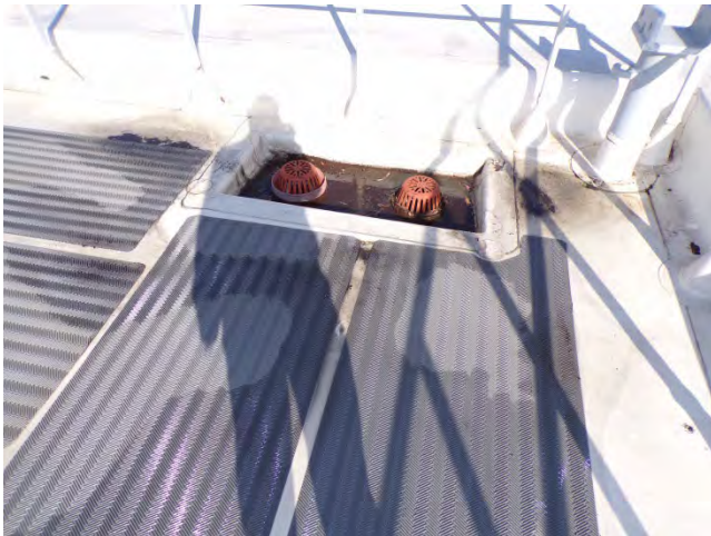
33. Near three drain combinations, the roof has a spongy feel when walking on it.
