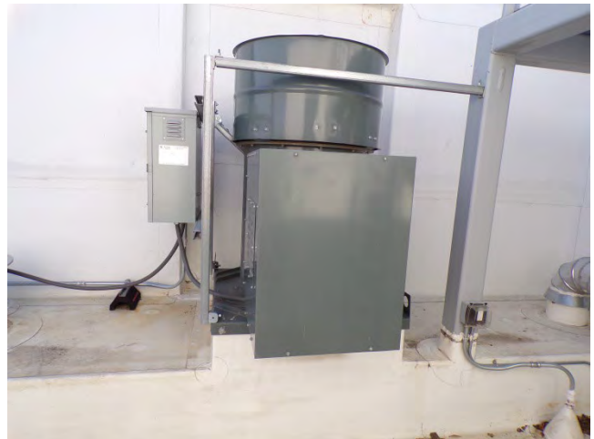
70. Two Loren Cook garage ventilation fans are roof-mounted; this one is near the stairwell penthouse.
