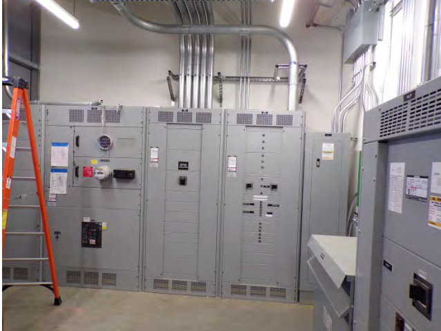
79. Infrared scanning of the electrical distribution equipment should be conducted once the building has achieved full occupancy for six months.
