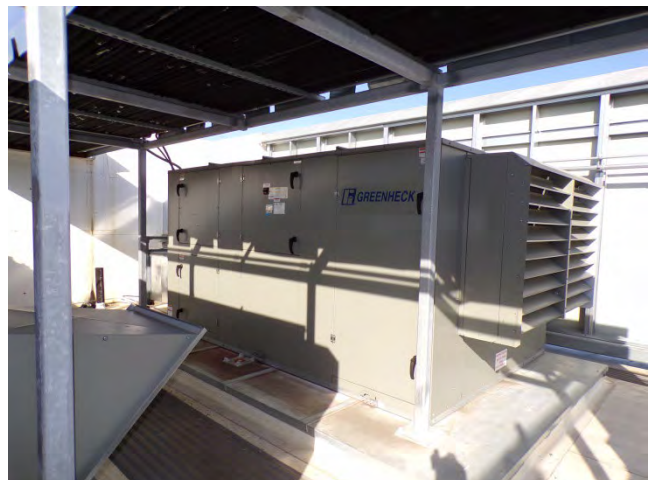
72. Two Greenheck ERVs are mounted on the roof and provide pre-conditioned air.
