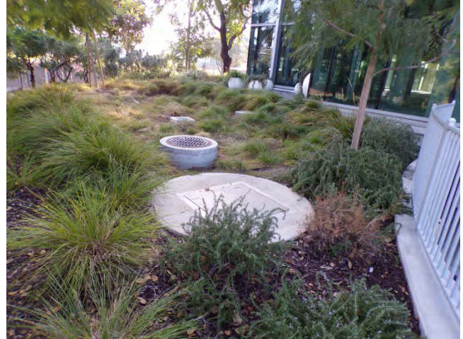
14. The vault for the storm water pump (foreground) is near the northeast corner of the building.
