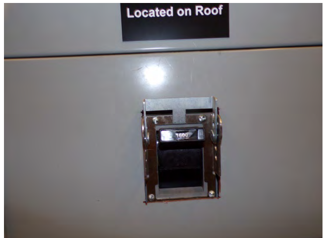
78. A 1,600 amp sub-main serves the rooftop HVAC equipment.
