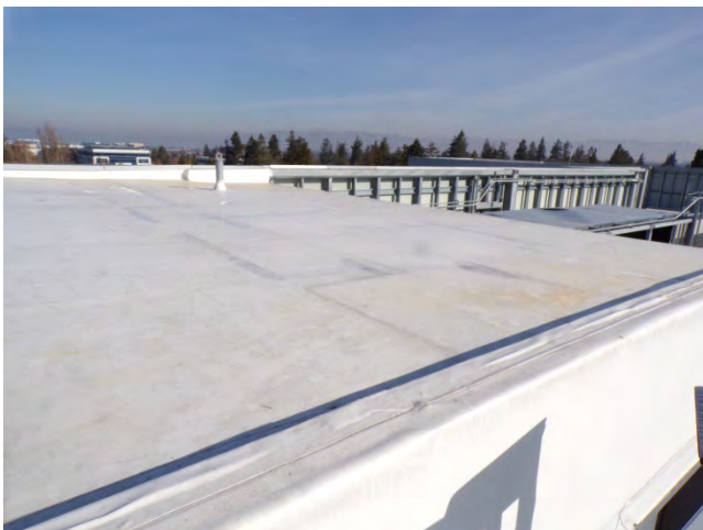
35. A TPO roofing system is also installed on the penthouse.
