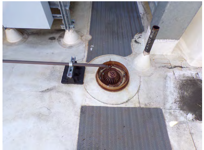
34. A grated drain without an overflow drain is provided for HVAC system condensate.
