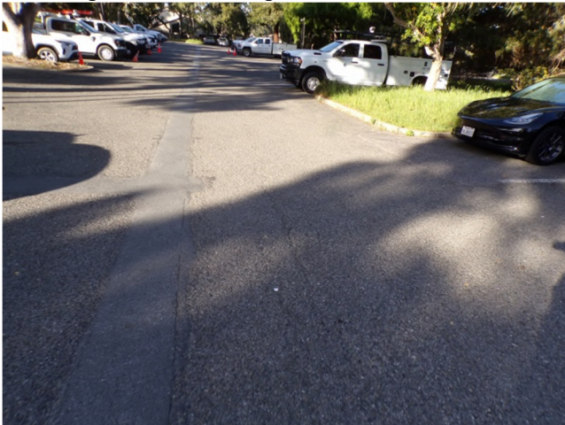
15. Degraded condition of asphalt paving—past repairs shown.
