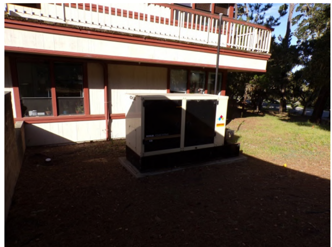
88. The emergency generator was installed and is maintained by California American Water. It provides electricity to their tenant space only.
