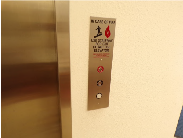
79. Required jamb-mounted floor designation signage is absent on both floors at elevator doors.
