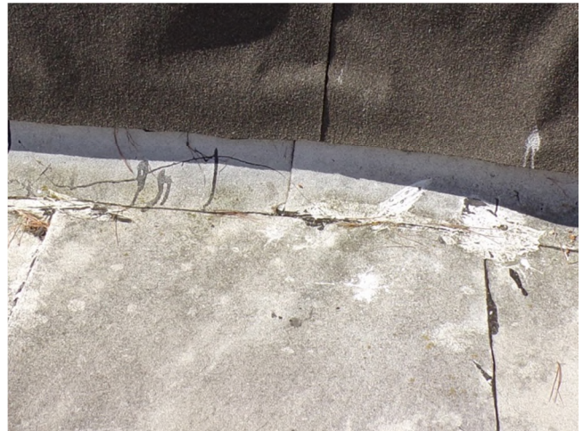
28. Both wings: We recommend that a TPO roofing system replace the existing BUR system. East wing shown.
