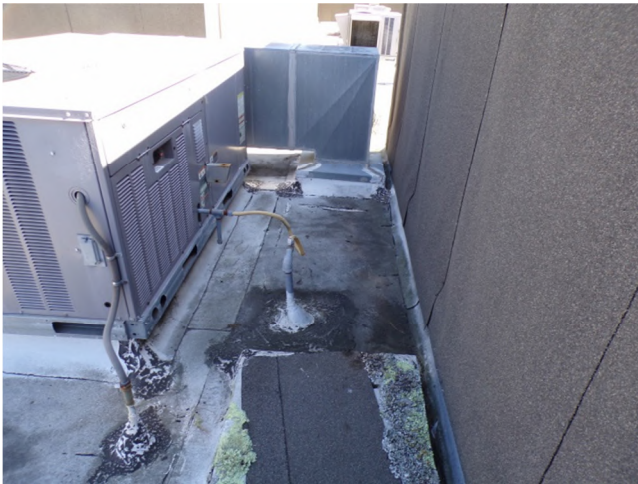
27. Both wings: The BUR system is in a generally run-down condition. East wing shown.
