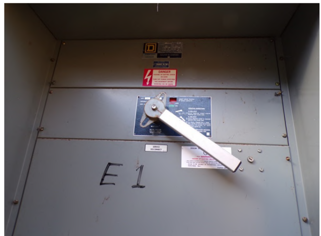
66. The main service equipment and the main disconnect are both rated at 1,200 amps.
