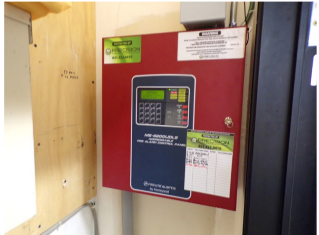
76. The FACP is no longer made and supported by the manufacturer.
