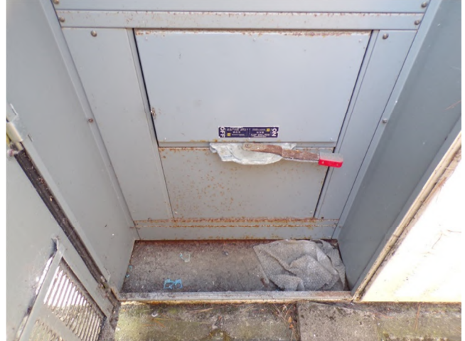
68. Rust was observed in all exterior electrical enclosures.
