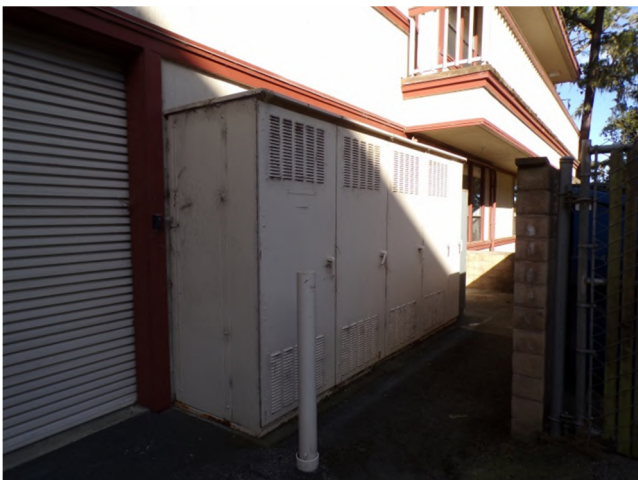
65. The main electrical service entrance equipment is located in an exterior location on the east side of the building.
