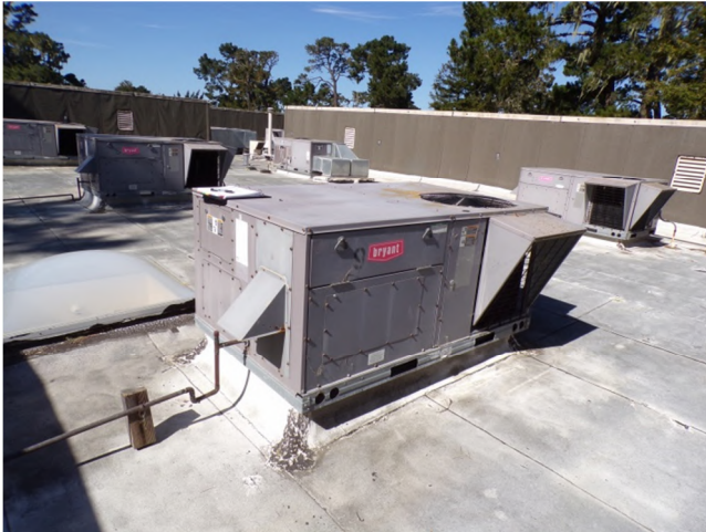
61. Twelve packaged units are installed. AC 9 shown. All twelve are generally similar in physical appearance.
