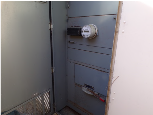
69. One electric meter is installed.
