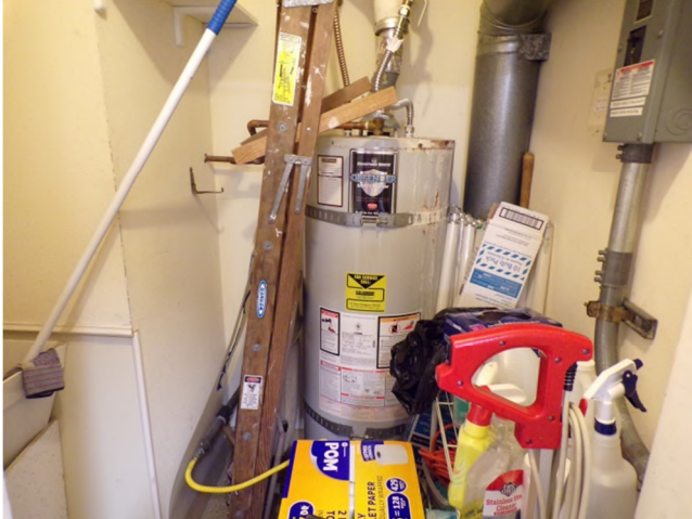
73. A 40 gallon gas-fired water heater is installed in the second floor janitor's closet.
