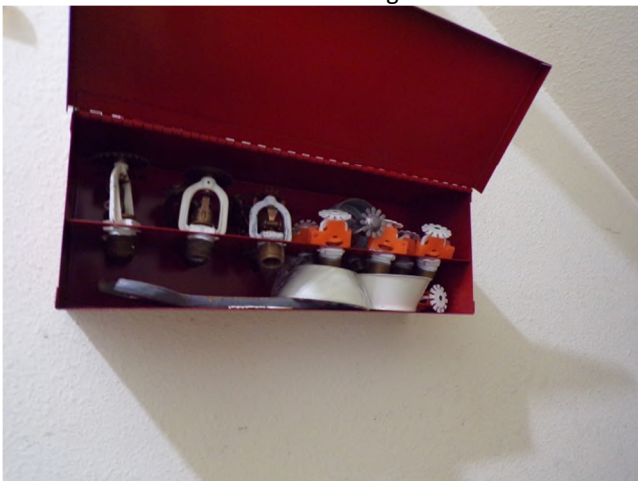
77. The spare sprinkler heads are found in the first floor janitor's closet.
