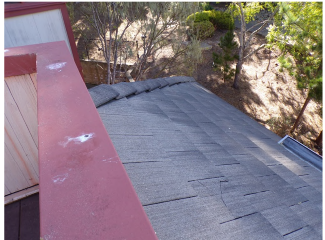
40. Cracked tiles on the pitched roofs were observed in various locations. Broken tile shown at right-center in foreground.
