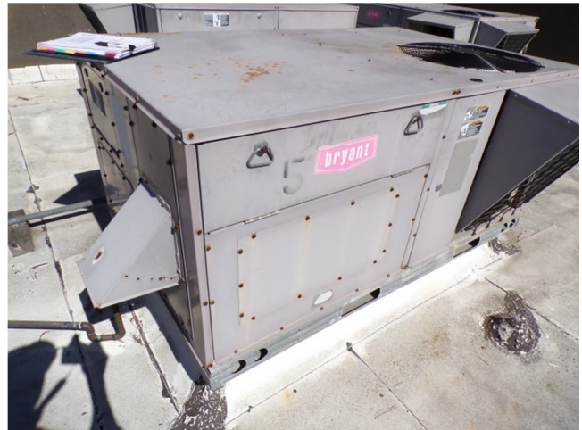
64. The provided cooling capacities (43 tons) appears inadequate for current tenant needs. AC 5 shown.
