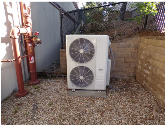
87. The CAC/BDP mini split-system was installed and is maintained by California American Water. It provides conditioned air to their server room only.
