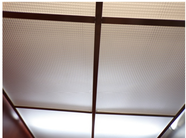
82. Ceiling diffuser grid in elevator cab.
