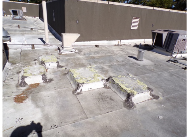
26. Both wings: The BUR system is in a generally run-down condition. East wing shown.
