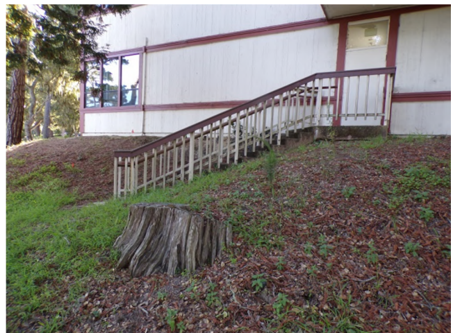
102. The railings of the north exterior stairs are non-compliant with current codes.
