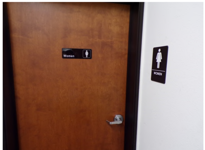
60. Accessibility signage with Braille (at right) is installed at restroom entrances.
