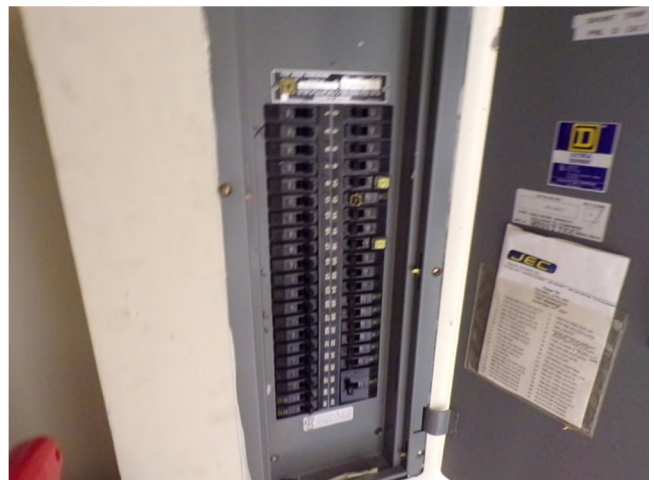
72. Branch sub-panels are found in interior locations.
