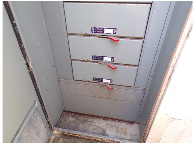
70. Each sub-main breaker is typically rated at 200 amps.
