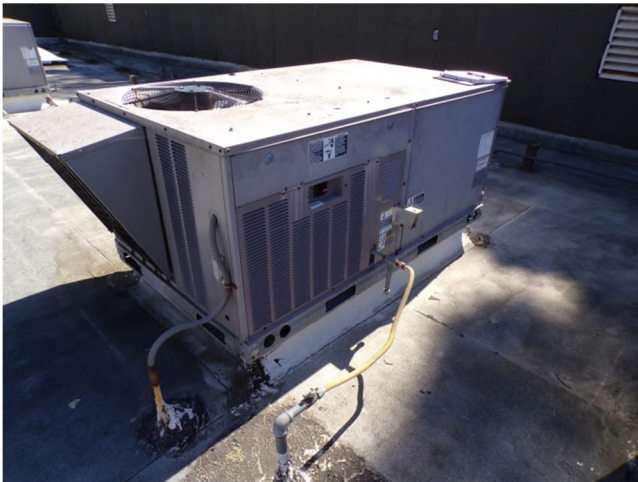
63. The furnaces all have flexible gas line connections. AC 7 shown.
