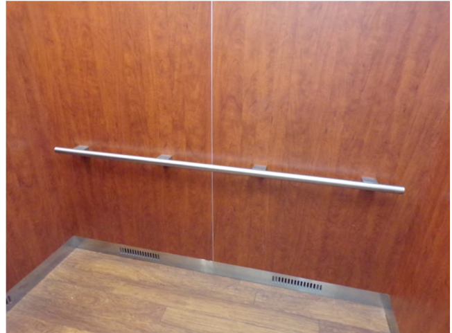
80. Interior finishes and stainless steel handrail in elevator cab.
