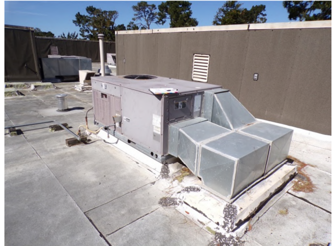
62. All packaged units were manufactured by Bryant in 2007. AC 2 shown.
