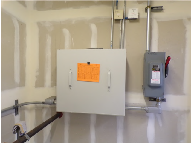
85. Elevator controller panel.
