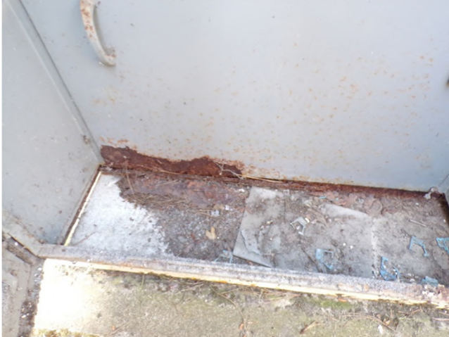
67. Rust-through at bottom of main disconnect enclosure.
