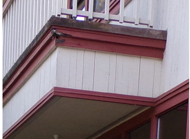
92. Rotten wood was observed in several exterior locations.
