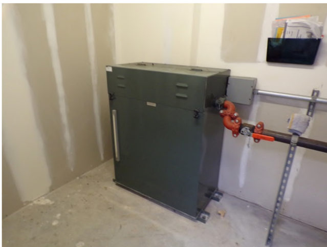
83. Hydraulic pump for elevator.
