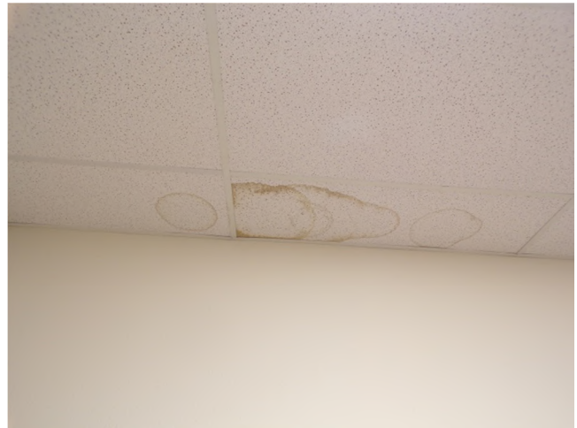
52. A small number of water stained ceiling tiles was observed in the second floor office areas we accessed.
