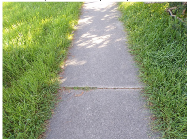
90. Changes in elevation in excess of ¼ inch in concrete panels create tripping hazards.
