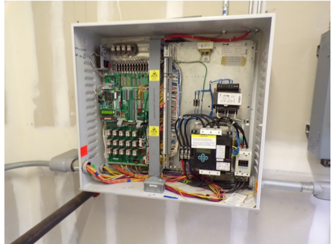
86. The elevator controller was modernized in 2007. A fully digital unit was installed.
