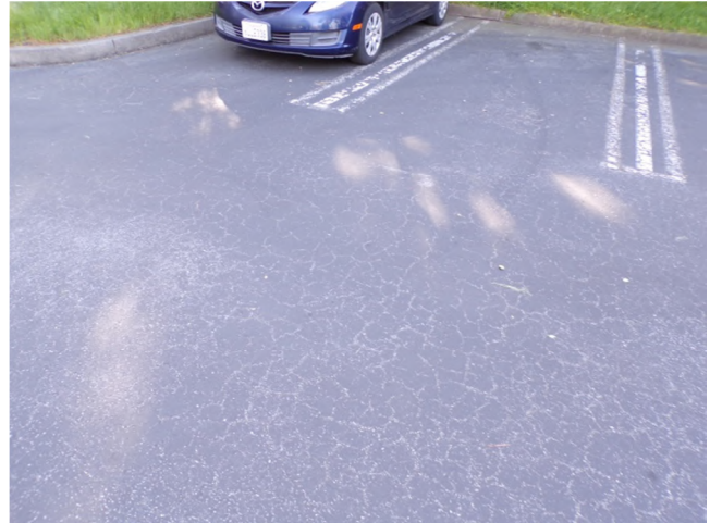
14. Degraded condition of asphalt paving—alligator cracking shown.
