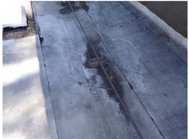
34. Both wings: Areas of past ponding are prevalent. East wing shown.
