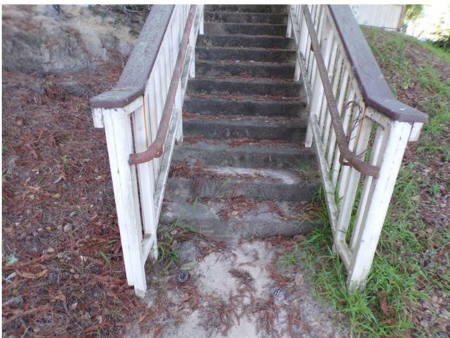
101. The north exterior stairs lack visually contrasting stripes on each tread, as required.
