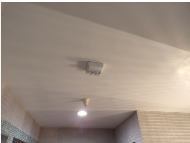
59. Horn/strobe alarm devices are installed in all restrooms.
