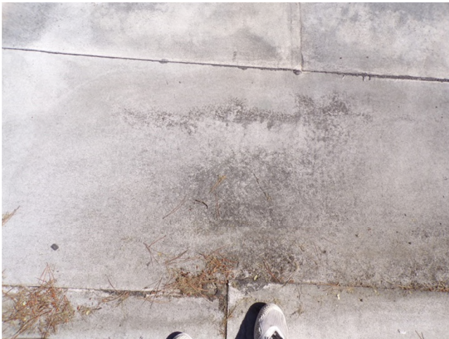
33. Both wings: Small accumulations of separated mineral granules were observed in several locations. West wing shown.
