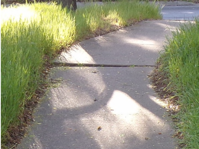
91. More egregious tripping hazards are also present.
