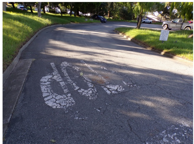
18. Degraded condition of asphalt paving—general surface and pavement marking degradation shown.
