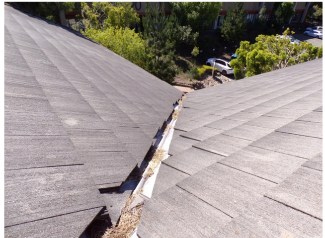
36. A concrete tile roofing system is installed on the pitched roofs. Broken tile in left foreground.
