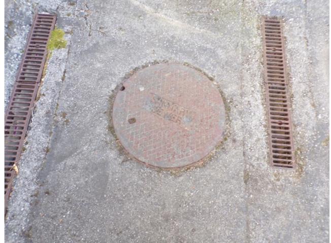
98. We recommend that a video snake sewer line inspection be conducted.
