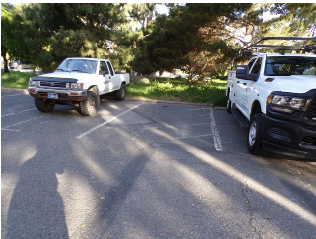
17. Restriping of all parking stalls will be required during the reserve term in conjunction with asphalt repairs.
