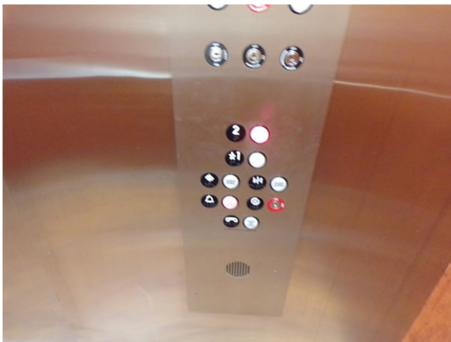
81. Elevator control panel in cab.
