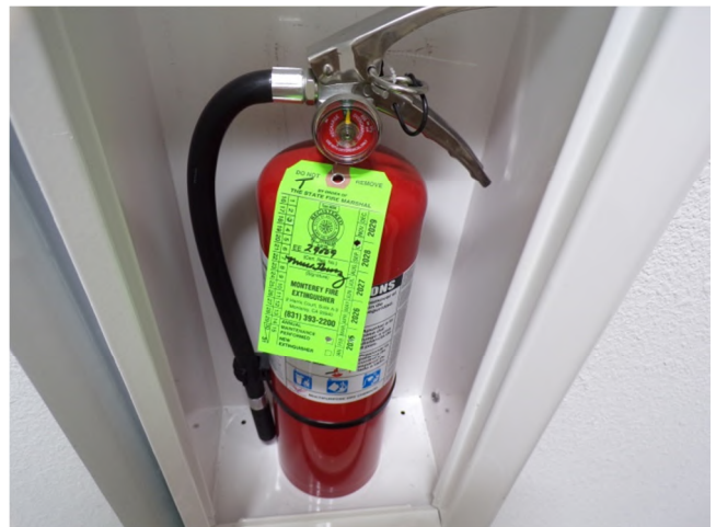
78. All observed fire extinguishers had valid inspection tags.
