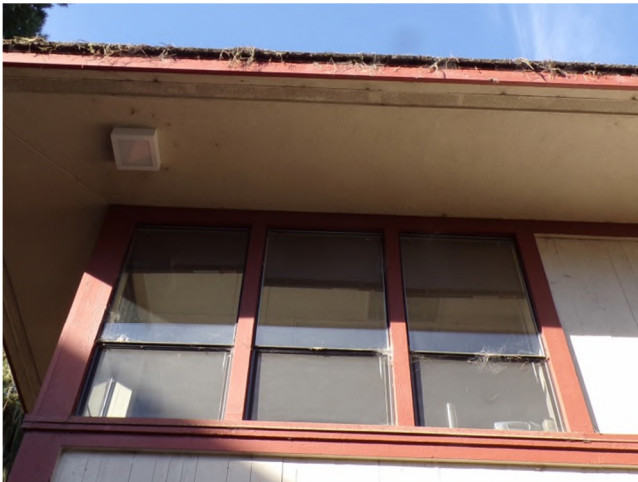
93. We are included an annual contingency allowance in the Spreadsheet for window rubber seal maintenance.
