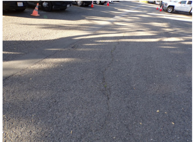
16. Degraded condition of asphalt paving—meandering cracking shown.
