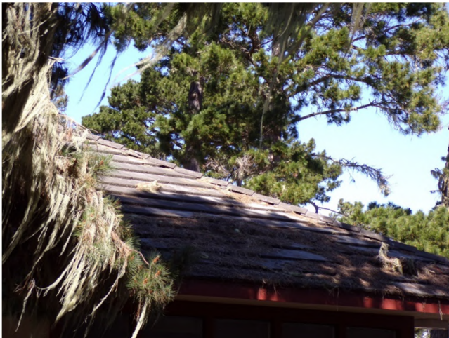
39. Accumulations of dead vegetation on the tile roof at southeast corner of east wing.
