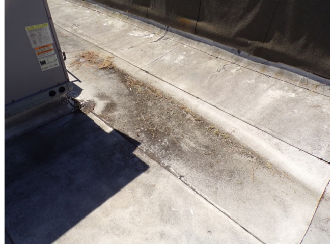
32. Both wings: Areas of past ponding are prevalent. West wing shown.
