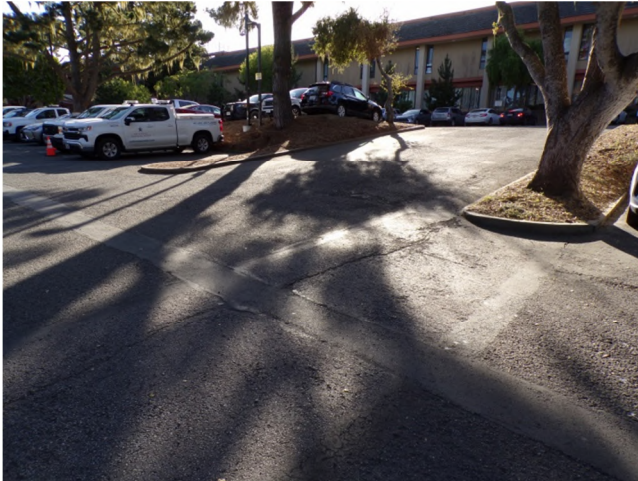
13. Degraded condition of asphalt paving—past repairs and general surface degradation shown.
