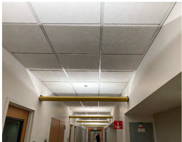
M-12. Corridor light fixtures.
