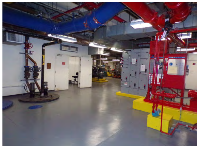
42. Interior finishes and fixtures in main mechanical room.
