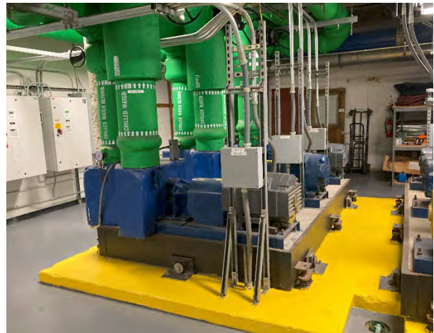
M-4. Chilled water circulating pumps.
