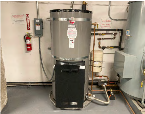
M-15. Domestic water heater.
