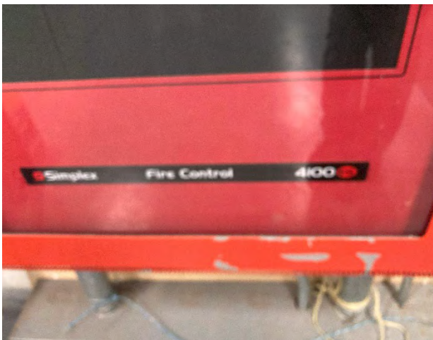
M-17. Fire alarm panel.
