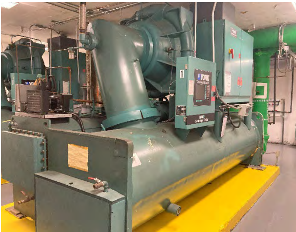
M-3. Water cooled chiller.
