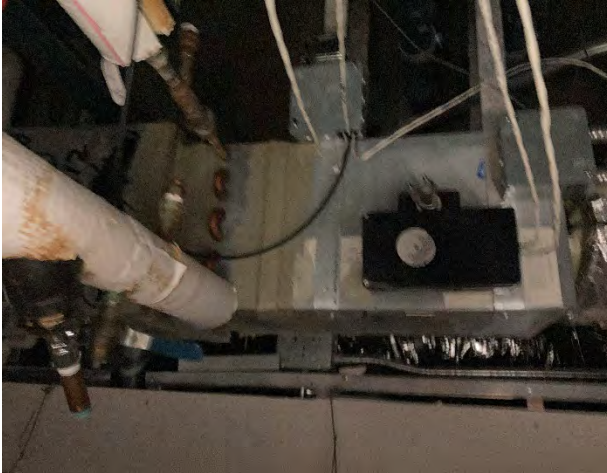
M-1. VAV box with hot water reheat coil.
