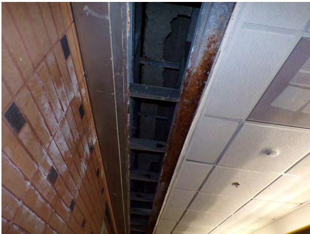
51. Water intrusion damage in first floor foyer near main mechanical room. Efflorescence also shown on brick wall.
