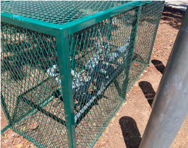
M-13. Natural gas service.
