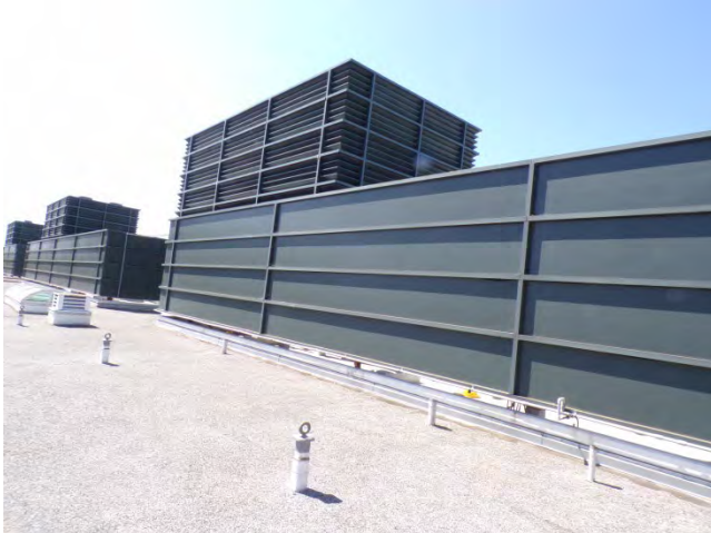
25. The mechanical equipment screens are steel-framed with painted fiberboard facings.
