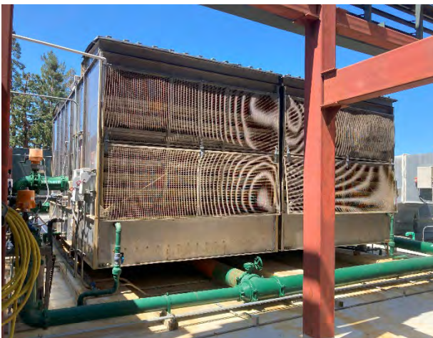
M-5. Cooling tower.
