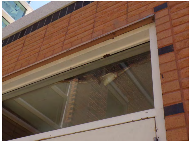
52. Water intrusion damage in first floor foyer near main mechanical room, as seen from exterior.
