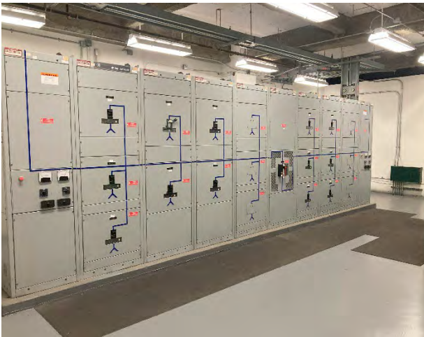
M-9. Main electrical switchgear.
