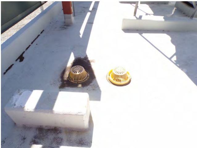
27. Within the screened areas, the roof and overflow drain combinations are not installed in shallow sumps.
