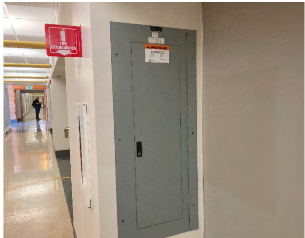
M-10. Electrical distribution sub-panel.
