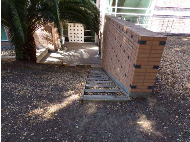
13. Two sets of timber stairs are located along the north elevation. The stairs are not compliant with current codes. Concrete/brick veneer retaining wall also shown.
