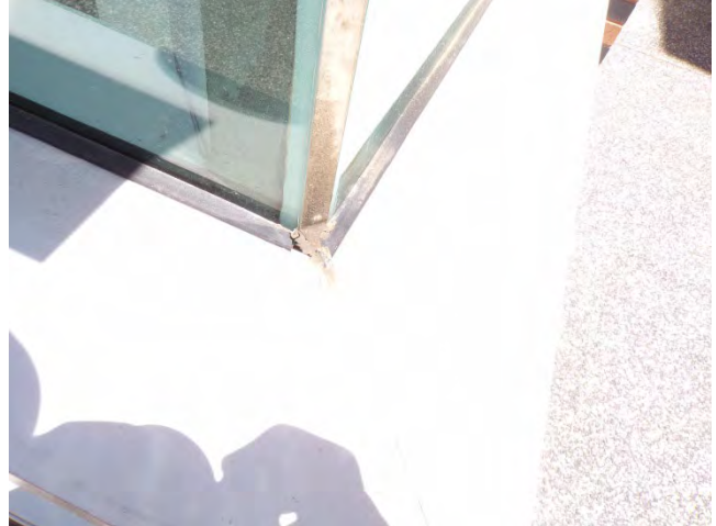
50. Shrunken rubber window seal with gap between seals shown.
