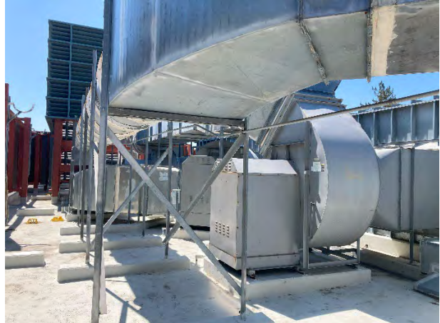
M-8. Laboratory exhaust fans.
