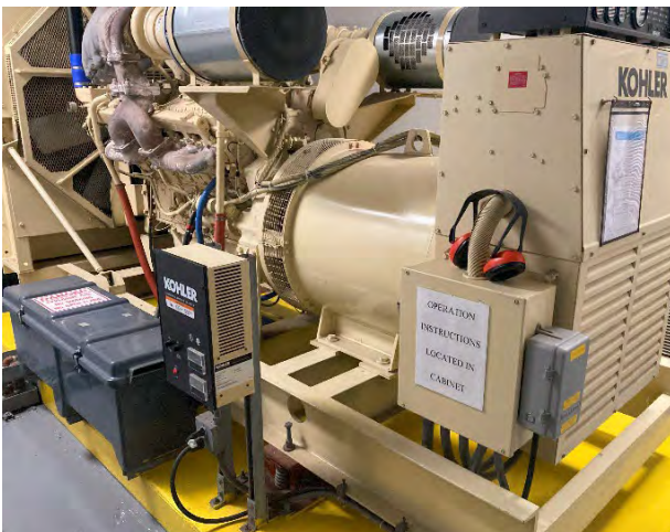
M-11. Emergency generator.
