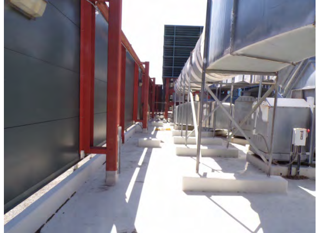
26. The gravel ballast is not applied within the equipment screened areas of the roof.
