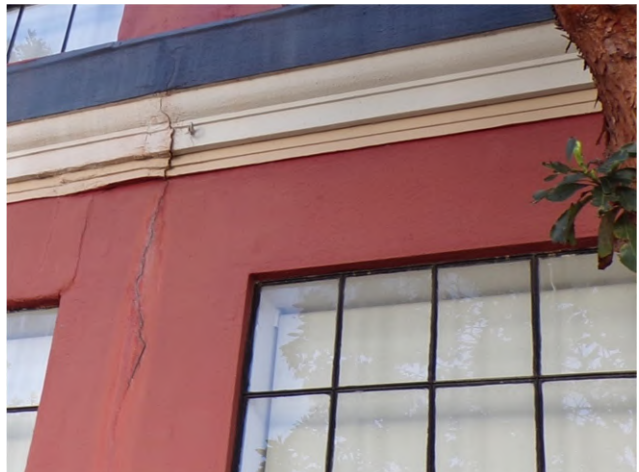
102. Degraded condition of exterior finishes with cracks shown.
