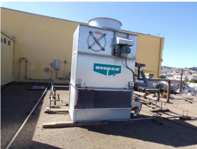
35. The Evapco cooling tower provides chilled water to the hydronic loop system.
