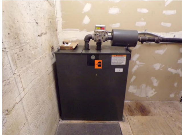
62. Hydraulic pump for elevator. The elevator and its hydraulic equipment date to 1998.
