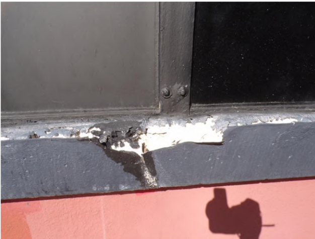
105. Degraded condition of exterior finishes with degraded paint and spalled concrete ledge shown.
