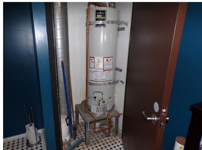
52. The natural gas-fired water heater is located in a service closet in a fourth floor restroom.
