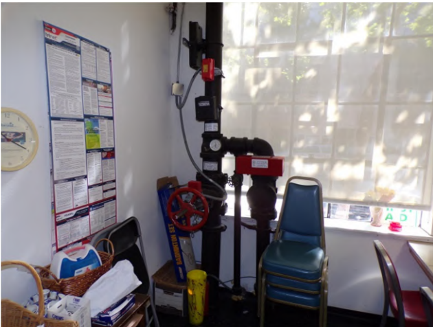
57. Five-year and annual NFPA fire sprinkler system inspections should be conducted, as required.
