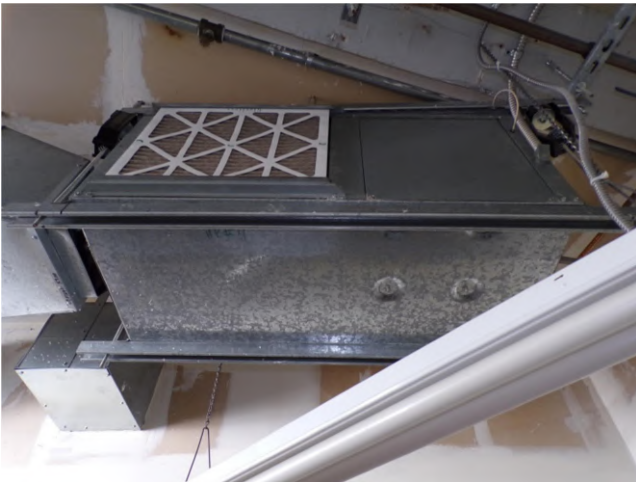
45. Seven water source heat pumps are installed in attic locations on the first and second floors.
