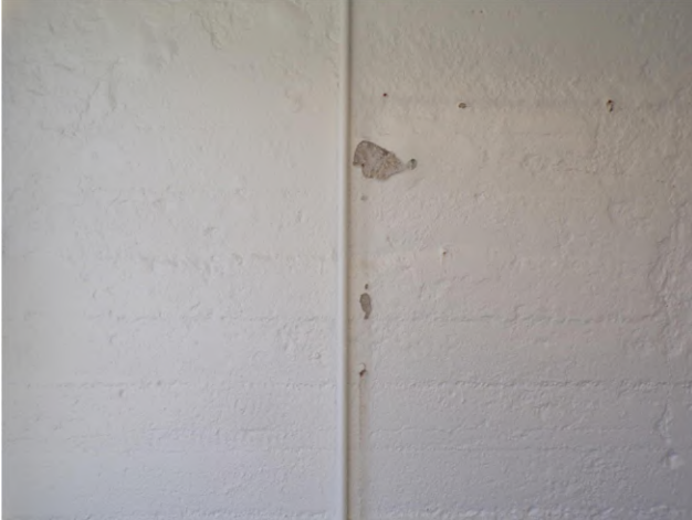
97. On the fourth floor, there is interior side evidence of water penetration through the perimeter concrete walls. Treatment with Xypex is recommended.
