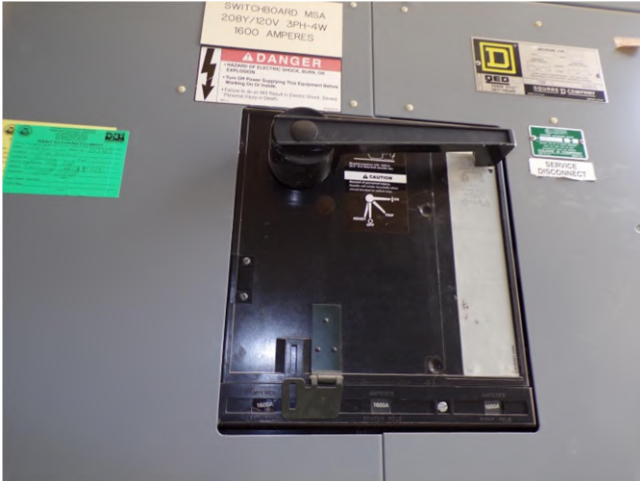
49. The 1,600 amp main disconnect.
