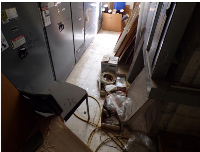
51. Items stored near or leaning on main electrical service equipment should be removed.
