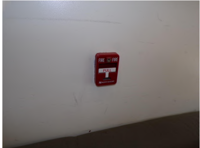
56. One manual pull station was observed.
