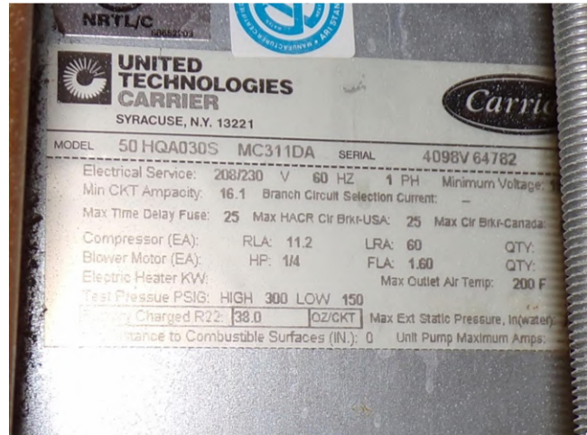
46. The six Carrier heat pumps were manufactured in 1998.
