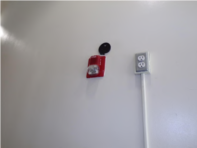
55. Fire alarm devices, such as the horn/strobe shown, are not provided in all required locations.
