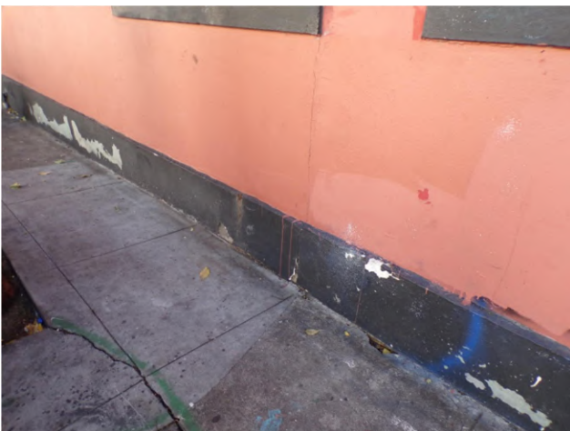
95. Concrete cracks and degraded condition of exterior paint finishes.
