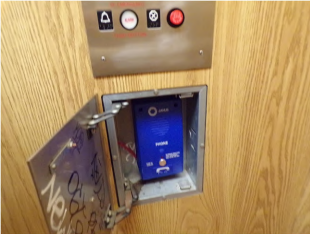
61. Hands-free communication device in elevator.
