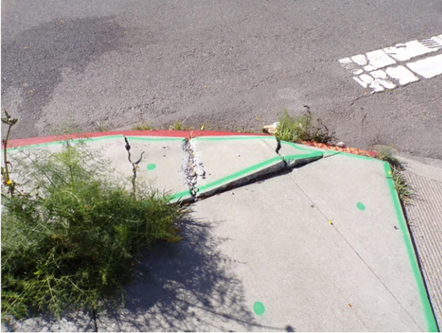
19. Tripping hazards were observed in several locations. Green paint denotes the tripping hazards. Southwest corner of site shown.
