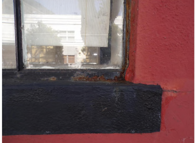
98. Rust is prevalent on the steel window frames.
