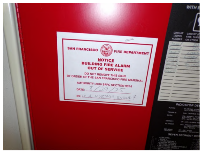
54. The fire alarm system is out of service owing to telephone line issues.
