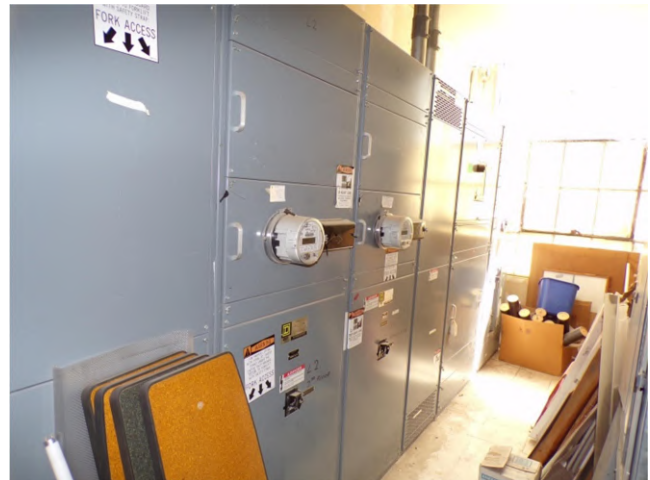
48. The 1,600 amp capacity main electrical service equipment was manufactured by Square D.
