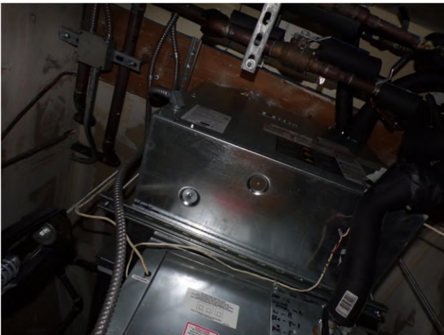
47. In 2022, a Bosch water source heat pump was installed atop an older Carrier unit.
