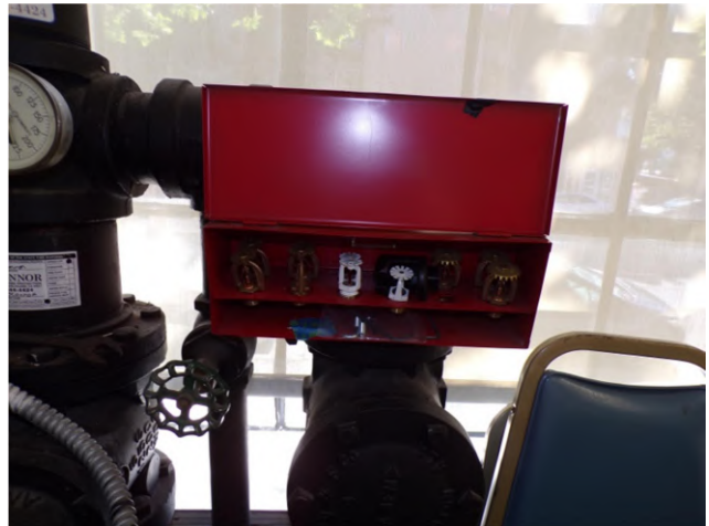
58. A box of spare sprinkler heads is provided.
