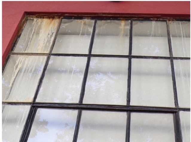
100. We recommend that the steel window frames be restored.
