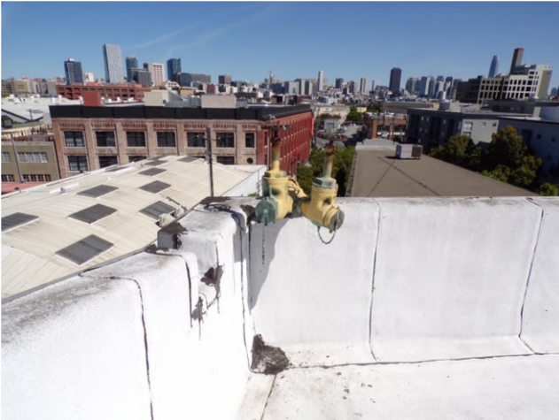
31. Fourth floor roof: Fire department connections. This roof level has taller parapets.
