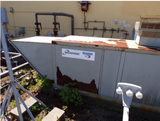
39. The age of the Modine make-up air unit is unknown. Replacement is recommended.
