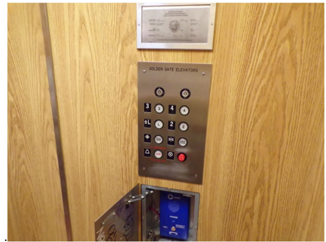
60. Elevator control panel in cab.
