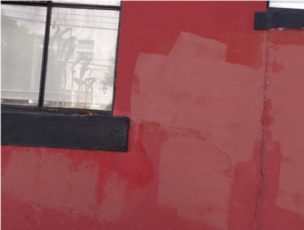
103. Degraded condition of exterior finishes with cracks shown.
