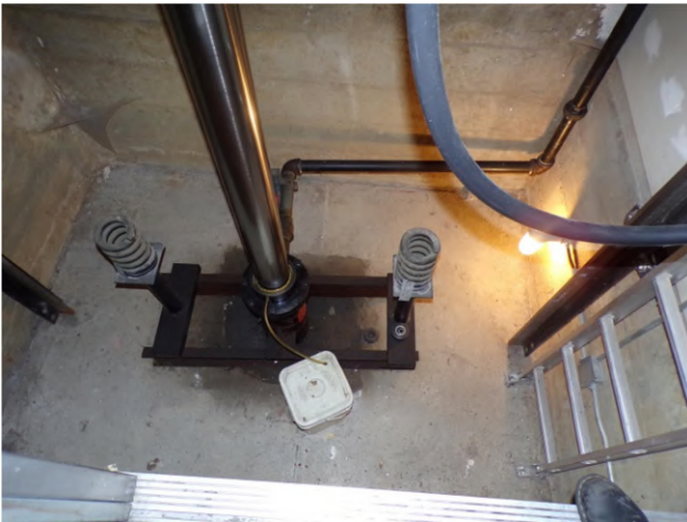
111. The elevator pit with hydraulic equipment.
