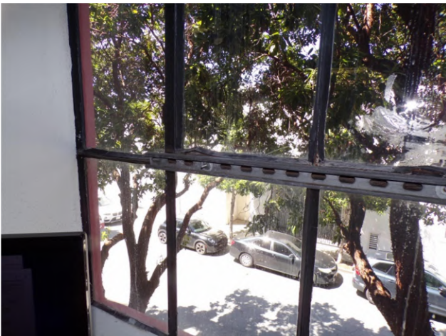
101. On the second floor, there is interior side evidence of water penetration through the windows. Buckled glazing compound shown.
