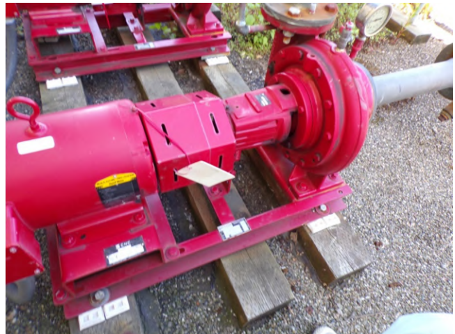
42. Two Bell & Gossett pumps serve the hydronic loop system.
