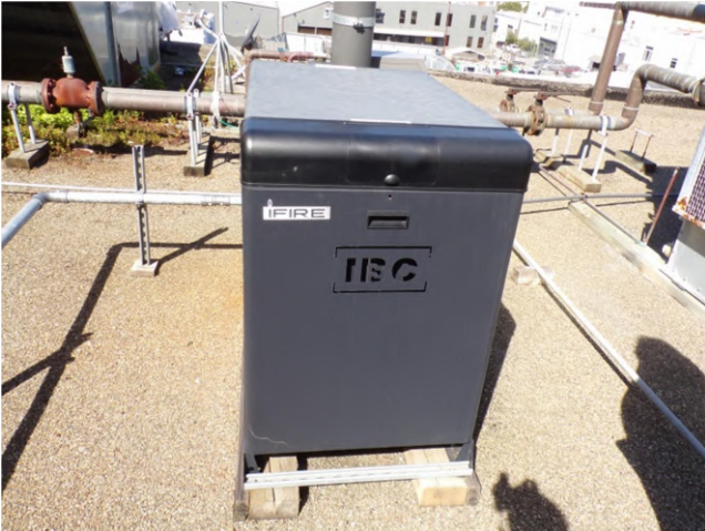
37. The IBC Technologies boiler provides hot water to the hydronic loop system.
