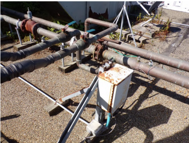
41. Rooftop piping for the hydronic loop system.
