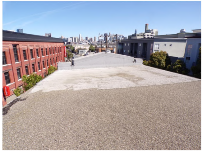
22. Main roof: At the far north end of the building, the pea gravel is not provided.
