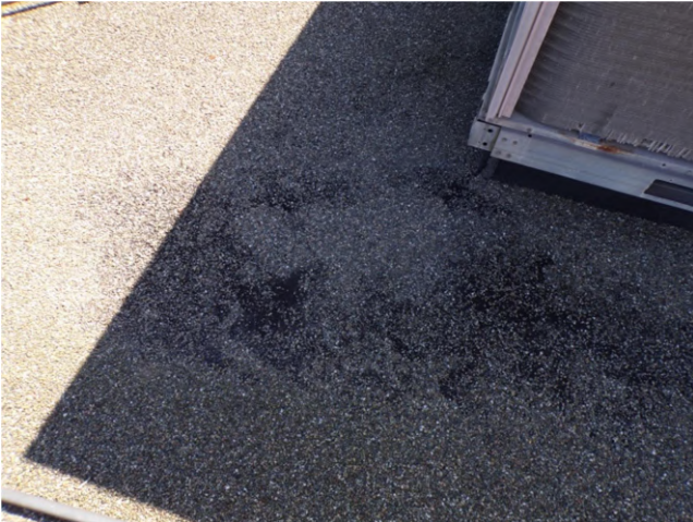
25. Main roof: The age of the roofing system is unknown; replacement is recommended.
