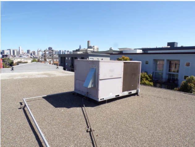
33. Two 12 ton Carrier packaged units are mounted on the main roof level.
