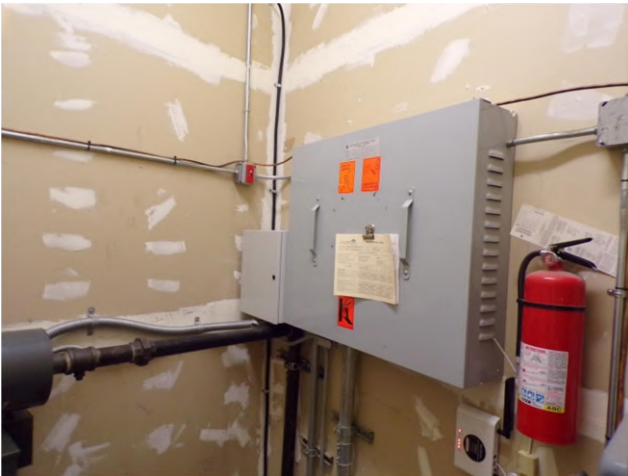
63. The digital control panel for elevator dates to 1998.
