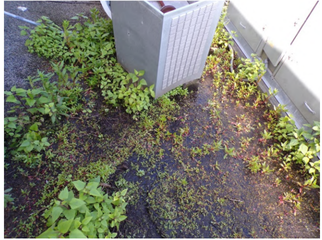
26. Main roof: An area of longstanding ponded water is present.
