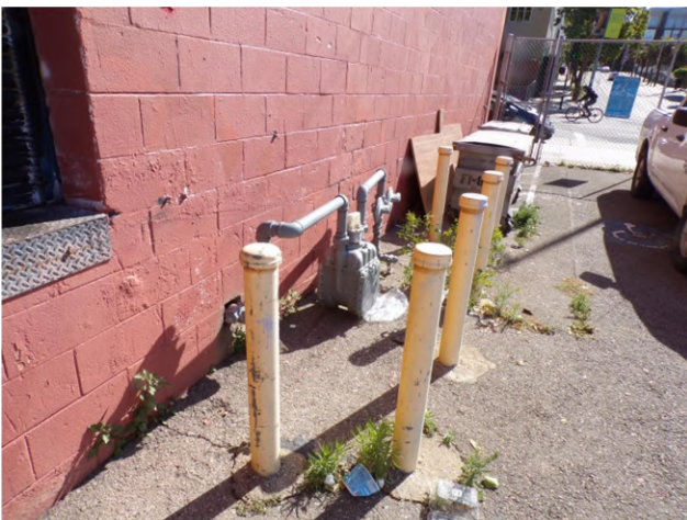
107. The gas service line is not fitted with an automatic seismic shutoff valve.
