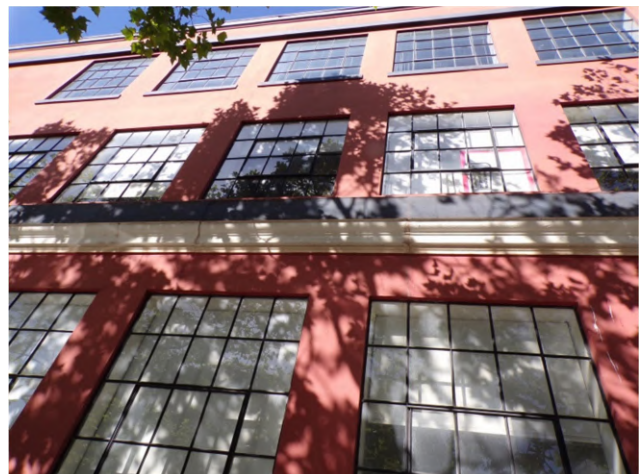
96. Concrete cracks and degraded condition of exterior paint finishes.
