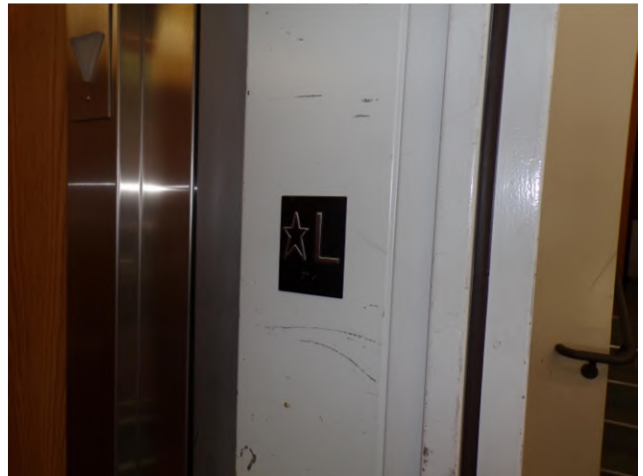
64. The installed door closure arrestors require physical contact. Replacement is recommended.
