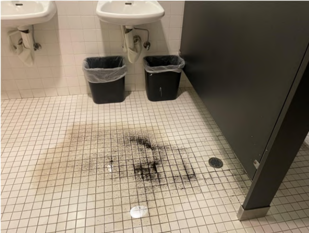
109. Earlier in the week of our site visit, minor flooding up through the floor drains occurred.
