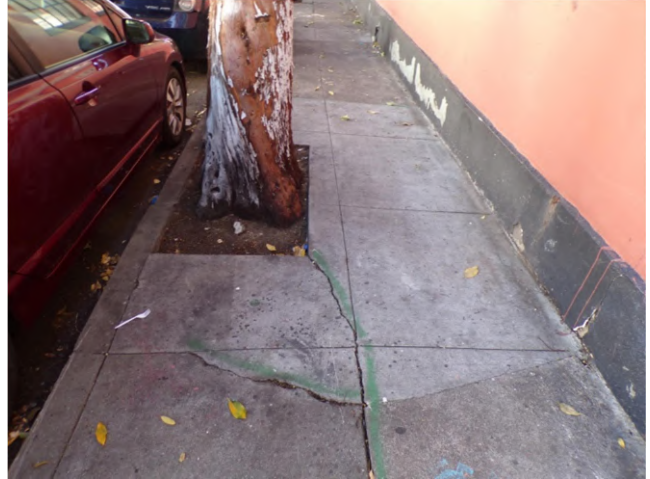
20. Tripping hazards were observed in several locations. Sidewalk along west elevation shown.
