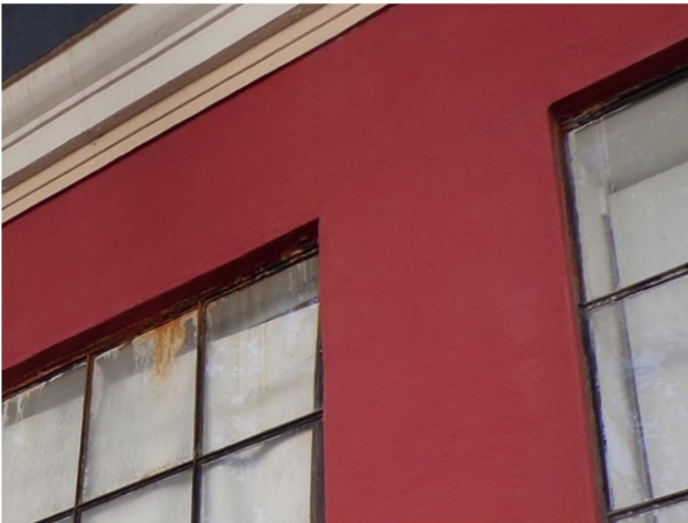
99. Rust is prevalent on the steel window frames.
