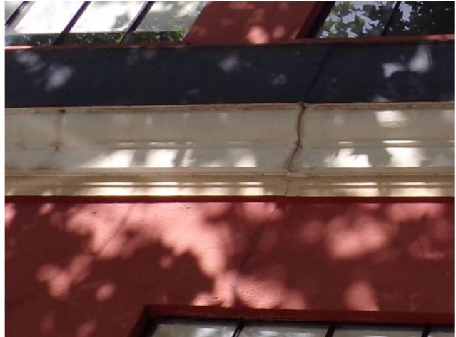
104. Degraded condition of exterior finishes with cracks shown.
