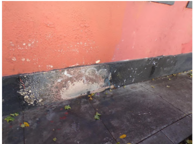
106. Degraded condition of exterior finishes with degraded paint shown.
