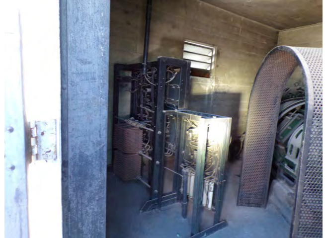
140. 5601E: The elevators have outdated relay-type controllers.
