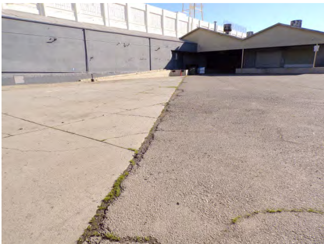
41. Bldg 5733W: Concrete paving at left; asphalt paving at right. Both types of paving are typically in a run-down condition throughout the property.
