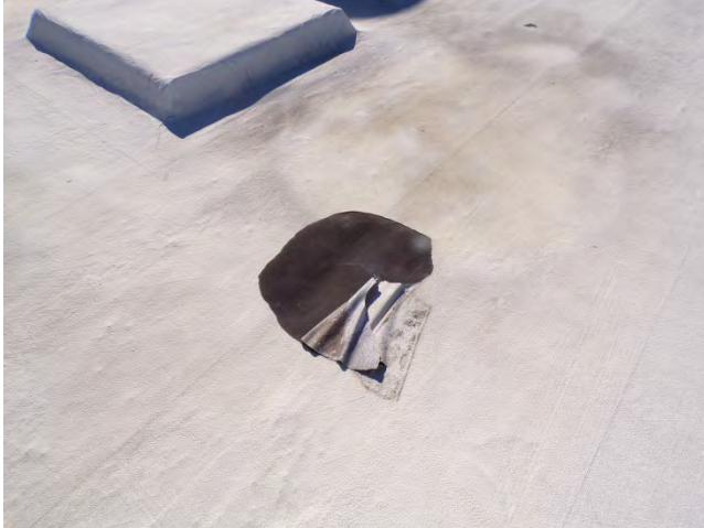
55. Bldg 5601E: The BUR roofing system is in an overall degraded condition.
