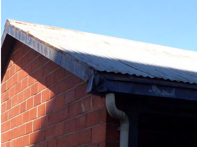
85. The ribbed steel panel roofing system on the carport is in a degraded condition; rust was observed in numerous locations.
