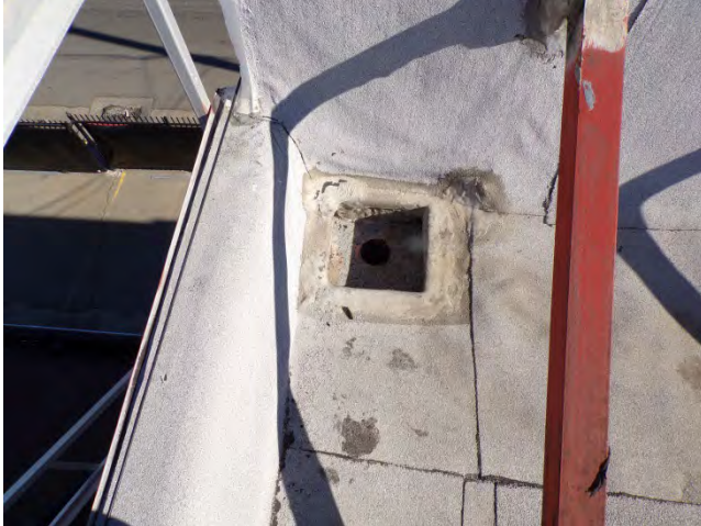
73. Some roof drains lack atrium grates or screens. Bldg 5733E shown.
