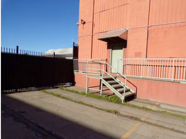
127. Various deficiencies were observed with exterior stairs. Damaged non-compliant railings shown.
