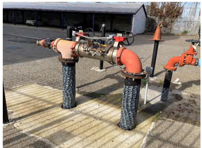
M-12. Bldg 5601: Fire sprinkler water service.
