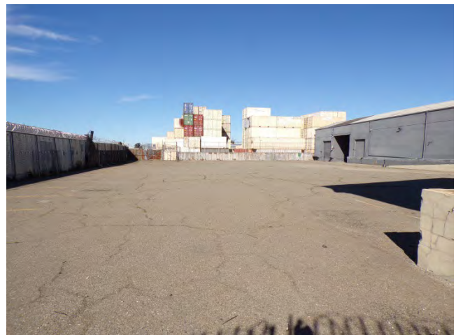
42. Bldg 5733W: Degraded asphalt paving requires repairs and resealing during the reserve term.
