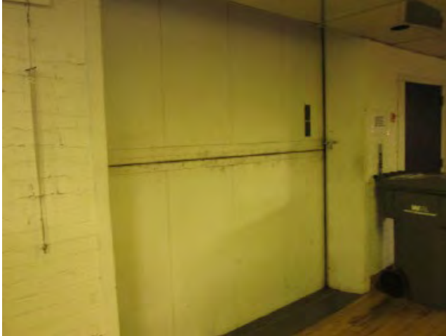
139. 5601E: Three freight elevators are installed in this building. (Photo from 2017 PCA.)
