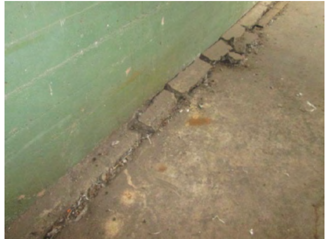
134. Various deficiencies were observed in loading areas. Degraded concrete shown. (Photo from 2017 PCA.)
