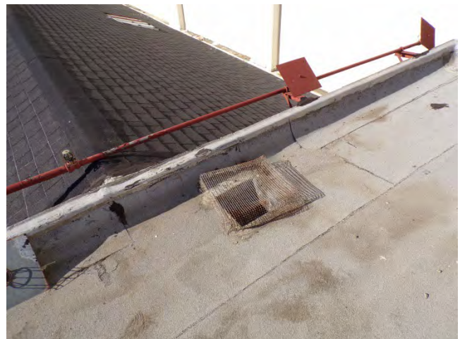
72. Bldg 5733E: Screened roof drains are installed; overflow protection is not provided.
