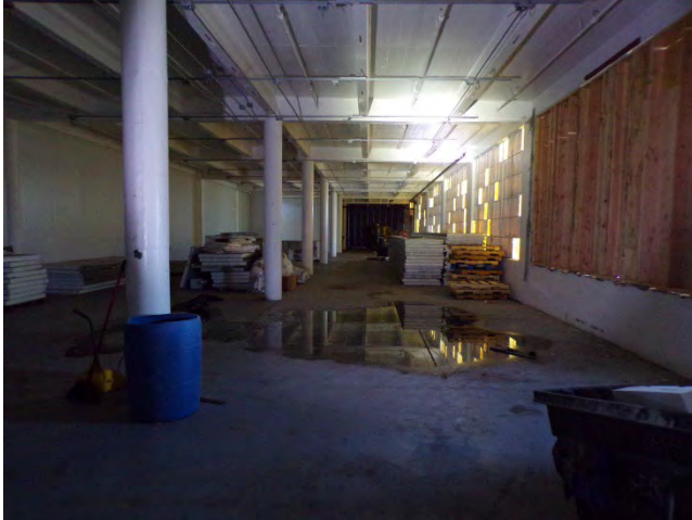
91. Bldg 5601E: Window opening at right is infilled with plywood. Water intrusion has occurred along the north elevation at third floor level.
