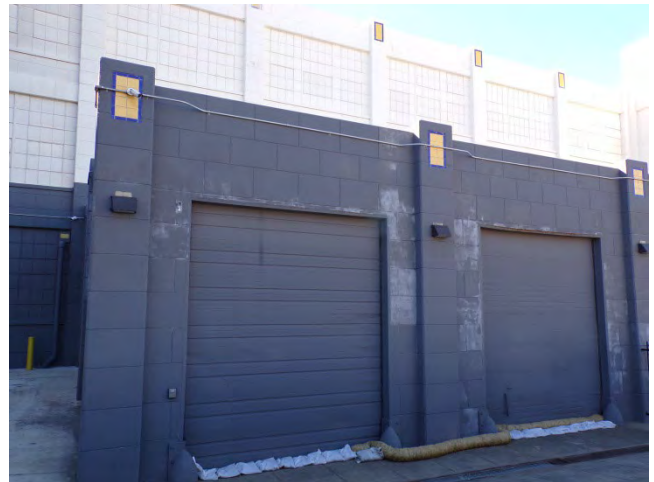
136. Steel framing at lintels is in a degraded condition; replacement is recommended.
