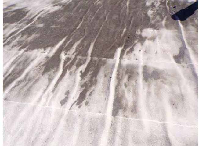
56. Bldg 5601E: The BUR roofing system is in an overall degraded condition.
