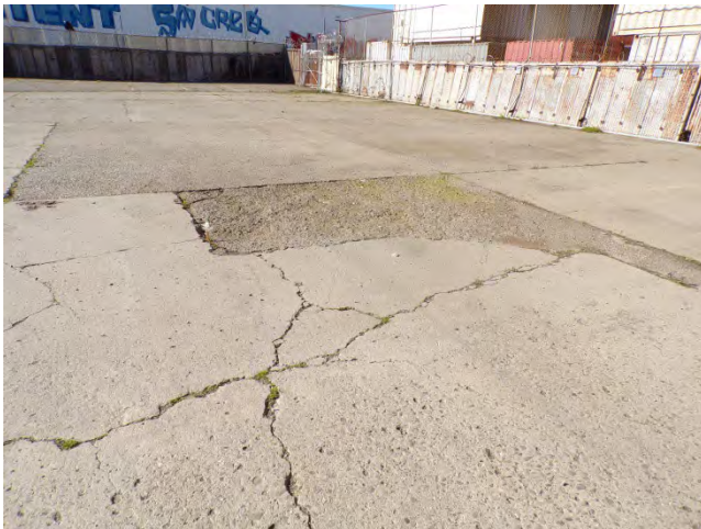
39. Bldg 5601W: Degraded condition of concrete parking area on north side of building.
