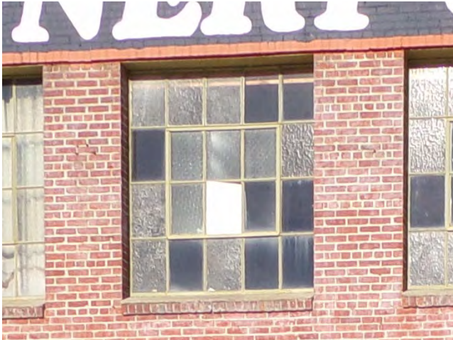
133. Various deficiencies were observed with exterior glazing. Glass pane replaced with cardboard shown.
