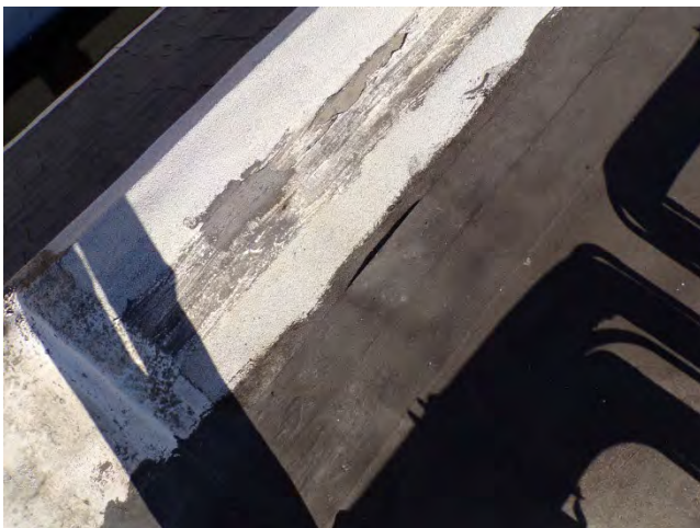
83. Bldg 5733W: The BUR roofing system is in an overall degraded condition. Split in roofing membrane at repair shown.
