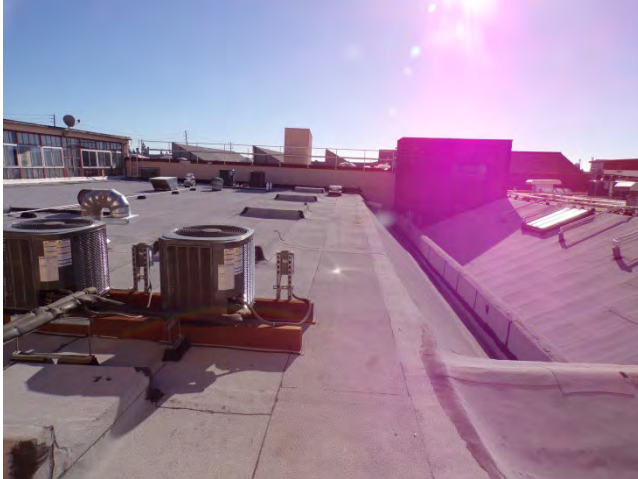
67. Bldg 5733E: The BUR roofing systems are in a generally run-down condition.
