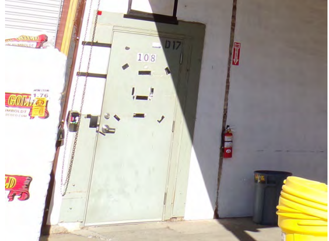
32. Bldg 5733W: Primary pedestrian entrance on south elevation. Door sill is not Accessibility compliant.
