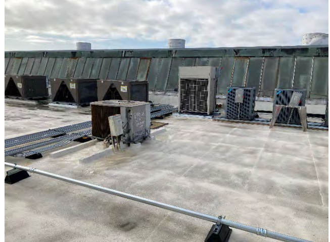
M-2. Bldg 5601E: Split system air conditioner.
