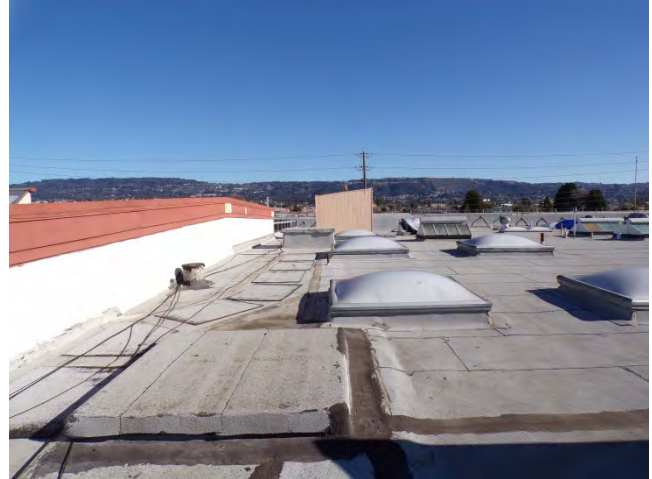
68. Bldg 5733E: The BUR roofing systems are in a generally run-down condition.
