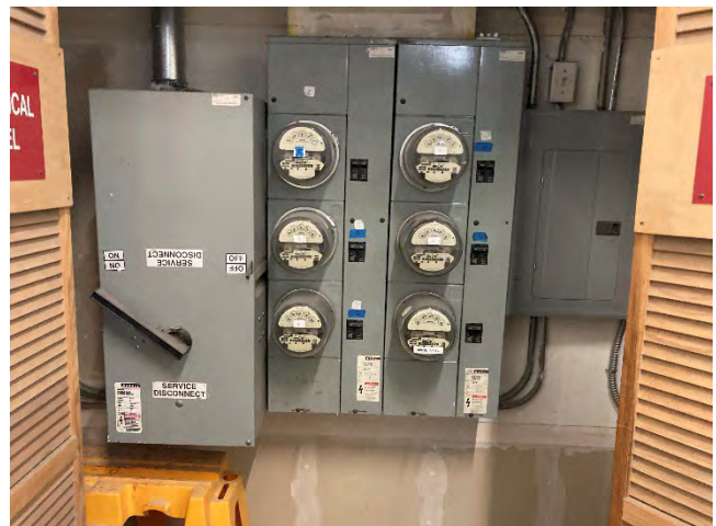
M-6. Bldg 5733E: Residential electric meter bank.
