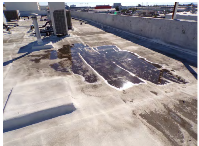
54. Bldg 5601E: Pooled water was observed in multiple locations.
