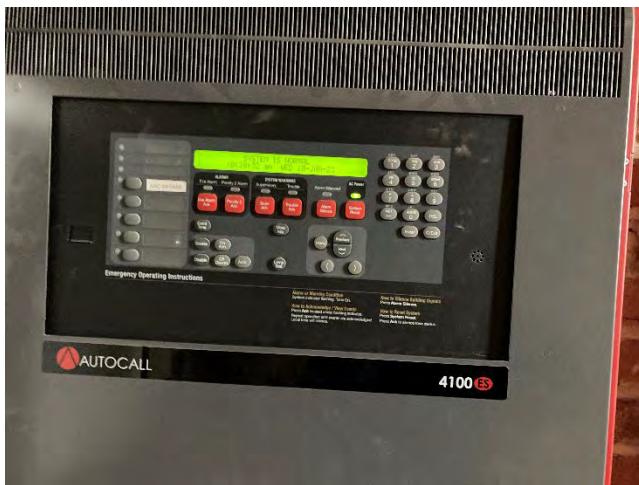
M-15. Bldg 5601E: Fire alarm panel.
