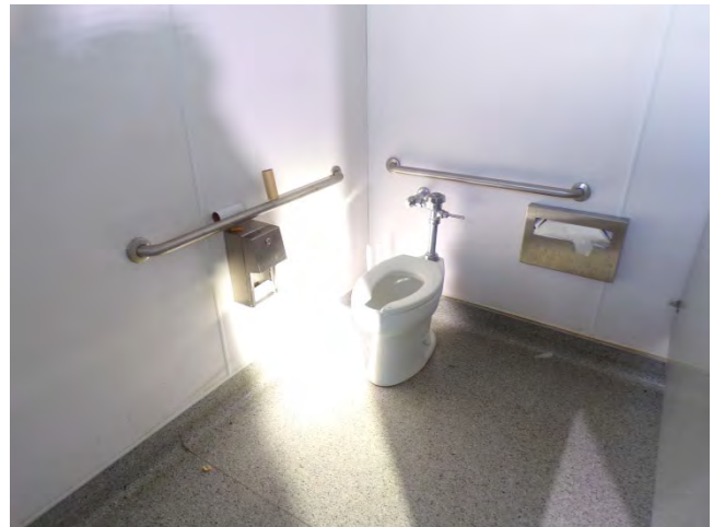
118. Bldg 5601E: Interior finishes and fixtures in restrooms.
