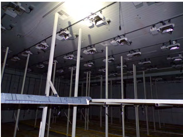
95. Bldg 5601W: Interior finishes, fixtures and equipment in plant cultivation rooms.
