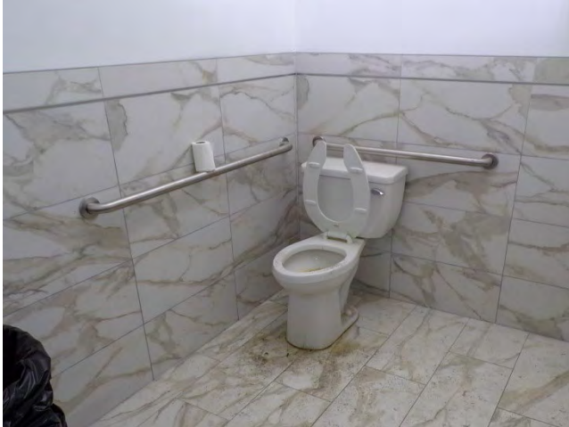
115. Bldg 5601E: Interior finishes and fixtures in restrooms.
