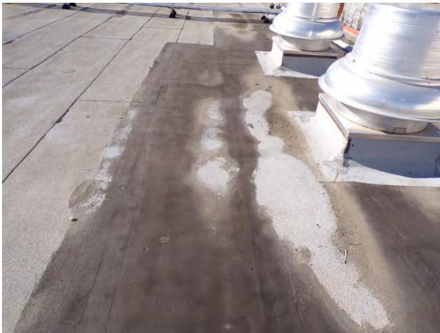
81. Bldg 5733W: The BUR roofing system is in an overall degraded condition. Separated mineral granules shown.
