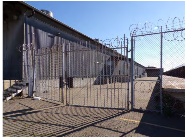
124. Deficiencies with fences and gates were observed. Most fencing at the property has an overall run-down appearance.
