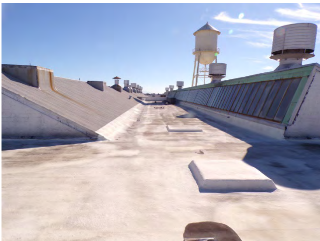
53. Bldg 5601E: The BUR roofing system is in an overall degraded condition.
