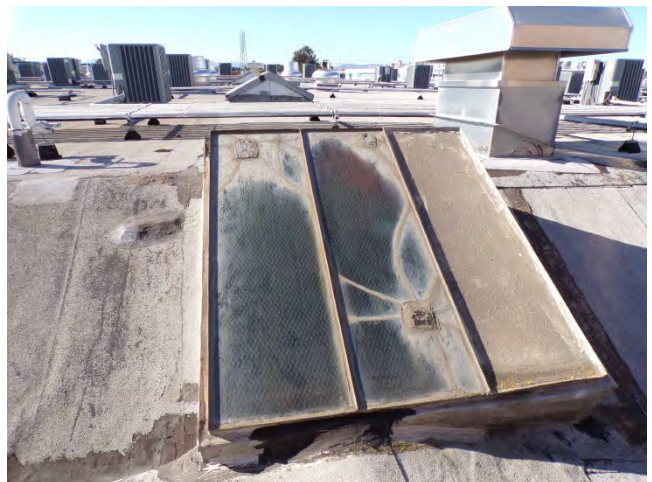
84. Bldg 5733W: Broken windows were observed in the skylights.
