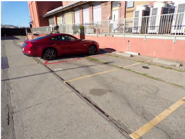
45. Bldg 5733E: The concrete-paved parking area is in a generally run-down condition.
