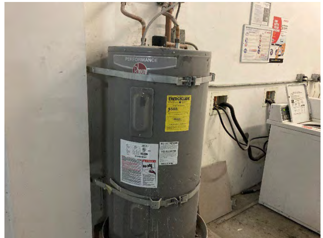
M-10. Bldg 5733E: Laundry room domestic water heater.
