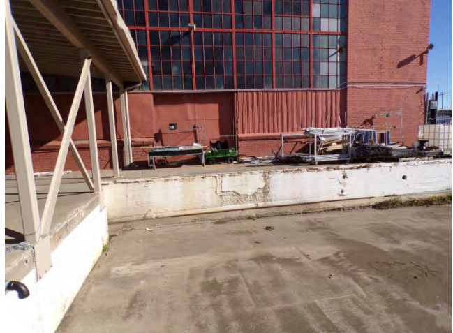
128. Various deficiencies were observed in loading areas. Degraded concrete shown.
