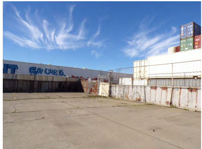
40. Bldg 5601W: Concrete parking area on north side of building. Site fencing is in an overall run-down condition in this portion of the property.
