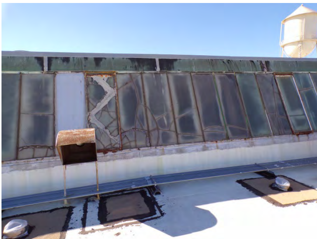
59. Bldg 5601E: Numerous broken windows were observed in the clerestories.
