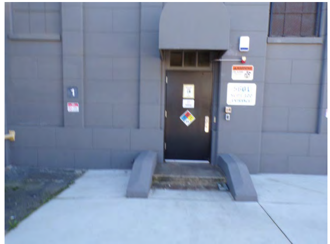
10. Bldg 5601E: Secondary entrance along San Leandro Street. Entrance is not wheelchair accessible.
