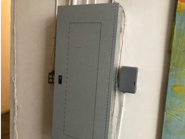
M-7. Bldg 5733E: Electrical distribution panel.
