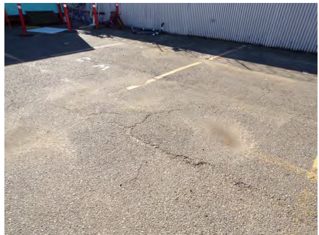
48. Bldg 5733W: Degraded condition of asphalt paving.
