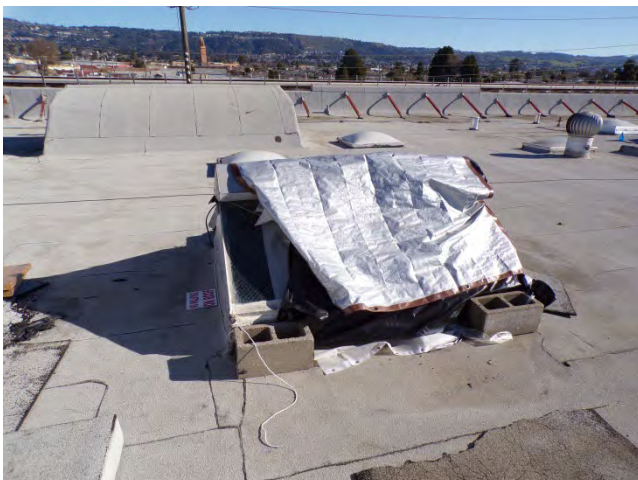
71. Bldg 5733E: Tenants have installed plastic sheeting on skylights that presumably leak.
