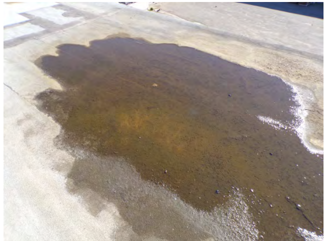
82. Bldg 5733W: Ponded water was present on the day of our site visit.
