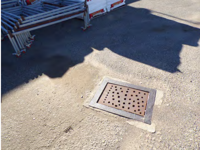
49. Bldg 5733W: Degraded condition of asphalt paving. Area drains are installed in several locations around the property.
