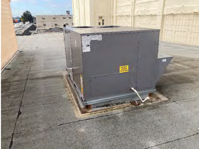
M-1. Bldg 5733E: Packaged air conditioner.
