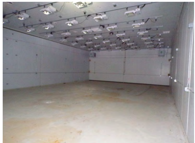
96. Bldg 5601W: Interior finishes, fixtures and equipment in plant cultivation rooms.
