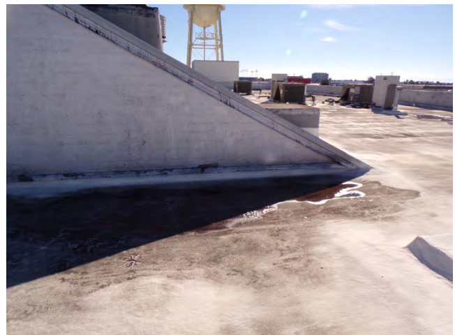
60. Bldg 5601E: Ponded water was observed in multiple locations.
