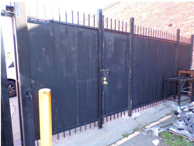
125. Deficiencies with fences and gates were observed. Painted fences should be repainted.
