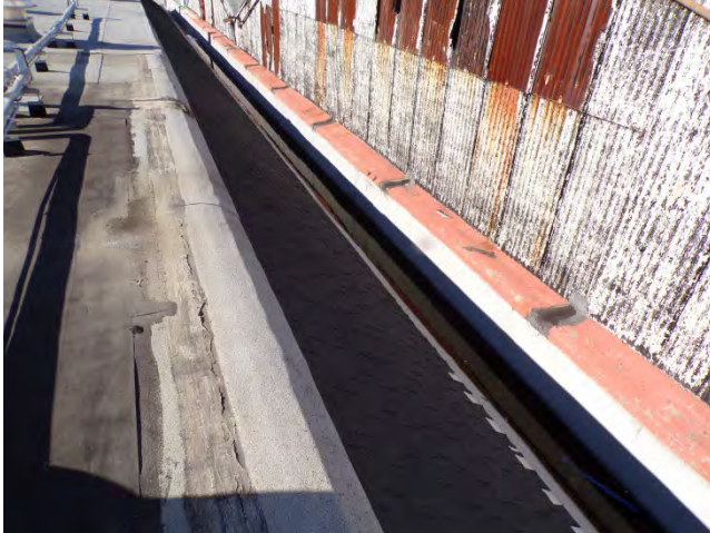
79. Bldg 5733W: Along the north side of the building, ponded water was observed at the foot of the pitched roof along most of its length.
