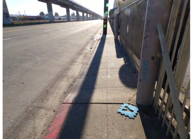
122. Changes in excess of 1/4" in concrete site work create tripping hazards.
