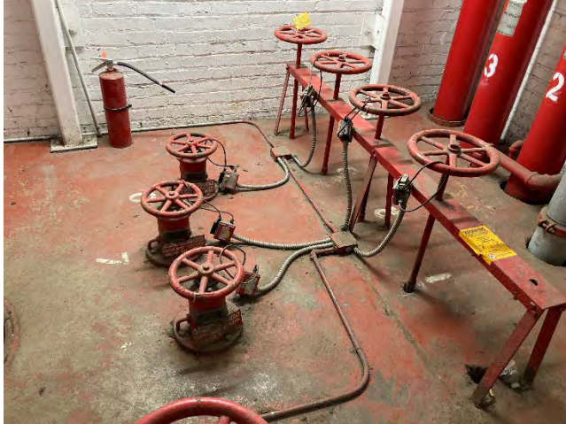
M-13. Bldg 5601 fire sprinkler vault with risers.
