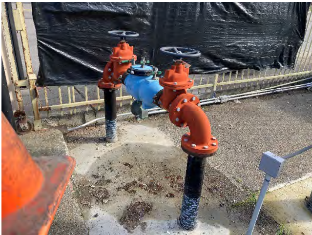
M-9. Bldg 5601: Domestic water service with backflow preventer.
