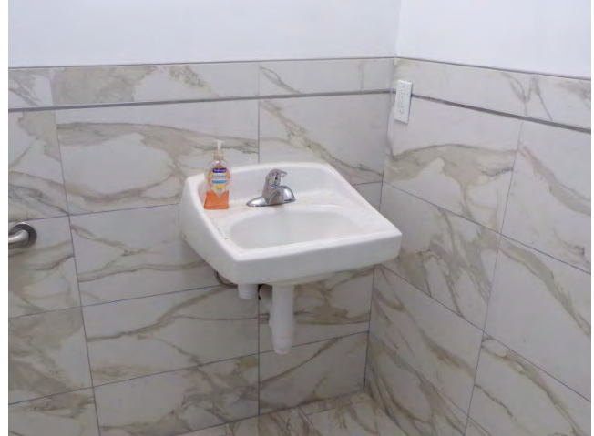
116. Bldg 5601E: Interior finishes and fixtures in restrooms.
