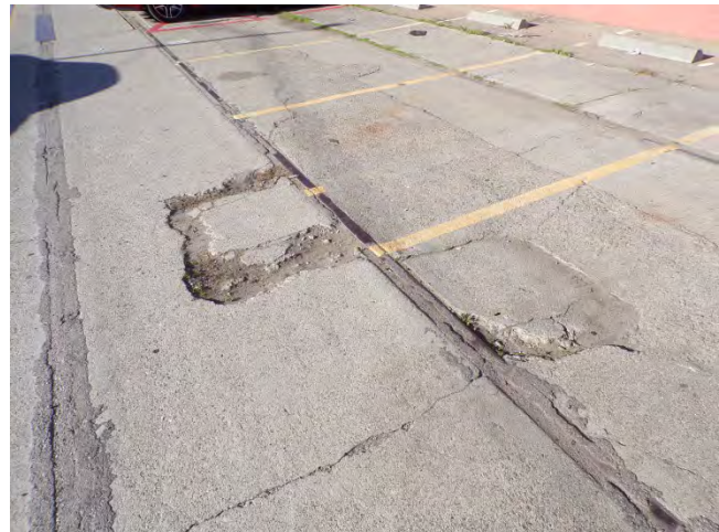
46. Bldg 5733E: Degraded condition of concrete paving.
