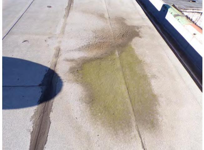
80. Bldg 5733W: The BUR roofing system is in an overall degraded condition. Area of past ponding shown.
