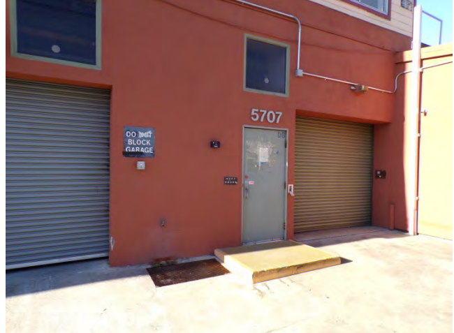
26. Bldg 5733E: Entrances into tenant spaces along the east elevation are not wheelchair accessible.
