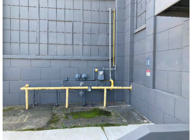
M-8. Bldg 5601E: Natural gas service without seismic safety shutoff valve.
