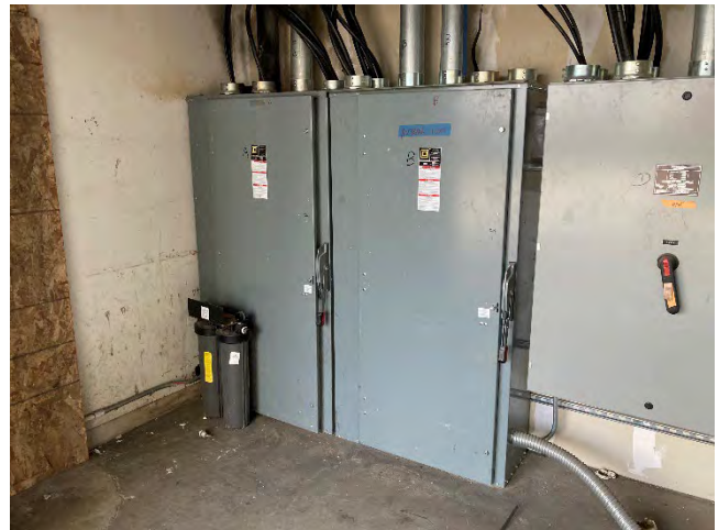
M-4. Bldg 5733E: Main electrical switchgear.
