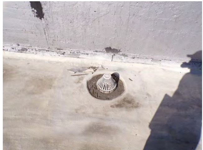
58. Bldg 5601E: Grated roof drains are installed; overflow protection is not provided.
