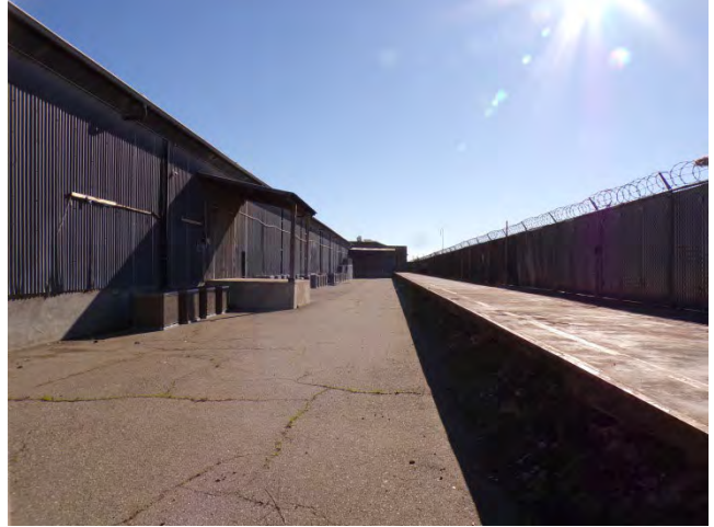
14. Bldg 5601W: Galvanized, ribbed steel wall panels are in an overall degraded condition. Raised concrete loading apron at right.
