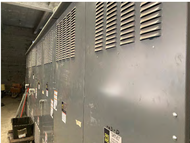
M-5. Bldg 5601E: Main electrical switchgear.
