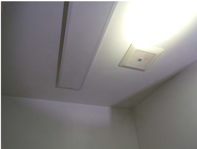
117. Bldg 5601E: Interior finishes and fixtures in restrooms.
