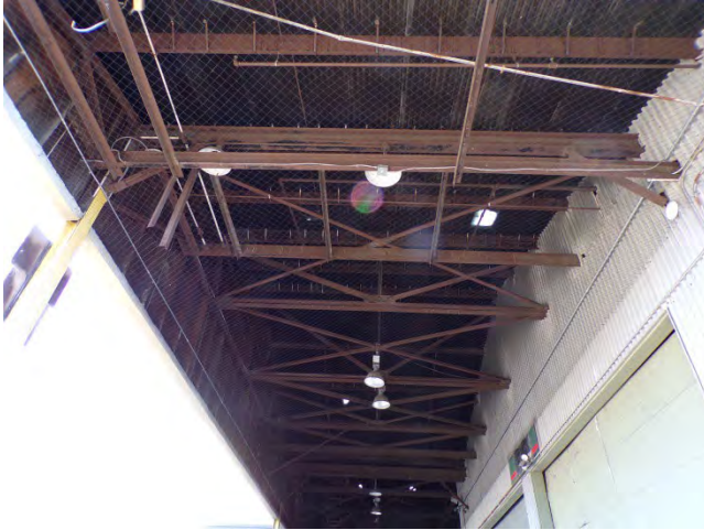
13. Bldg 5601W: Exposed steel structure should be repainted during the reserve term.
