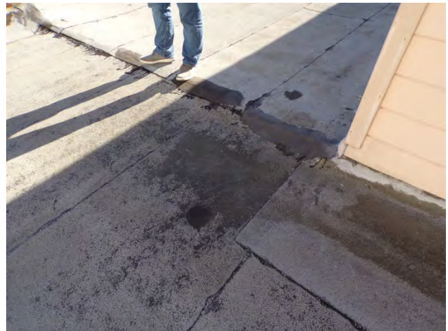
70. Bldg 5733E: The BUR roofing system is in an overall degraded condition.
