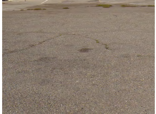
50. Bldg 5733W: Degraded condition of asphalt paving.
