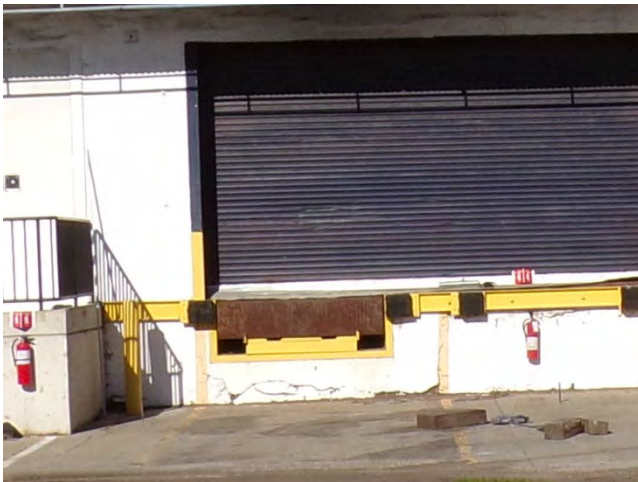
129. Various deficiencies were observed in loading areas. Rusted leveler should be repainted.
