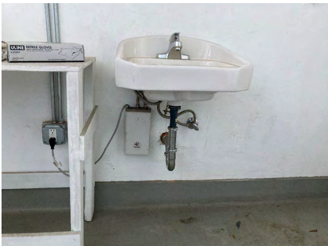
M-11. Bldg 5601E: Under-sink instantaneous electric domestic water heater.
