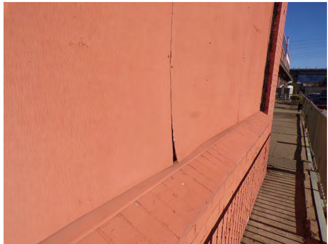
130. Exterior wood was observed in a degraded condition. South elevation of Bldg 5733E shown.
