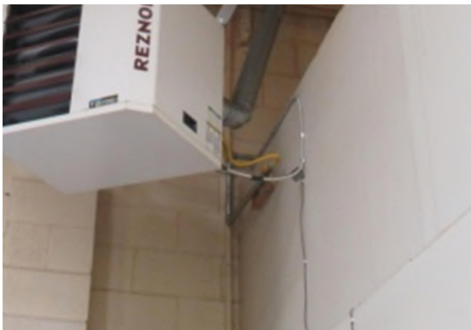
23. Yellow flexible gas connection at the unit heater.
