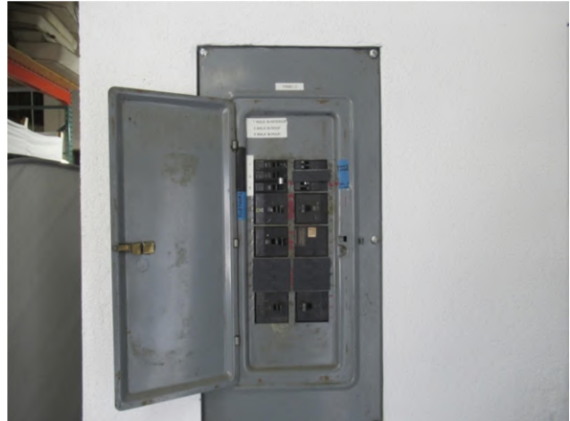
26. The Square D electrical sub-panel in Suite 444.
