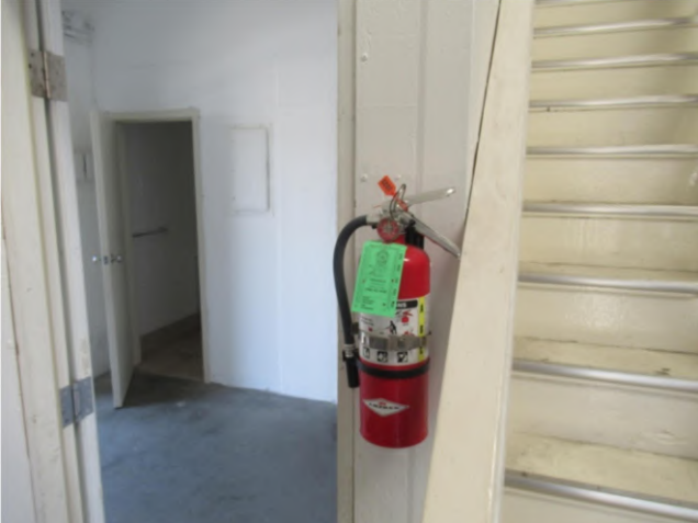
31. The fire extinguisher in Suite 1720 has a valid inspection tag.
