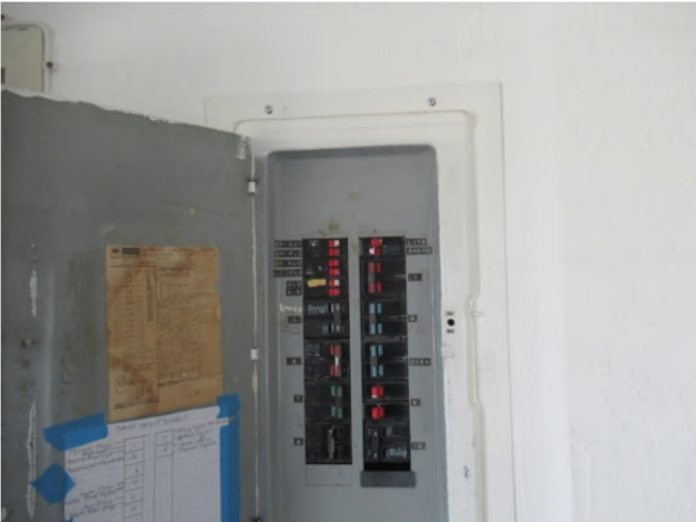
27. The Murray electrical sub-panel in Suite 1720.
