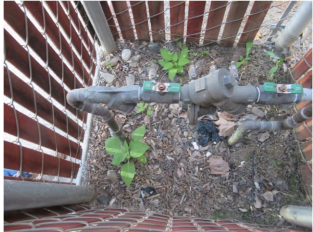
14. The backflow prevention device.
