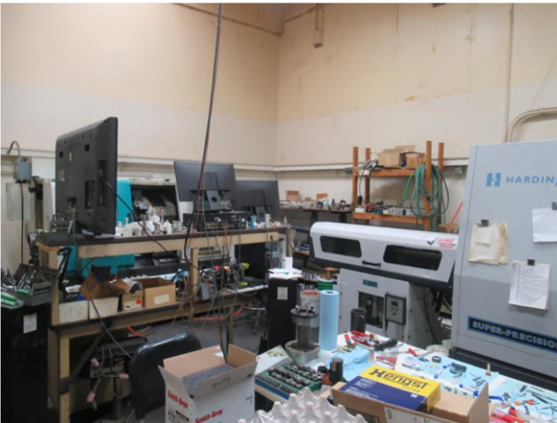
39. First floor interior finishes in Suite 460. This tenant has many pieces of machine equipment installed that obstruct an Accessible path of travel.
