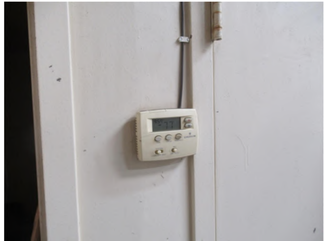
22. The thermostat for the unit heater is digital.
