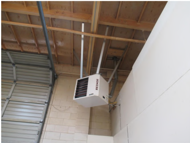
21. A Reznor suspended unit heater is installed in Suite 460.
