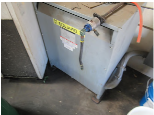
54. A 75 kVA step-up transformer is installed in Suite 460.
