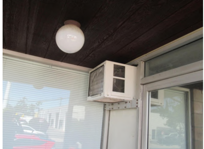
20. This equipment installed in the wall next to the Suite 444 entrance is presumably an air conditioner.
