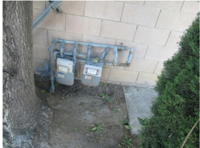
28. The gas service lacks a seismic shutoff valve.
