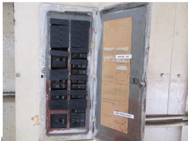
53. The Square D electrical sub-panel in Suite 460.
