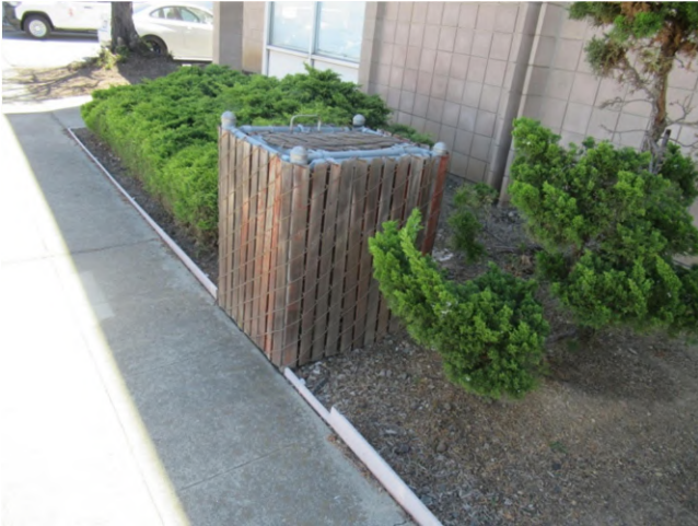
13. The public sidewalk along Lano Street. The small, fenced enclosure contains a backflow prevention device at the water service entrance.
