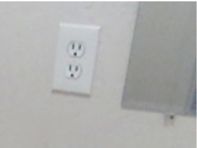
35. Non-GFCI receptacles are installed in wet areas. Suite 444 restroom shown.
