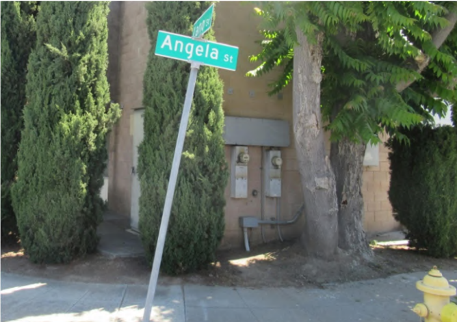
25. It was reported that the building owner upgraded the electrical service with the equipment and meters shown at center. This equipment is just around the corner from the main service, which is partially in view at left.
