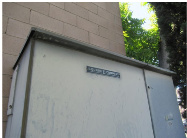
24. The main electrical service is a Square D panel. The enclosure's door could not be opened; interior access was not possible.
