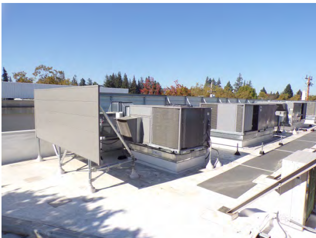
53. Four Carrier packaged units are located on the south side of the roof. Screens for HVAC equipment also shown.
