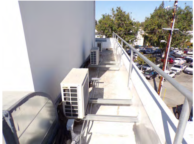
58. Three Daikin heat pumps are installed on the north side of the roof; each has a one ton cooling capacity.
