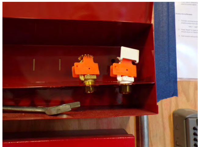
78. Only two spare sprinkler heads are in the sprinkler head spares box; six are required, as is a wrench (shown). The box is in the main service room next to the FACP.
