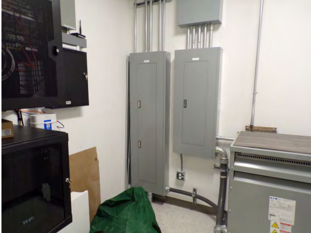
61. Electric distribution system sub-panels are located in secondary service rooms on both floors.
