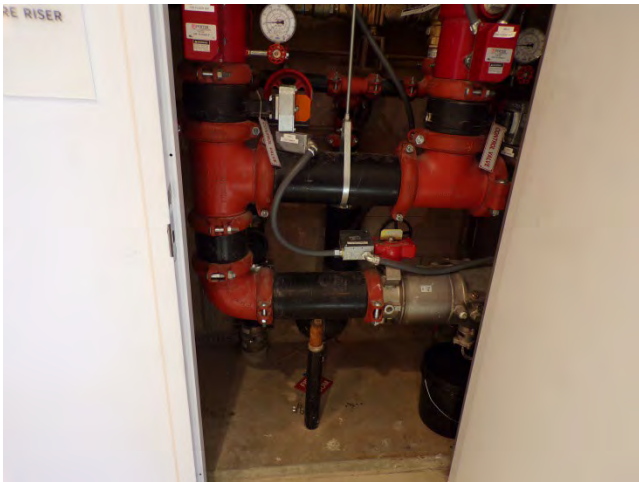
75. The two 6" fire sprinkler risers are located in a service closet near the northeast corner of the building.
