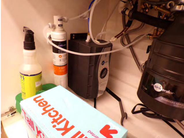
67. Instantaneous electric water heaters are installed in tenant suites in under-counter locations.
