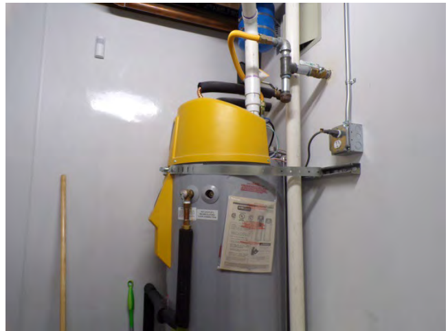
64. A 100 gallon natural gas-fired water heater is installed in the second floor janitor's closet. Flexible gas line connection shown.
