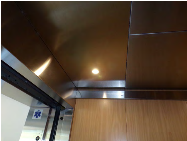
69. Interior finishes and fixtures in elevator.
