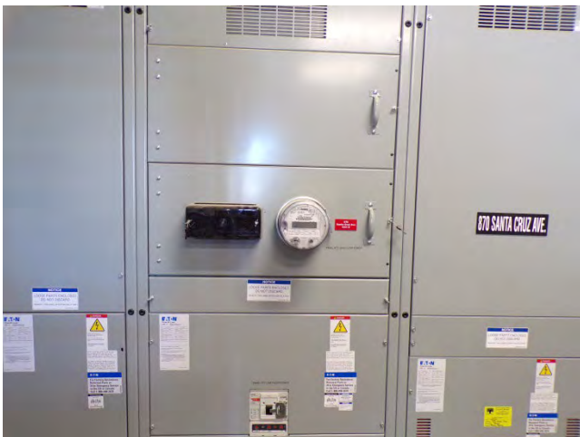
59. The main service entrance panel is rated at 600 amps. It is located in the main service room near the southwest corner of the building.
