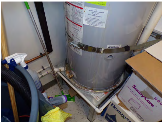
65. The water heater has compliant seismic strapping.
