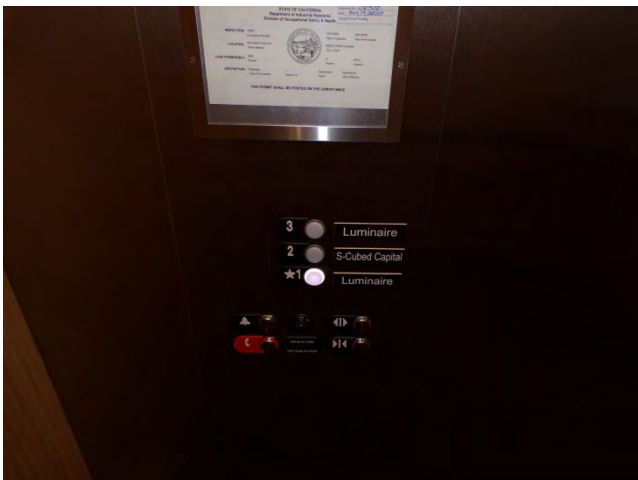
71. Elevator cab control panel.
