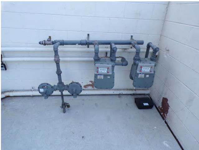
63. The gas service line lacks an automatic seismic shut-off valve.
