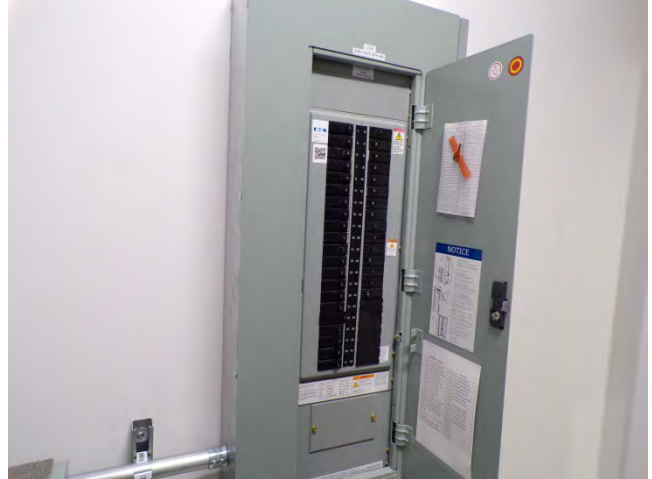
62. No evidence of infrared scanning of the electrical distribution equipment was observed.
