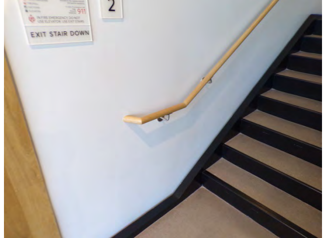
44. Both sets of stairs appeared compliant with current Accessibility requirements.
