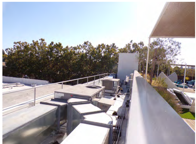
54. Two Carrier packaged units are located on the north side of the roof.
