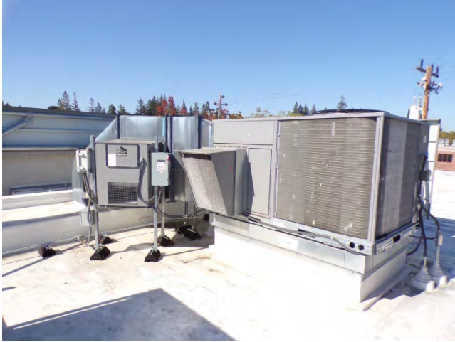
55. The Carrier packaged units were installed in 2022 and appeared in "Good" condition.
