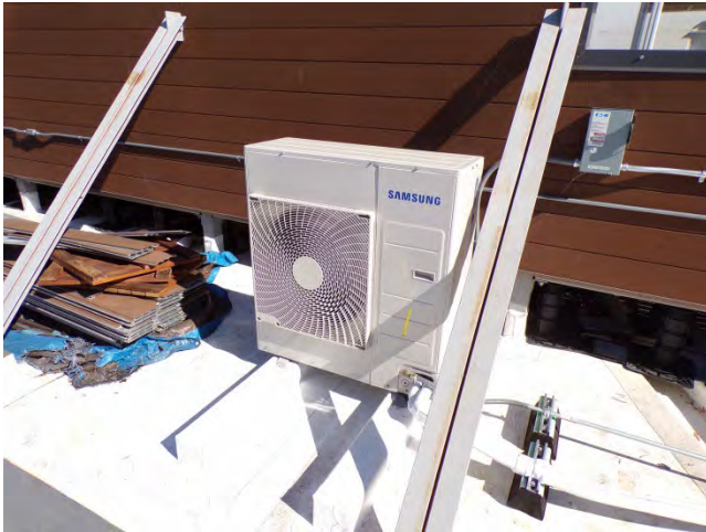
57. One Samsung 2.5 ton heat pump is installed on the south side of the roof.
