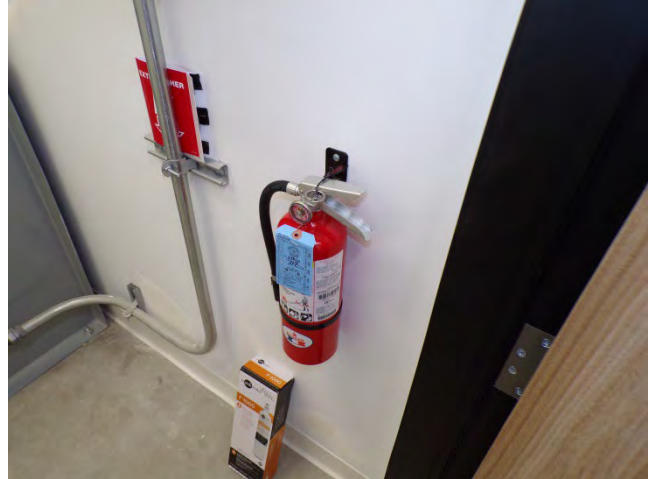
74. All observed fire extinguisher inspection tags were current, dated May 8, 2024.
