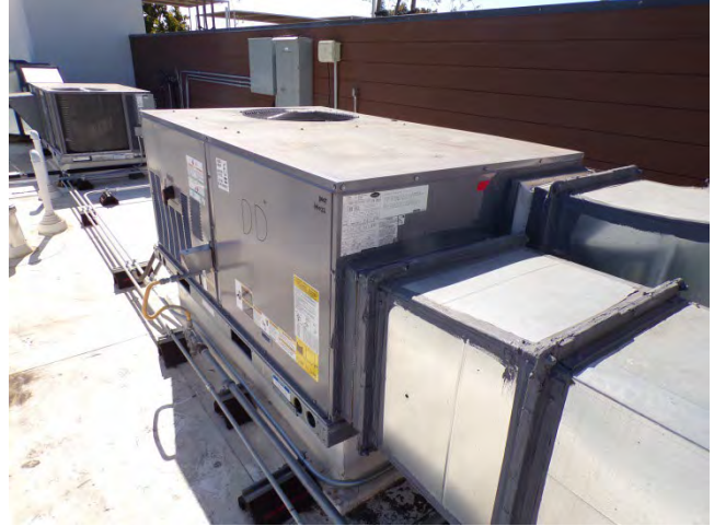
56. All six rooftop furnaces have flexible gas line connections.
