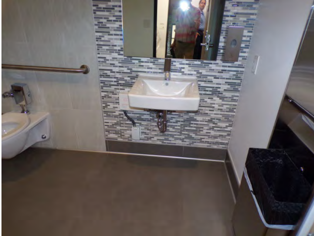
49. Second floor: Interior finishes and fixtures in restrooms. This sink drainpipe lacks required insulation.
