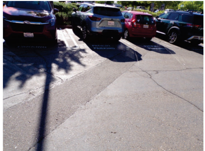
22. MOB 2: Past full-depth repairs and meandering cracking in asphalt paving.
