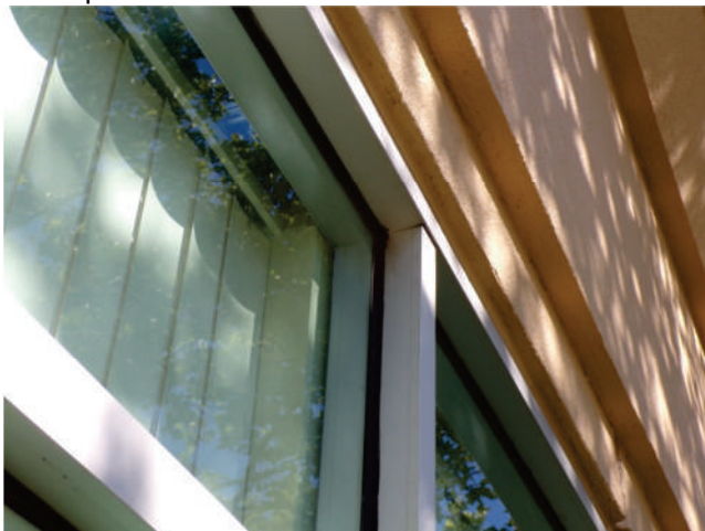
119. A contingency allowance to replace degraded rubber window seals, if applicable, is included in the Spreadsheet. MOB 2 shown.
