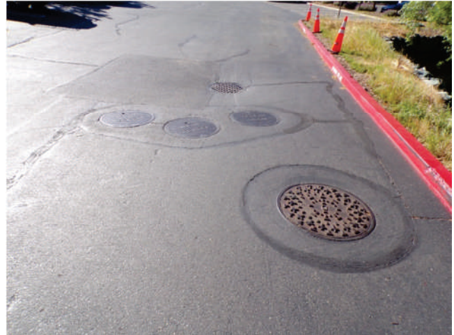
32. MOB 8: Past full-depth repairs. Meandering and linear cracking in asphalt paving also shown.
