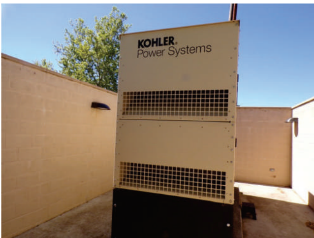
35. MOB 8: The emergency generator serves only MOB 8.
