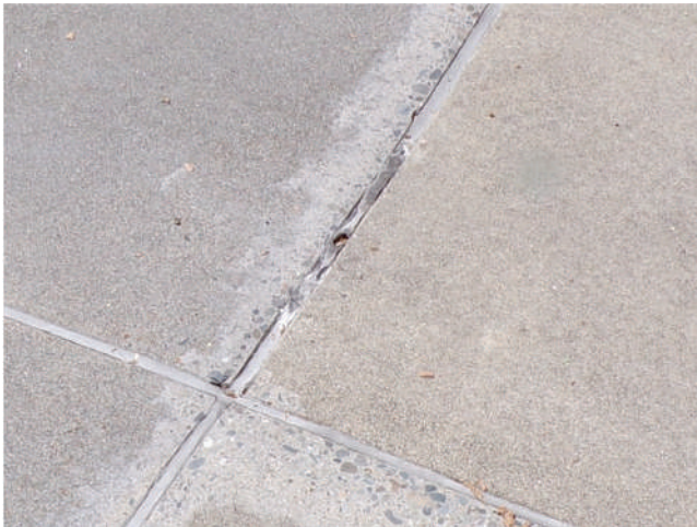
117. An allowance to replace degraded flexible sealants in concrete joints is included in the Spreadsheet. MOB 2 shown.
