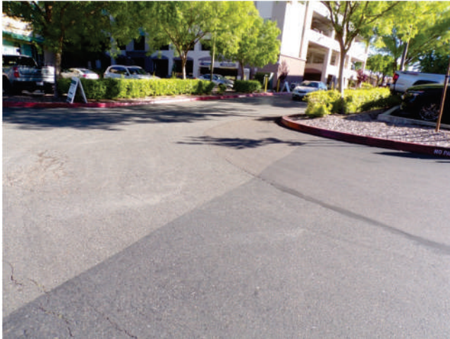
31. MOB 8: Repairs, resealing, and restriping the asphalt paving is recommended.
