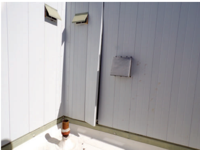
53. MOB 2, south wing: One of the interlocking metal parapet facing panels is misaligned.
