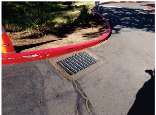
30. MOB 8: Drain inlets are located in several locations in the parking lot. Degraded condition of asphalt paving also shown.
