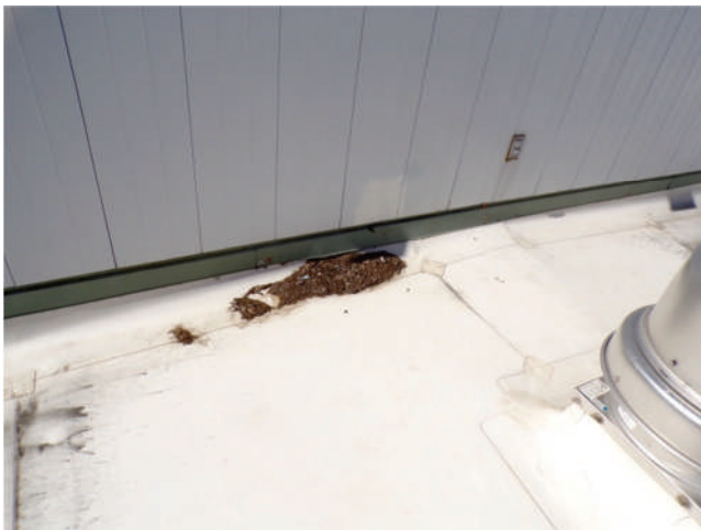
59. MOB 2, north wing: Minor accumulations of dead vegetation and other debris were observed on both the north and south wing flat roof areas.
