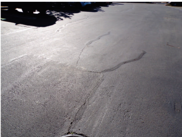
29. MOB 8: Past full-depth repair and meandering cracking in asphalt paving.
