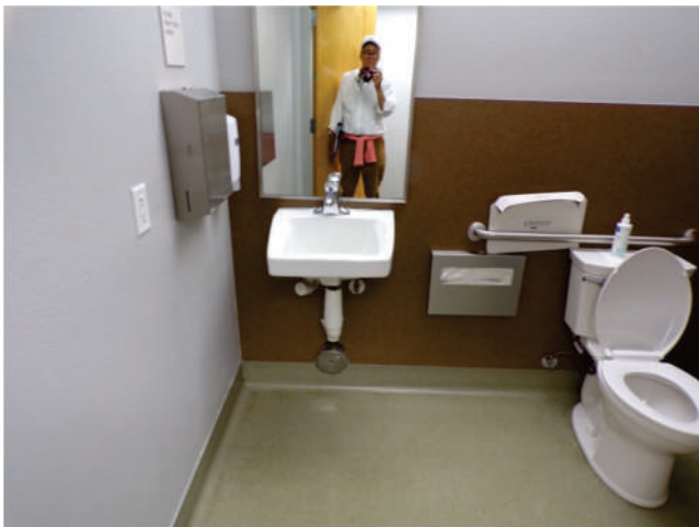
101. MOB 2: Interior finishes and fixtures in older restrooms. Horn/strobe alarm devices are not installed in these restrooms.
