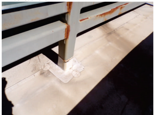
72. MOB 8: We recommend that the mansard frames be treated for rust, primed, and repainted.
