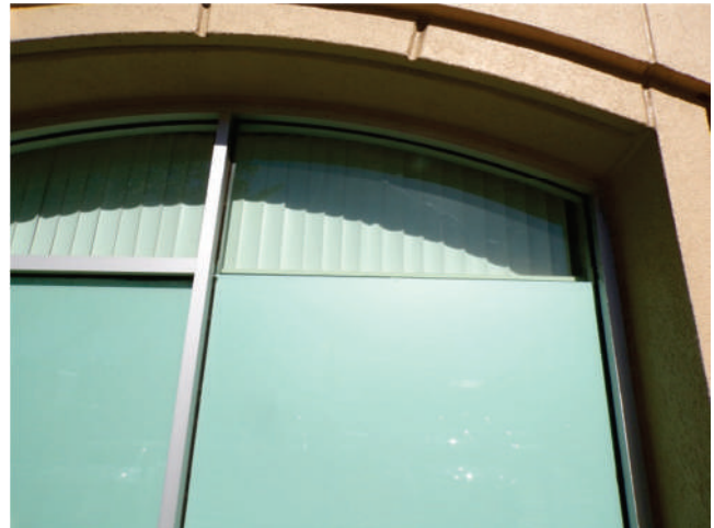
118. MOB 2: An aluminum muntin is missing at a window on the south elevation, east wing.
