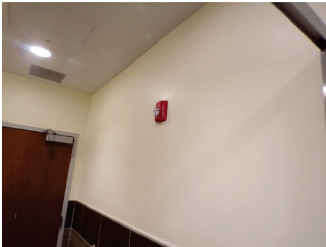
105. MOB 8: Interior finishes and fixtures in restrooms. Horn/strobe alarm devices are installed in all observed restrooms in this building.
