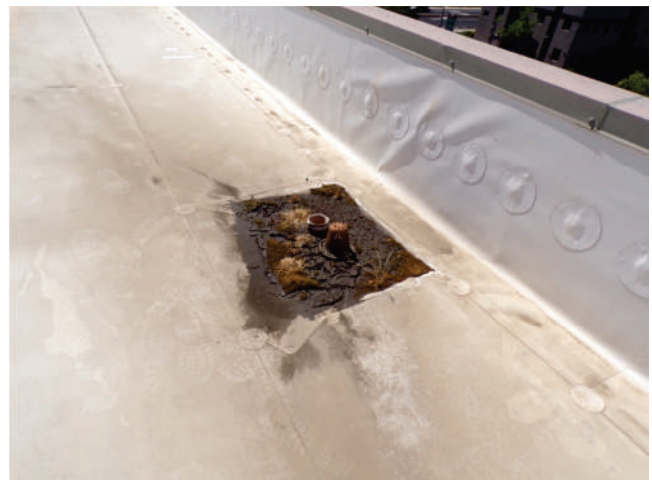
66. MOB 8: Roof and overflow drains are located in shallow sumps. Accumulation of grime in sumps is typical.
