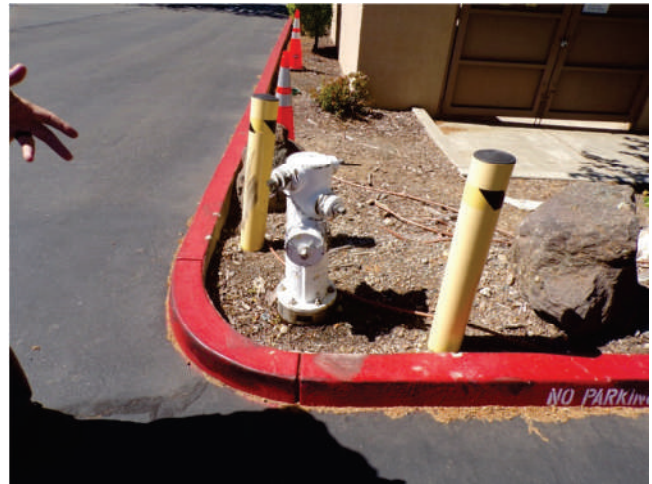
34. MOB 8: Fire hydrant and bollards. The hydrant has been damaged by vehicular contact on two reported occasions. An automatic check valve has been installed at base of hydrant.
