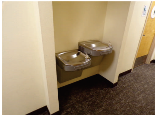
102. High-low water fountain combinations are installed in both subject buildings. MOB 2 shown.
