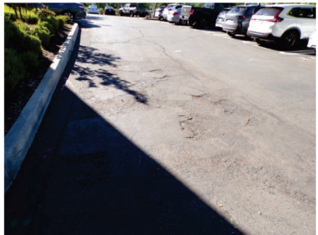
24. MOB 2: Surface degradation of asphalt paving.
