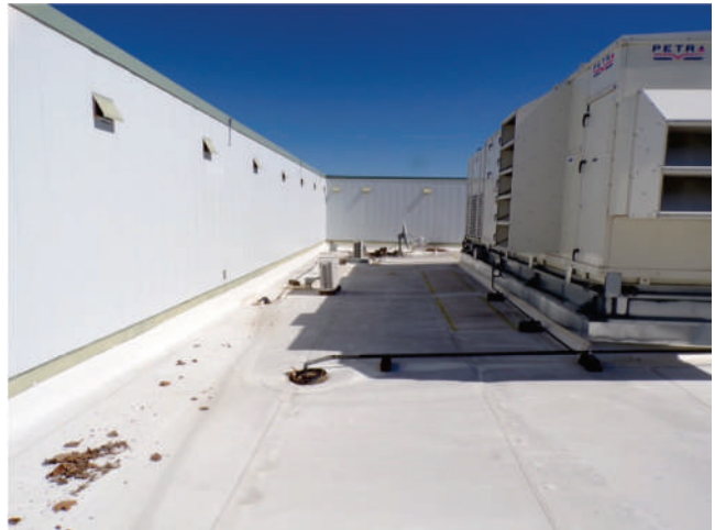
52. MOB 2, south wing: The roofing system appeared in generally "Good" condition.
