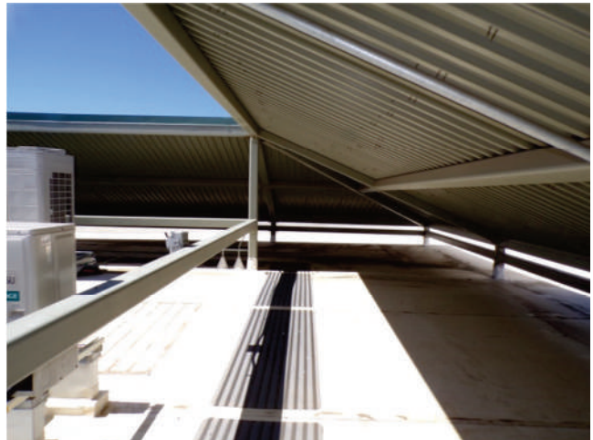
70. MOB 2: The mansards on this building do not function as true roofs in the sense that they do act as a weatherseal for the interior areas beneath them.
