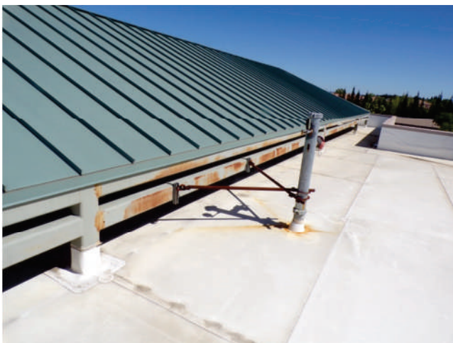
71. MOB 2: Rust is prevalent on the painted steel mansard frames.
