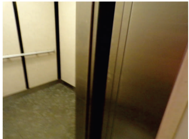
120. MOB 2: Both elevators in this building have door closure arrestors that require physical contact to activate.
