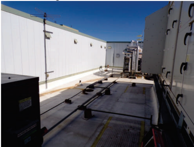
57. MOB 2, north wing: Rust stains are caused by the boiler on this wing's roof.
