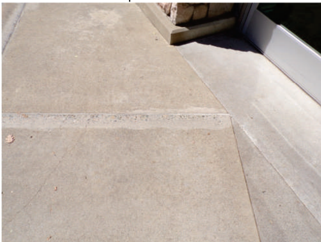
41. MOB 2: Evidence of past concrete grinding.
