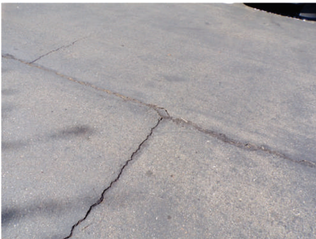
23. MOB 2: Linear cracking in asphalt paving.
