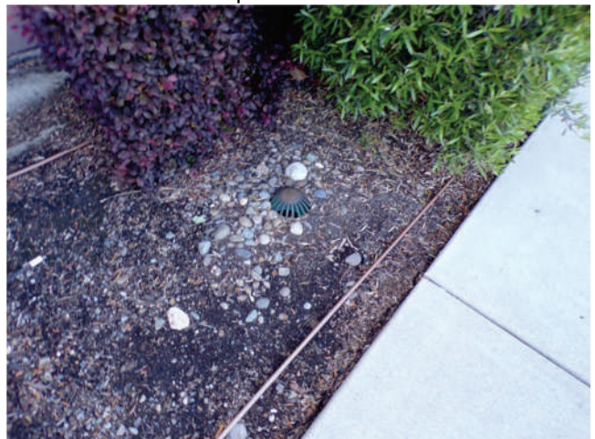
48. MOB 8: Drain inlets are also located in landscaped areas.
