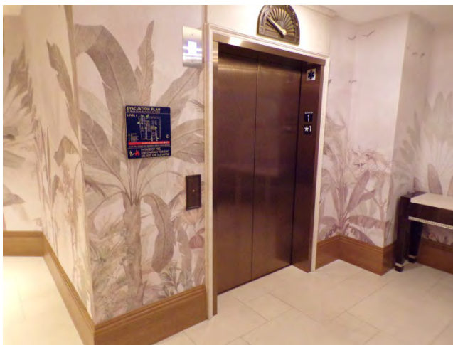
81. Main Bldg: Three Otis passenger elevators are installed.
