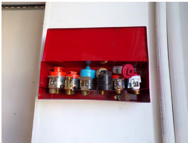
74. Main Bldg: A box of spare sprinkler heads is located in the FACP service room, as required.
