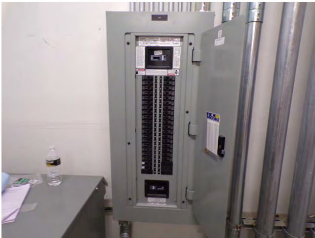
63. Main Bldg: Numerous sub-panels, also manufactured by Siemens , are installed.
