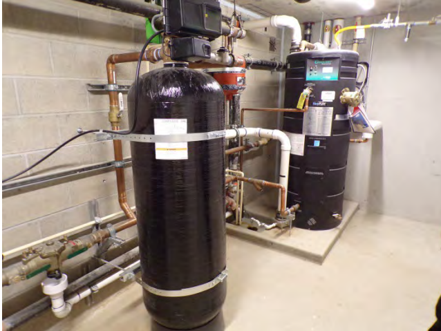
67. Main Bldg: A dedicated water heater and filtration tank serve the laundry room.
