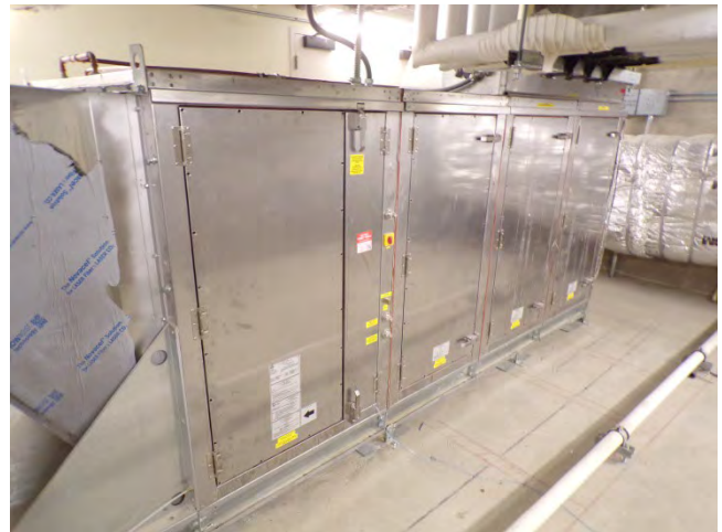
58. Main Bldg: Interior CaptiveAire air handler for pollution control units for garage ventilation.
