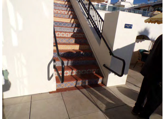
44. Main Bldg: Numerous sets of exterior stairs are installed.
