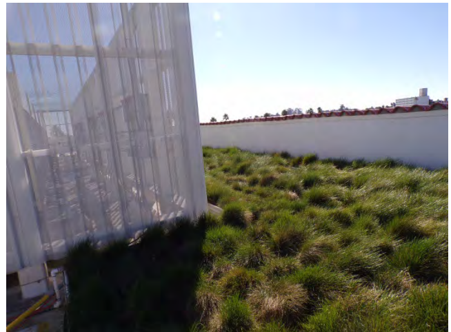
16. Main Bldg: Green roofing systems are installed over approximately 25% of the roof area.
