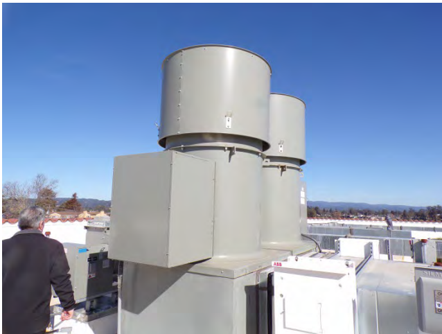
57. Main Bldg: Roof-mounted Greenheck pollution control units for garage ventilation.
