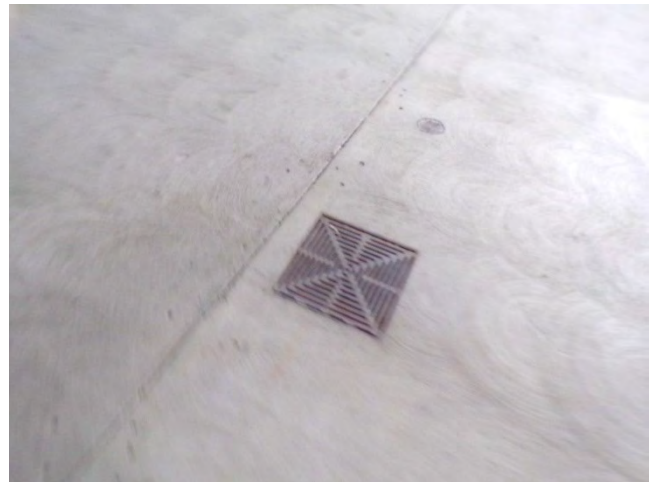
52. Main Bldg: Area drains are provided on the basement level of the parking garage.
