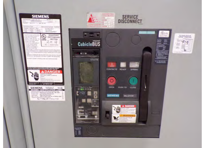
62. Main Bldg: The 3,000 amp main circuit breaker was ground fault performance tested on August 24, 2024. Re-testing is required on a three-year interval.
