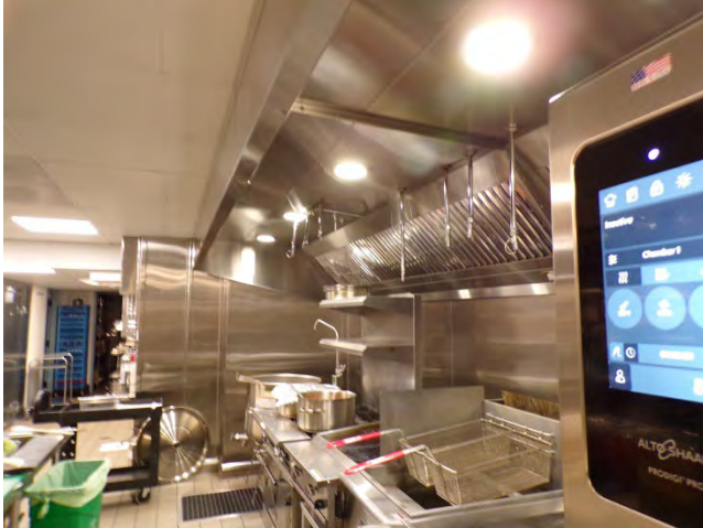
31. Main Bldg: Interior finishes and fixtures in kitchens. ANSUL fire suppression systems are installed above cooktops.
