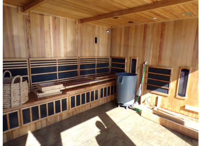
98. Main Bldg: The sauna room suffered water flooding during a storm and the floor was damaged; repairs are underway.
