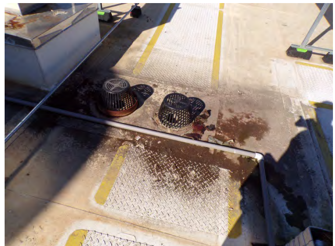
18. Main Bldg: Roof and overflow drain combinations are installed. Evidence of past ponded water also shown.
