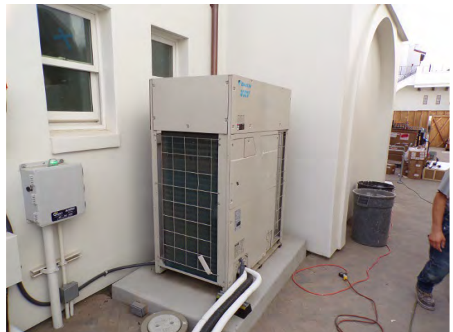
60. Tower Bldg: The Daikin 12 ton heat pump system is reportedly the only source of heated and cooled air for this building.
