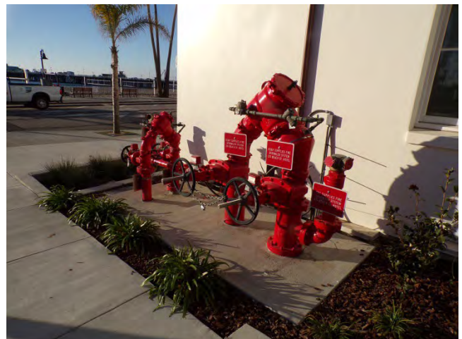
72. Four inch (left) and an eight inch (center) backflow prevention devices are provided. Tower Bldg in background.
