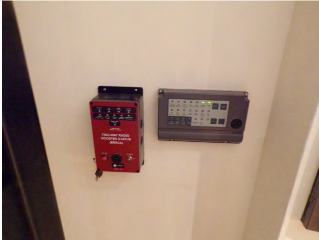
79. An ERRCS system is installed.
