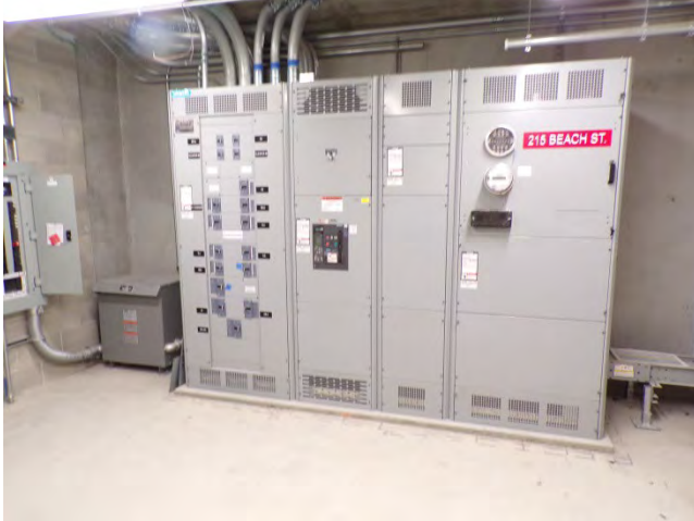
61. Main Bldg: The 3,000 amp main service entrance panel was manufactured by Siemens .
