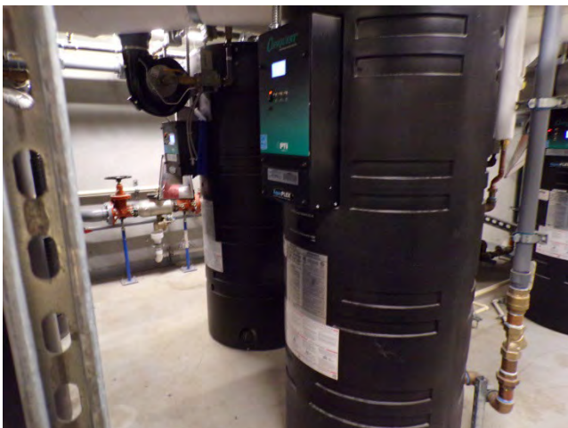
65. Main Bldg: Four natural gas-fired water heaters, manufactured by Conquest/PVI , are provided for general hotel use.
