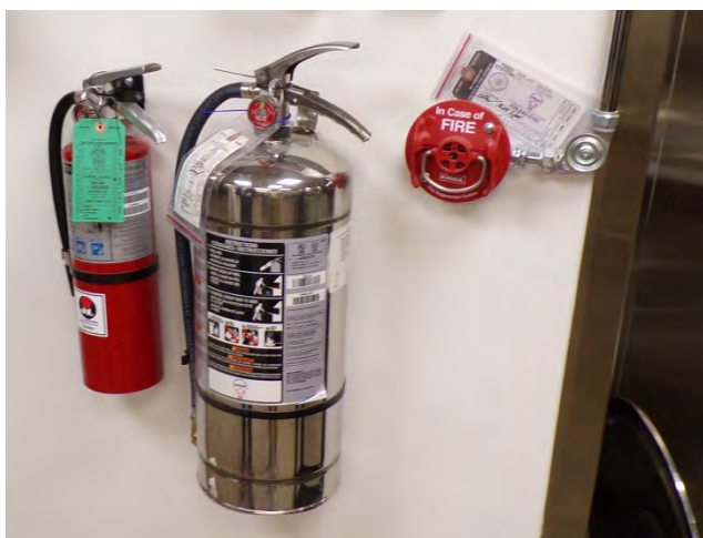
78. Manual pull stations were observed in a few locations. The silver fire extinguisher is a 10 lb. Class K-type, which are provided in the kitchens.
