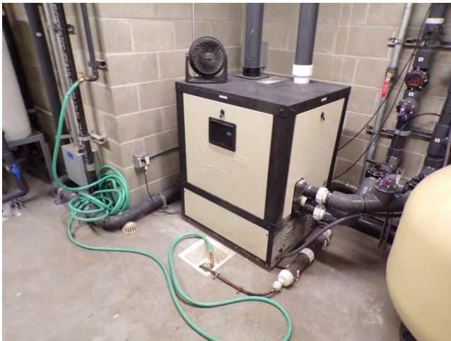
69. Main Bldg: Two Pentair ETi 400 natural gas-fired pool heaters are provided as are filtering equipment and two pumps. One pool water heater serves the swimming pool; the other serves the spa pool.
