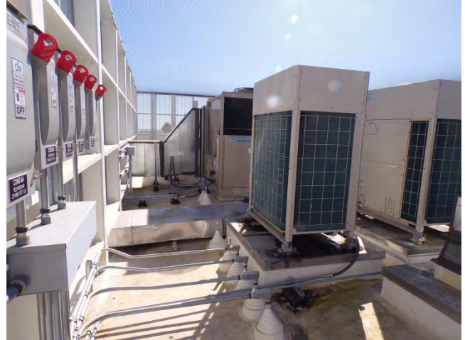
56. Main Bldg: Daikin air source heat recovery VRV units.
