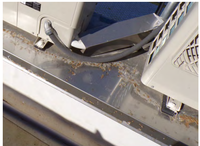
102. Main Bldg: Rust on steel caps on HVAC equipment curbs where plastic film coating is damaged.
