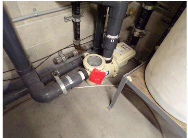
70. Main Bldg: Two Pentair water pumps are provided for the pool equipment. Pool pump shown.
