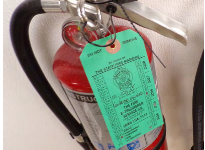
80. Five lb. ABC-type dry chemical fire extinguishers are installed throughout. All observed fire extinguishers had current inspection tags.
