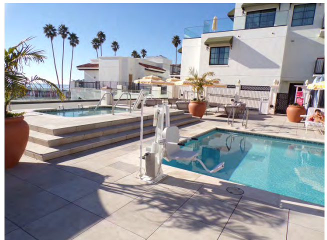
96. Main Bldg: An anchored pool chair lift is installed near the swimming pool. The portable lift was not observed.
