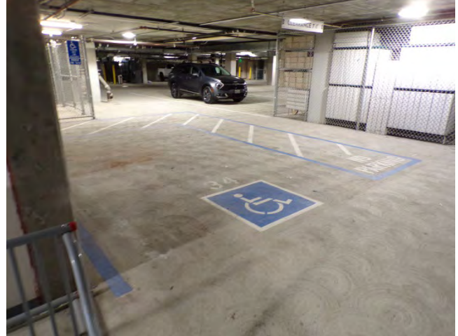
50. Main Bldg: Seven Disabled Accessible parking stalls are provided, two of which are Van Accessible (shown).
