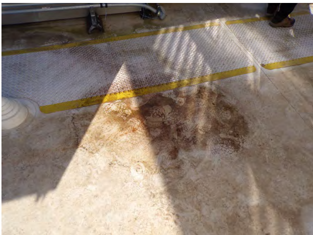
17. Main Bldg: TPO roof staining from past ponded water shown. Allwest recommends a contract for annual roof inspections and cleanings be initiated and maintained for both buildings.
