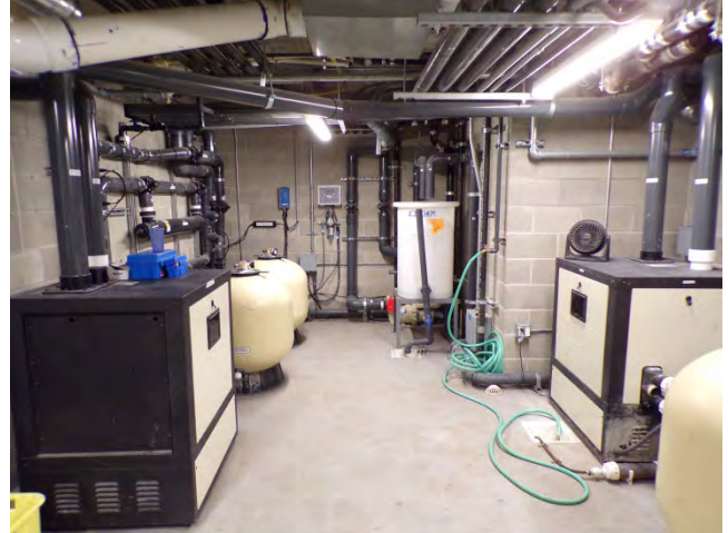
68. Main Bldg: The pool equipment is located in a dedicated service room.
