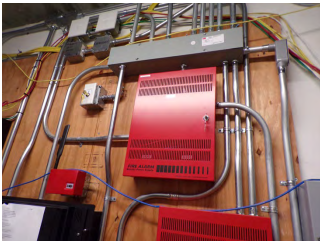
73. Main Bldg: The main FACP is located in a dedicated service room on the north side of the building. The FACP serves both buildings.
