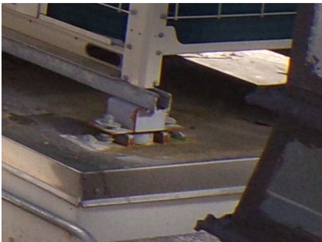
101. Main Bldg: Rust on steel supports for HVAC equipment.
