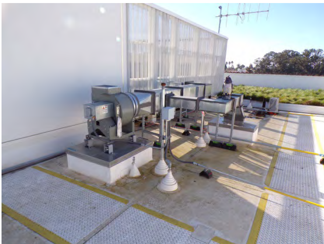
59. Main Bldg: Roof-mounted exhaust fans and ductwork.
