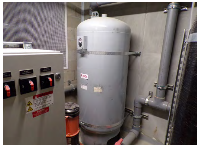
66. Main Bldg: The domestic hot water system is supplemented by two 132 gallon hot water storage tanks, both manufactured by Elbi .
