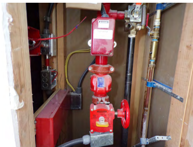
76. Tower Bldg: Sprinkler riser. Box of spare sprinkler heads at lower left.
