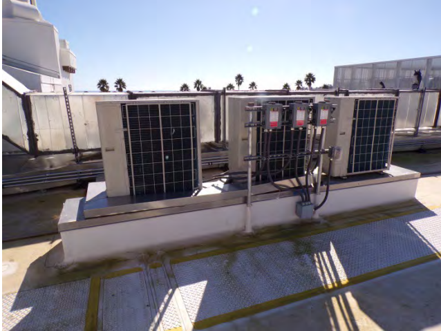
55. Main Bldg: Daikin split-system heat pumps.
