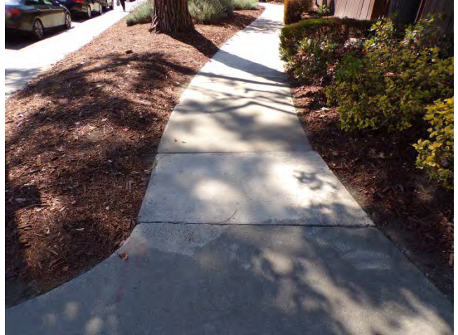
98. Changes in elevation greater than 1/4" in concrete site work create tripping hazards.
