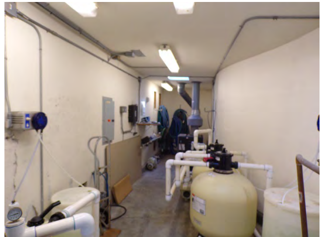
76. Clubhouse: Interior finishes, fixtures, and equipment in pool equipment room.
