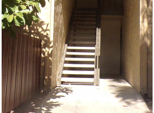
26. Bldg 25: Exterior stairs lack closed risers and handrails on both sides. Guardrails are also non-compliant with current codes.
