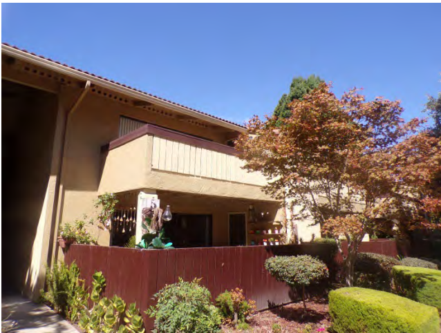
9. Bldg 8: South elevation. Balcony railings have been replaced. This is the older design for the replaced railings with the stucco portion left in place on the short side of the balcony.
