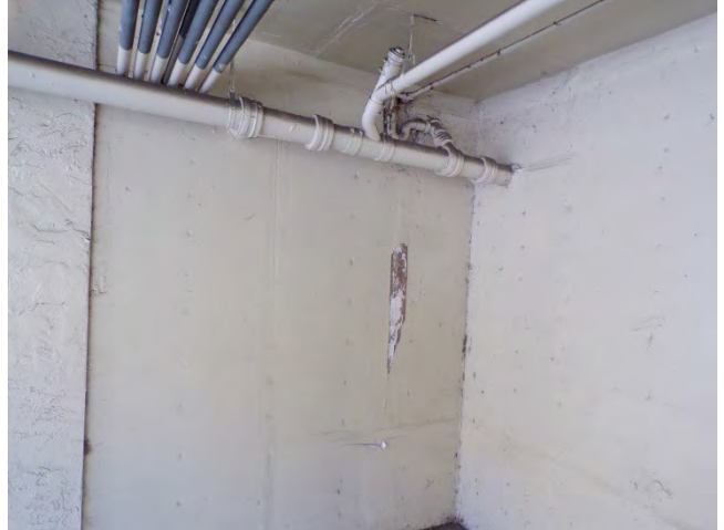
20. Bldg 19: Minor damage to gypsum board finishes—in varying degrees—is typical in tuck-under parking areas.
