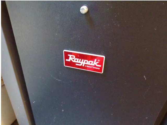
79. Clubhouse: Three Raypak pool water heaters are provided. They were installed in 2017 and 2020.
