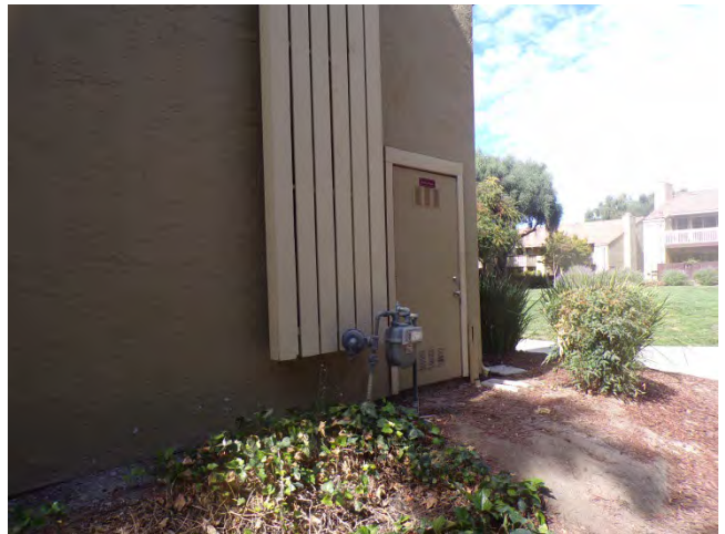
22. Bldg 21: Hot water boilers are located in closets which are accessible from the exterior. Vertically-oriented wood planks are used as a decorative and screening element.
