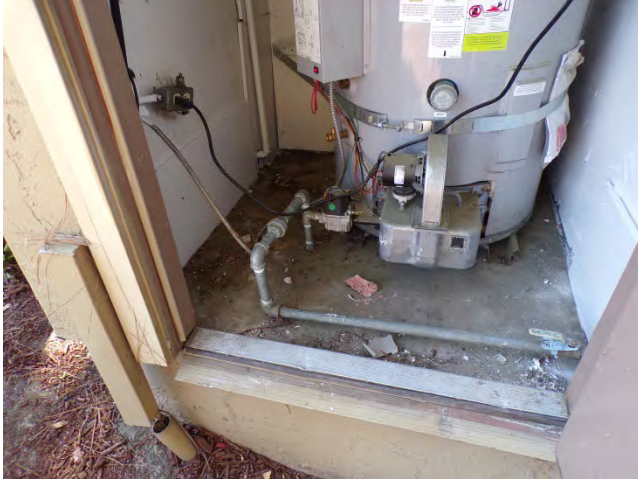
109. Rigid gas line connections were observed on some boilers.
