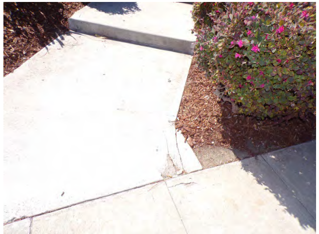
102. Degraded portions of the concrete site were observed in numerous locations.
