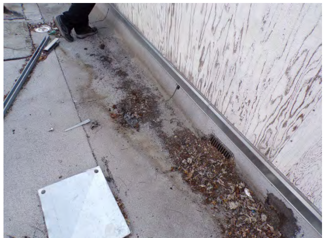
48. Clubhouse: The BUR roofing system should be cleaned of detritus as part of routine maintenance.
