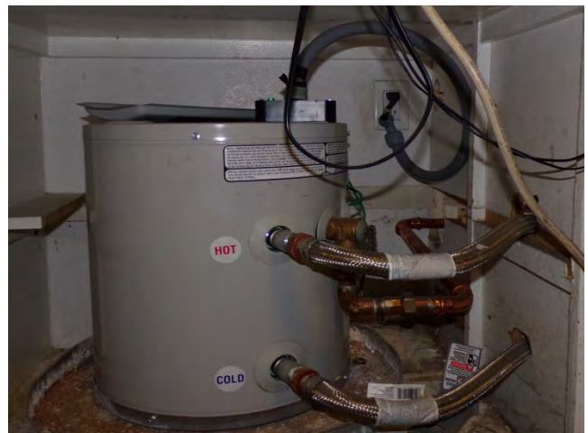
84. Leasing Office: A five gallon electric water heater is installed; it lacks seismic strapping.
