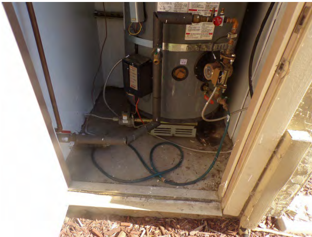
33. Bldg 32: A flexible gas line connection is installed on this building's boiler.
