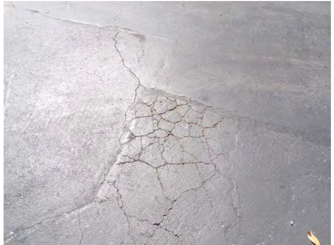
94. Degraded portions of the asphalt paving were observed in numerous locations.
