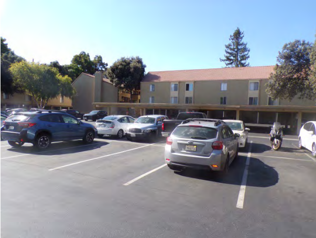
97. Parking stall re-striping will also be required in conjunction with recommended asphalt repairs and re-sealing.
