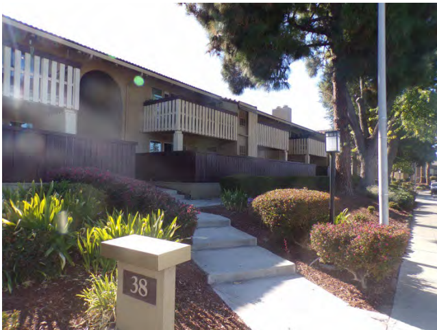
39. Bldg 38: Exterior stairs lacks handrails and tread striping. Second balcony railing update design at far left. First design update shown elsewhere.
