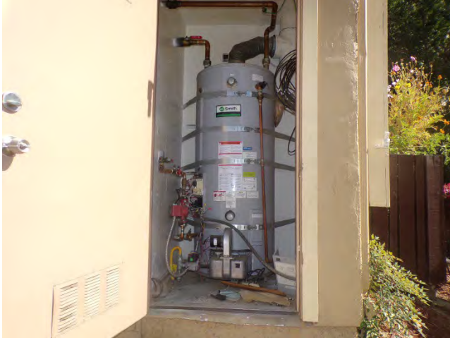
25. Bldg 24: Hot water boilers are located in closets which are accessible from the exterior. Observed boilers were installed between 2004 and 2024. This one was installed in 2017.
