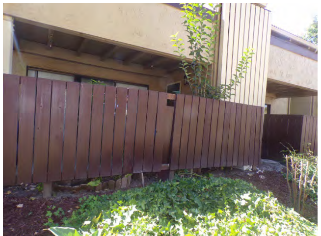
12. Bldg 11: Lower floor patios have painted wood plank railings (fences). Displaced plank is shown at center of photo.
