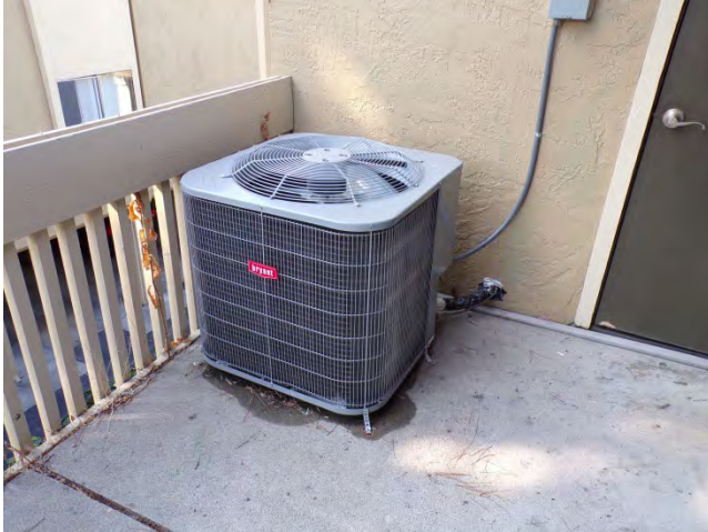
85. Apartment 8C: A two ton Bryant split-system heat pump was installed in 2023. This is one of the newer upgraded air conditioning systems.
