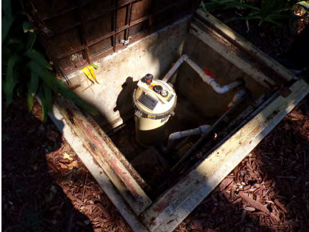
103. There are four fountains on the property; none are functional. Rehabilitation of the fountain equipment is recommended.
