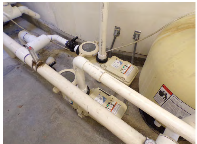
78. Clubhouse: Interior finishes, fixtures, and equipment in pool equipment room. New pool pumps were reportedly installed in 2024.
