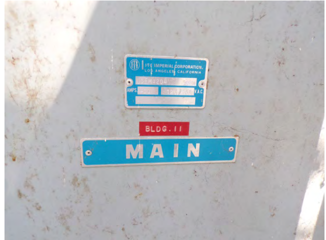
80. Each 12-unit residential building has a 400 amp main service entrance panel, manufactured by ITE. The 8-unit buildings have 200 amp main panels.
