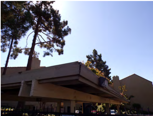
45. Degraded wood elements on carports should be replaced.
