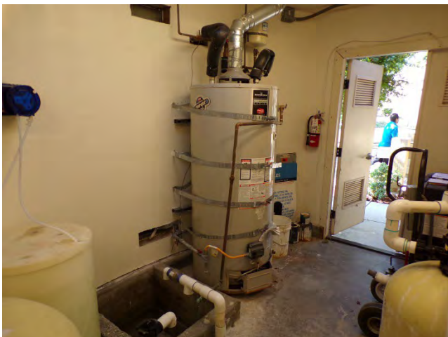
77. Clubhouse: Interior finishes, fixtures, and equipment in pool equipment room. This boiler was installed in 2021.
