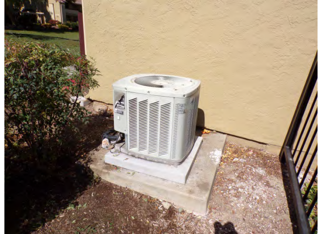
86. Apartment 32J: A three ton Trane split-system air conditioner was installed in 2002. This is one of the older upgraded air conditioning systems. This is the only unit of this type at the property.
