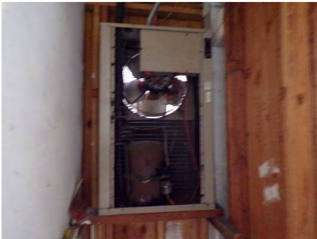
57. Two ton air conditioning units, manufactured by Fedders , are installed in a majority of apartments in exterior service closets. These date to original construction.
