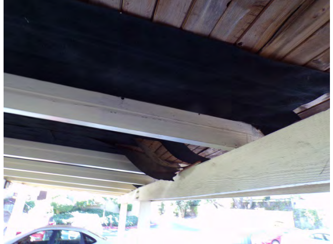
104. The tar paper on the underside of some carports is in a degraded condition.
