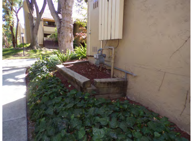
14. Bldg 13: East elevation. Gas meters are installed at each residential building, typically in close proximity to the boiler closet. All gas service lines lack an automatic seismic shut-off valve.
