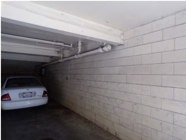
15. Bldg 14: CMU retaining walls in tuck-under parking areas give evidence of water penetration through the walls.
