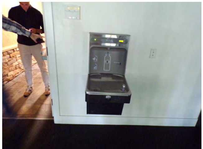
72. Clubhouse: A drinking fountain with bottle fill is installed in the fitness area.
