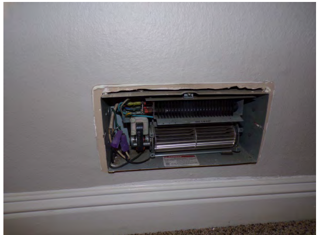
58. Small, electric in-wall heaters are installed in those apartments that have the original air conditioning units.
