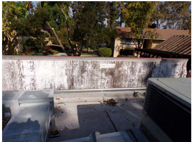
106. Clubhouse: The paint on the plywood facings of the interior side of the parapets is in a degraded condition. Repainting is recommended.
