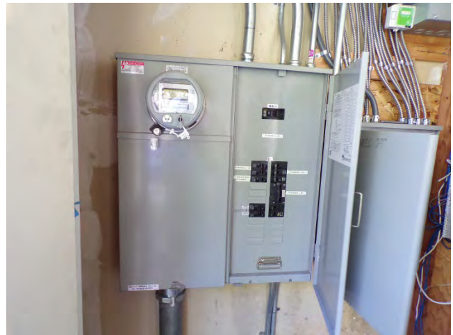
82. Clubhouse: A 200 amp main service entrance panel is installed; it was manufactured by Milbank.
