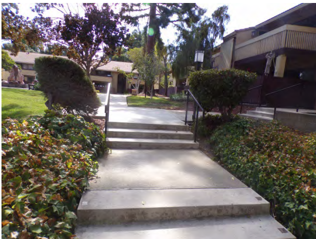
23. Bldg 22 (at right): Handrails are not provided at all exterior walkways (foreground).
