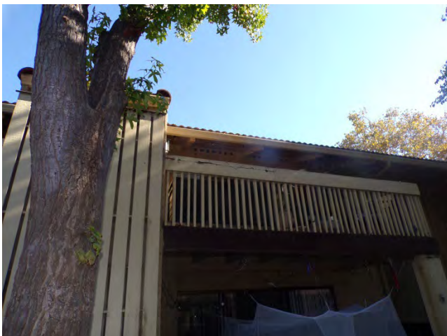
41. Bldg 40: Damaged wood on balcony railing. First railing update design.
