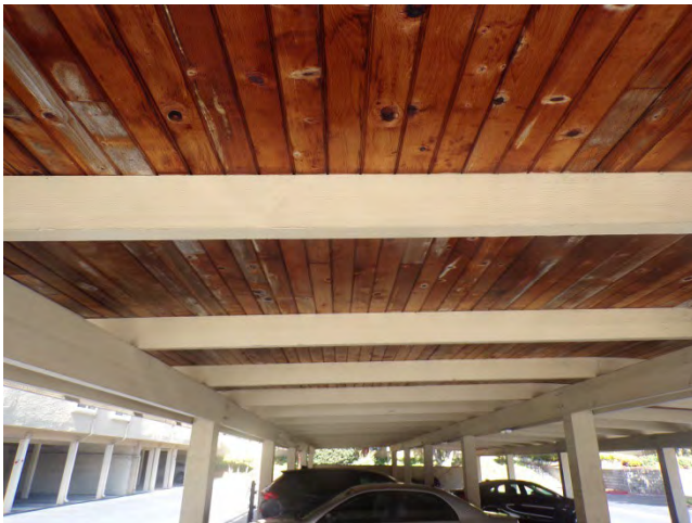
105. At some carports, the tar paper is absent altogether.
