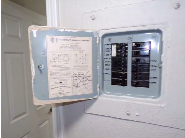
61. Original ITE 125 amp branch circuit breaker panel with original breakers are found in apartments with the older Fedders air conditioners.
