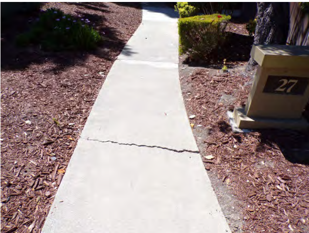
101. Degraded portions of the concrete site were observed in numerous locations.
