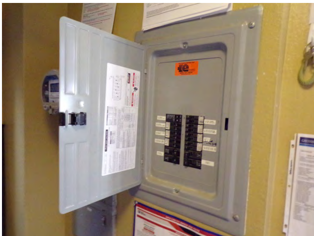
83. Clubhouse: A 125 amp main service entrance panel is installed; it was manufactured by Murray.
