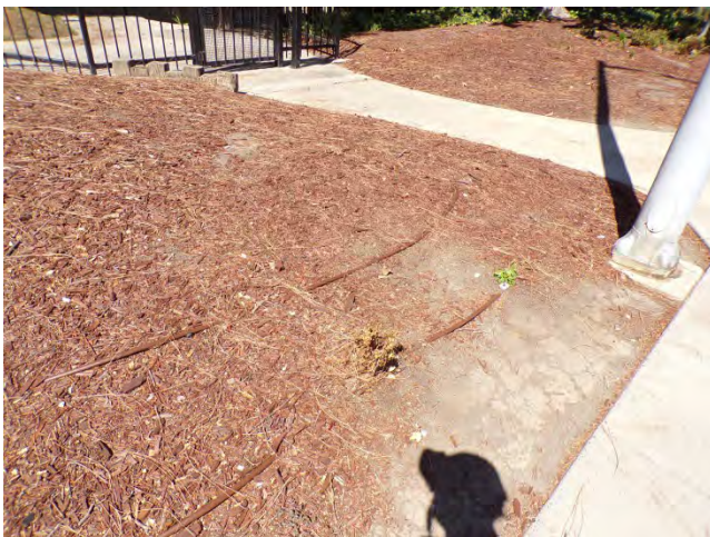
89. Degraded elements of landscaping were observed; dead shrub shown.
