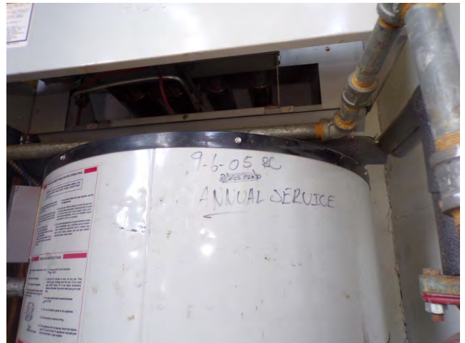
40. Bldg 39: The boiler in this building was the oldest one AllWest observed with a marking indicating September 6, 2005.
