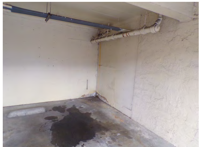
36. Bldg 35: Minor damage to gypsum board finishes—in varying degrees—is typical in tuck-under parking areas.
