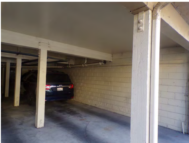
17. Bldg 16: The condition of the finishes in the tuck-under parking areas is typically degraded. Evidence of water penetration through the CMU wall also shown.
