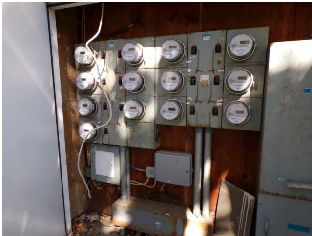
81. Each residential building has a bank of separate meters, one for each apartment and one for common areas.
