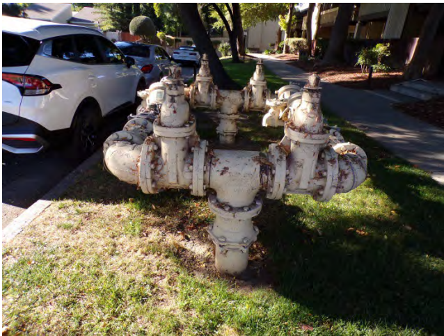
27. Bldg 26 (at right): The backflow prevention device for the domestic water supply is located near this building.
