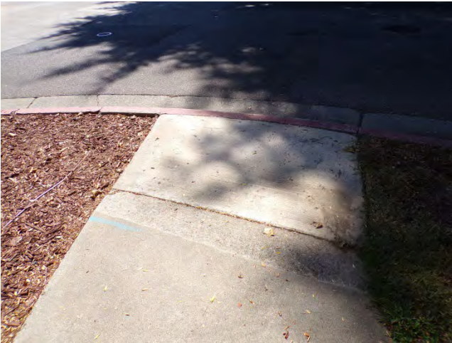
99. Abundant evidence of past concrete grinding to address tripping hazards was observed around the site.
