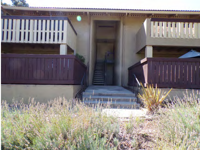
37. Bldg 36: Exterior stairs lack visually contrasting stripes on all treads, as required, except at the Leasing Office. Note the variety in balcony railings.
