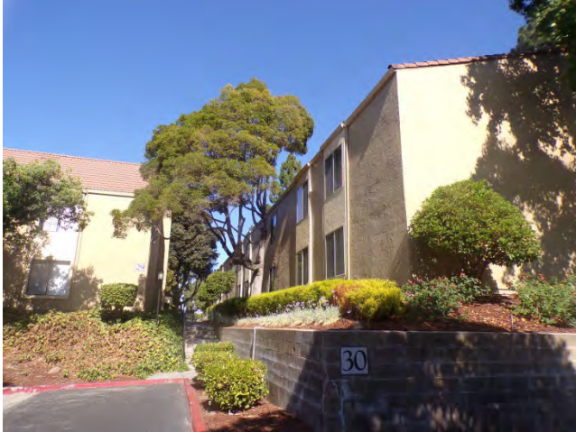
31. Bldg 30: North elevation at center of photo. Efflorescence can be seen on CMU retaining wall.
