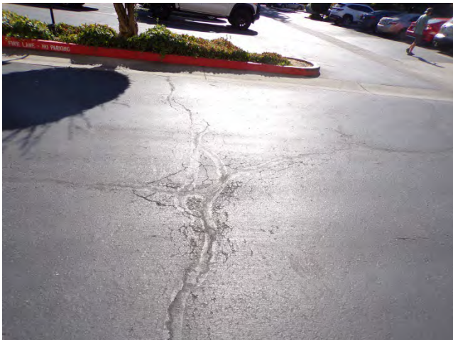
95. Degraded portions of the asphalt paving were observed in numerous locations.
