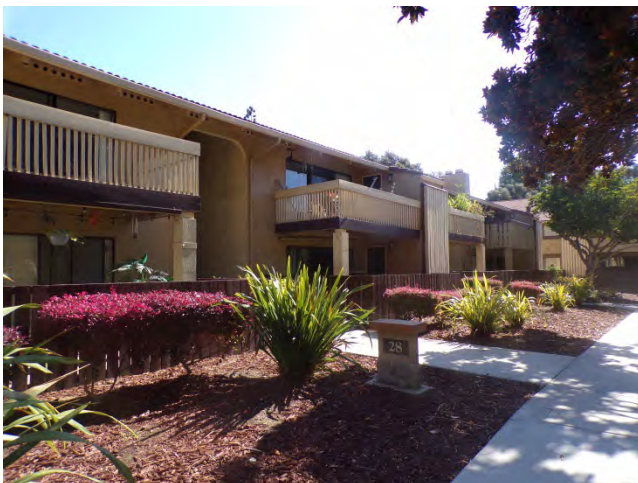
29. Bldg 28: Partial view of north elevation with landscaping. This is the older design for the replaced railings, but the stucco portion has been replaced on the long and the short sides of the balcony.
