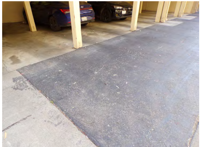
96. AllWest recommends that asphalt repairs and re-sealing be conducted during the reserve term.
