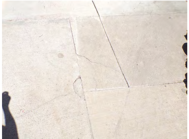
100. Degraded portions of the concrete site were observed in numerous locations.
