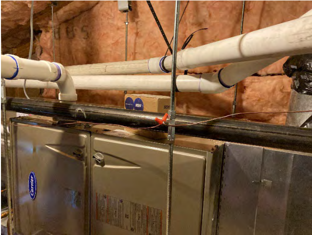
M-1. Main Bldg: Split system fan coil unit.
