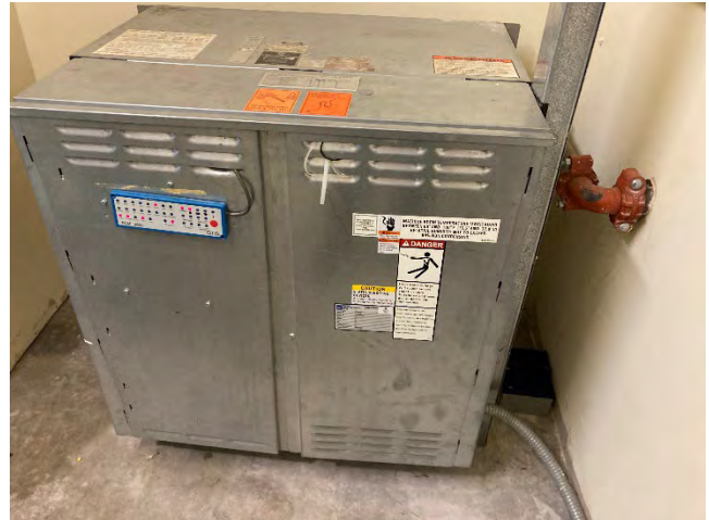
M-32. Gym: Hydraulic elevator drive machine and controller.
