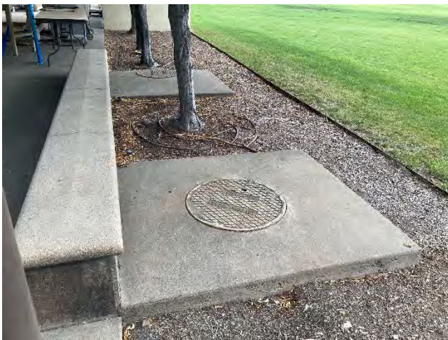
M-21. Main Bldg: Kitchen grease interceptor.
