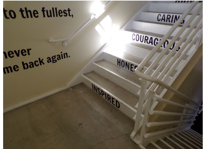
62. Gym: Stairs lack compliant visually contrasting striping at top and bottom treads.
