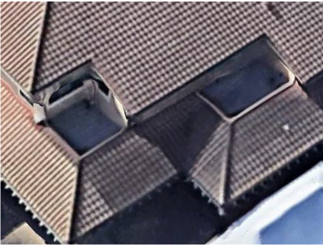
81. Gym: Two small areas of BUR are recommended for replacement.
