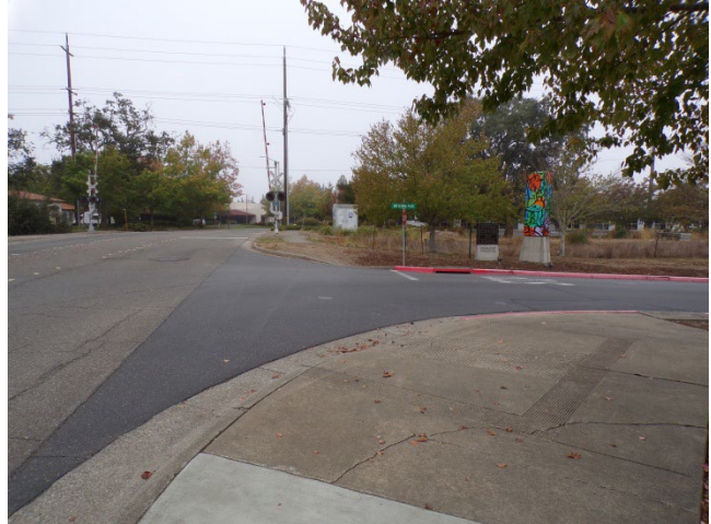
92. The curb ramp (foreground) lacks truncated domes; the far corner lacks a curb ramp altogether.
