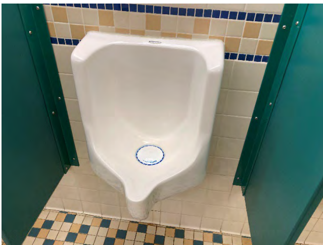
M-23. New waterless restroom urinal.
