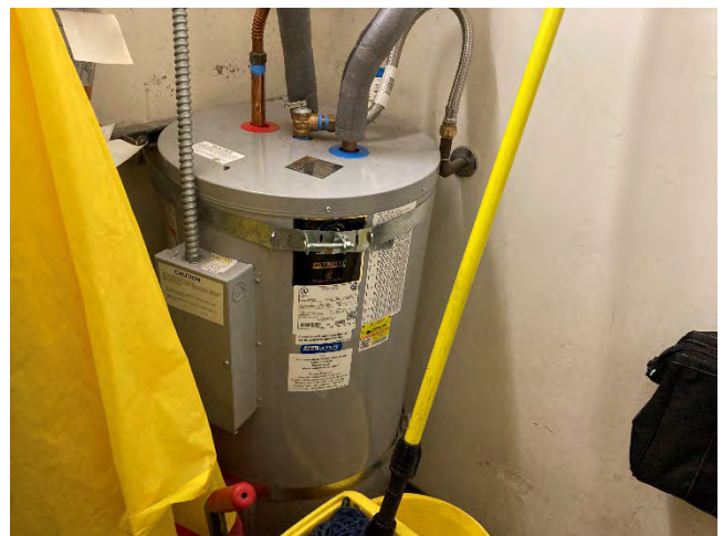
M-24. Electric domestic water heater.
