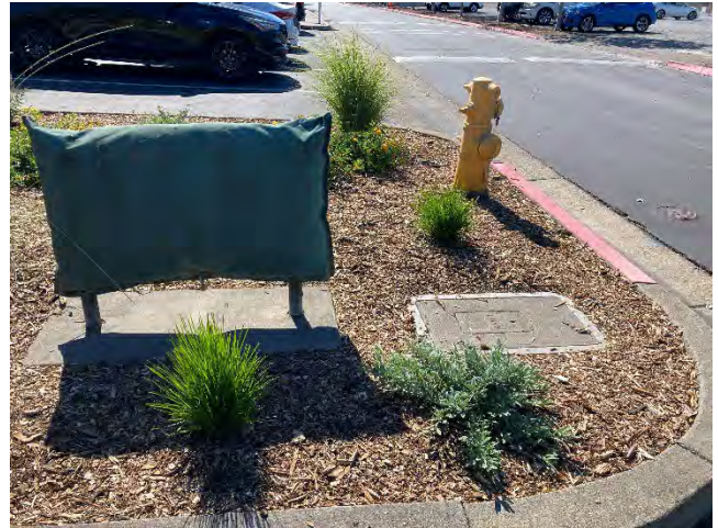
M-20. Domestic water service entrance.
