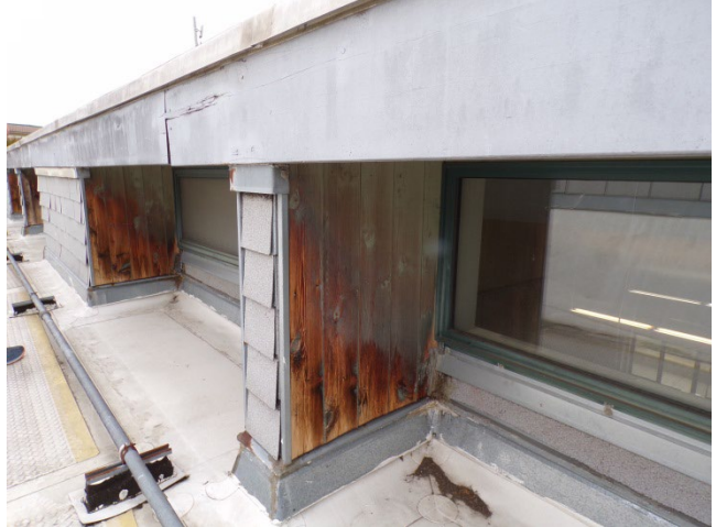
38. Main Bldg: Clerestory wood trim throughout is in a degraded condition.
