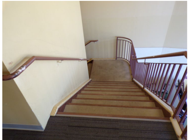
58. Gym: Entrance lobby unenclosed staircase. Minor damage to some paint finishes shown.
