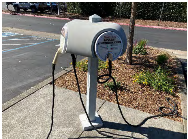
M-18. Electric vehicle charging station.
