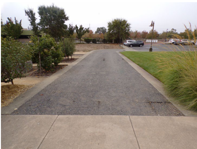
77. The short drive near the southeast corner of he Main Bldg requires gravel replenishment.
