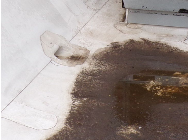
91. Main Bldg: A leak was reported near this scupper above the northwest wing.
