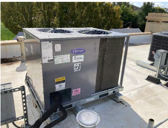
M-5. Main Bldg: Split system air conditioning condenser.
