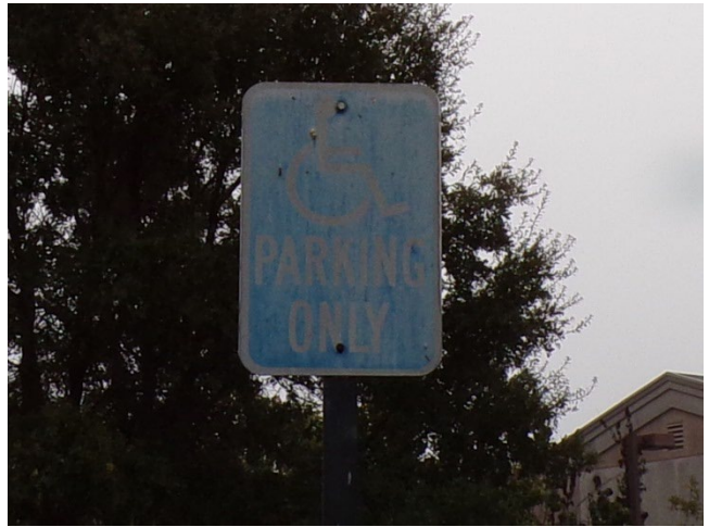
82. Accessible parking signage is typically in a degraded condition.
