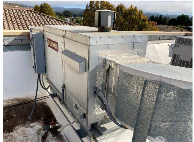
M-8. Main Bldg: Natural gas-fired kitchen make-up air unit.
