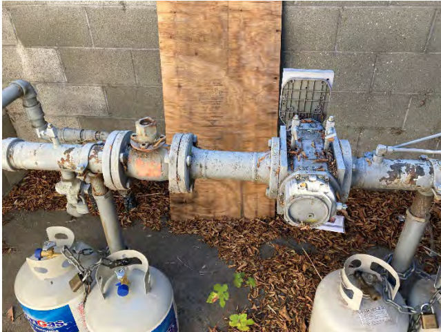
M-19. Natural gas service entrance.
