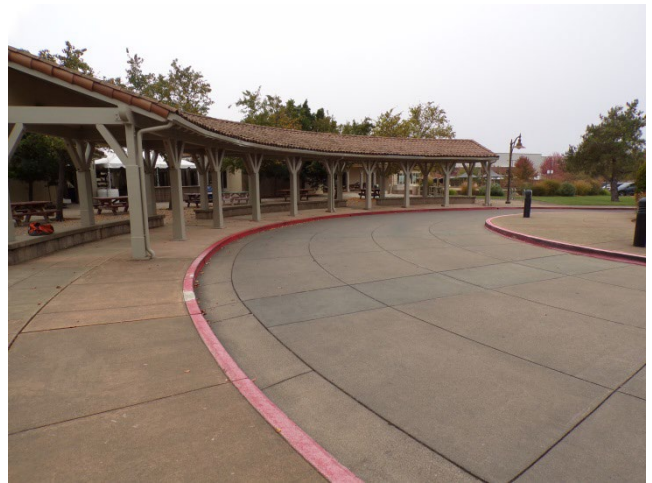
10. Main Bldg: Afternoon student pick-up shade shelter and drive aisle. Accessible pick-up areas are not provided at either the north (shown) or south student drop-off areas.
