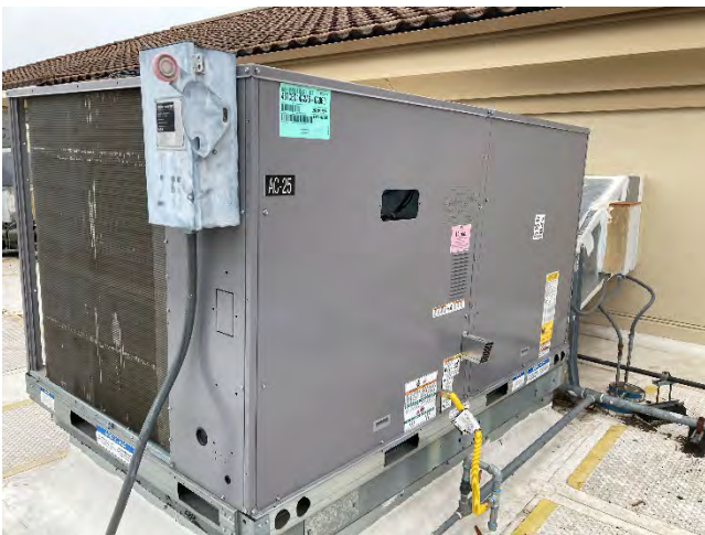
M-3. Main Bldg: Packaged air conditioner.
