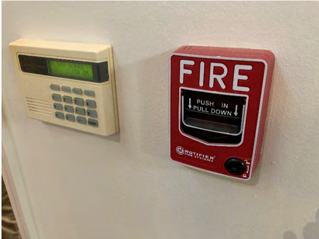
M-31. Key pad security panel.
