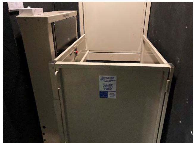
M-34. Main Bldg: Theater wheelchair lift.
