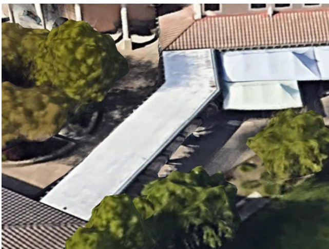
89. AllWest recommends that the BUR system on the covered walkway be replaced.
