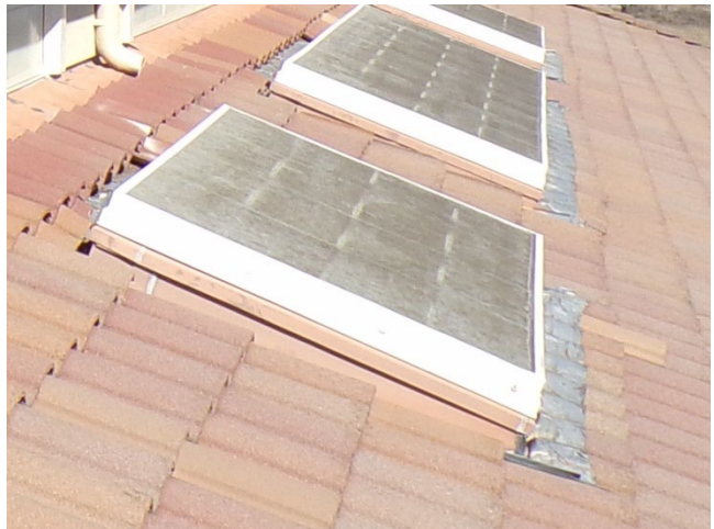
40. Gym skylights with deteriorating fiberglass panels.
