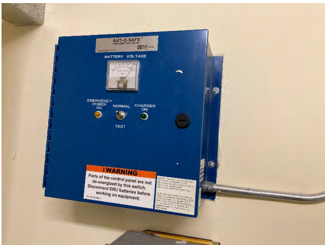
M-33. Elevator battery emergency recall panel.
