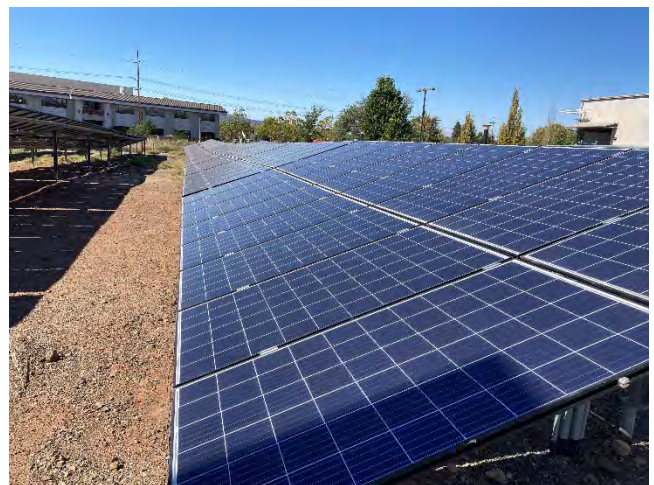
M-12. Solar photovoltaic power generation panel array.
