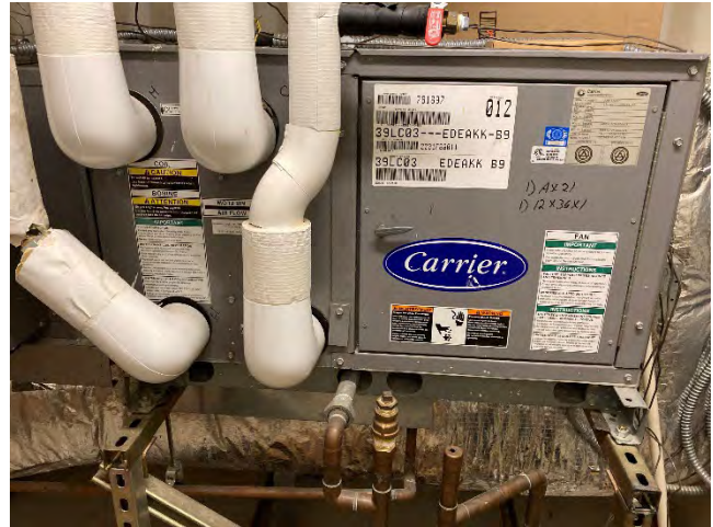
M-2. Gym: Four-pipe fan coil unit.
