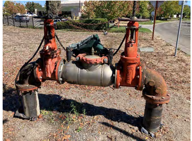
M-26. Fire sprinkler service entrance.
