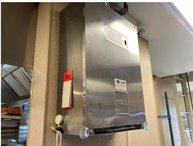
M-29. Kitchen hood fire suppression tank.
