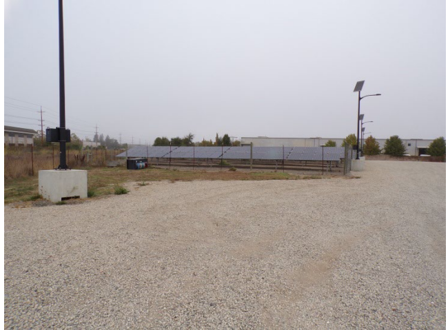
32. Solar array at west edge of property, looking north.
