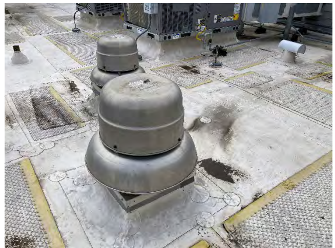
M-10. Main Bldg: Rooftop exhaust fans.
