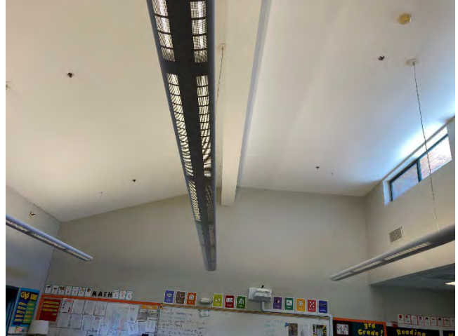
M-14. Main Bldg: Classroom light fixtures.
