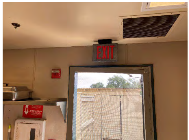
M-30. Illuminated exit sign and horn/strobe.
