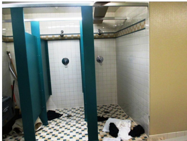
75. Gym showers do not meet Accessibility requirements.
