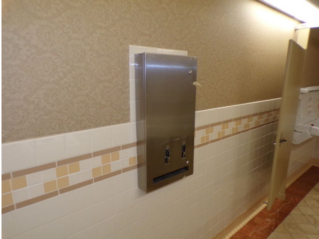
73. Main Bldg. The sanitary napkin dispenser in the adult women's restroom is not Accessibility compliant.
