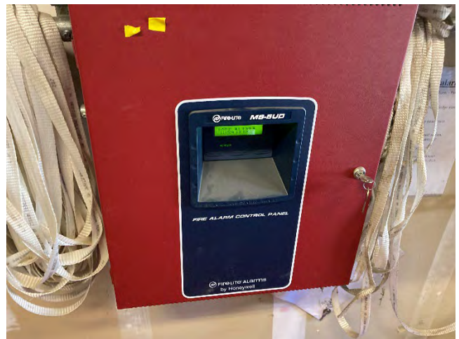
M-28. Fire alarm panel.
