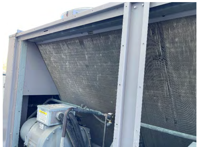
M-6. Gym: Air-cooled chiller.
