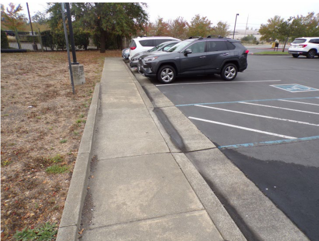
83. Truncated domes are not installed in any required location at the school.
