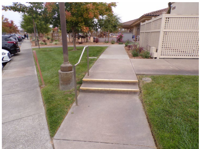
78. Main Bldg: The stairs near the southwest corner of the building have a handrail on one side only. Tread striping should be renewed.
