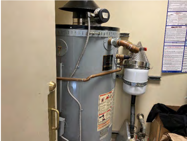
M-25. Natural gas domestic water heater.
