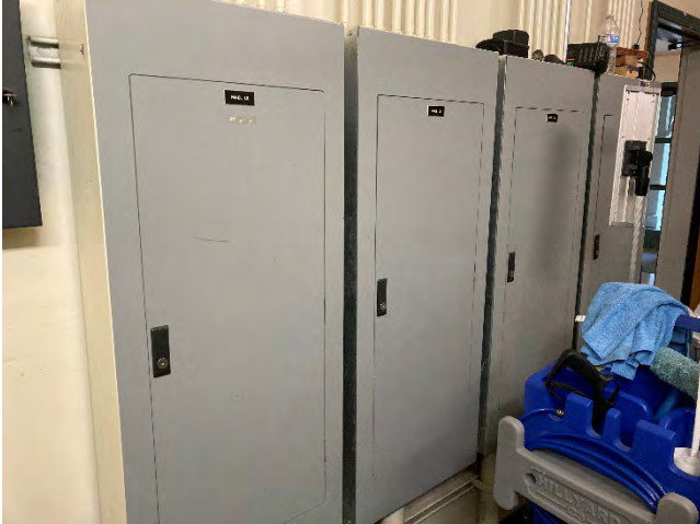
M-13. Electrical distribution panels.
