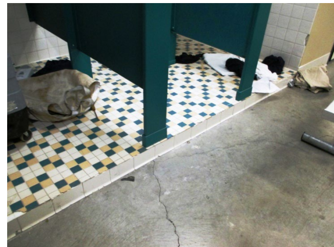
66. Gym: Locker room showers do not meet Accessibility requirements.
