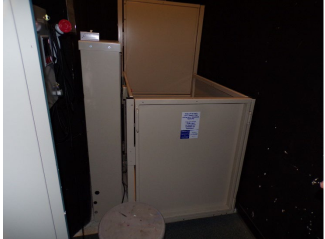
68. Main Bldg: Stage lift at auditorium provides access from seating area level to stage level.
