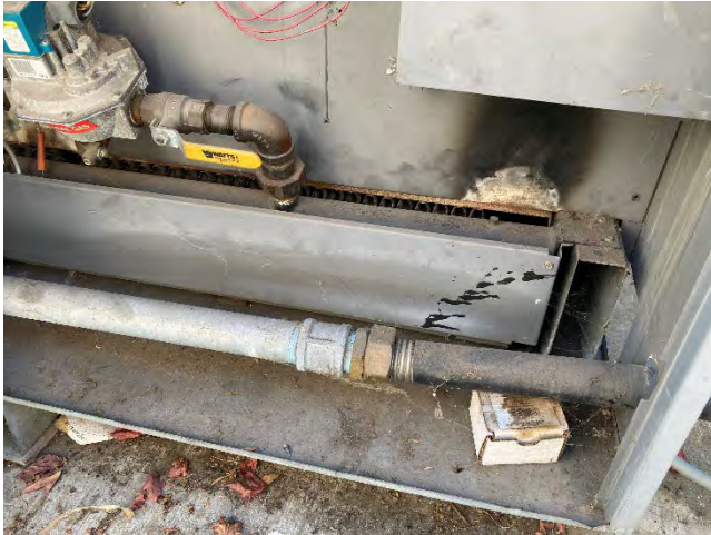
M-7. Gym: Natural gas-fired boiler.
