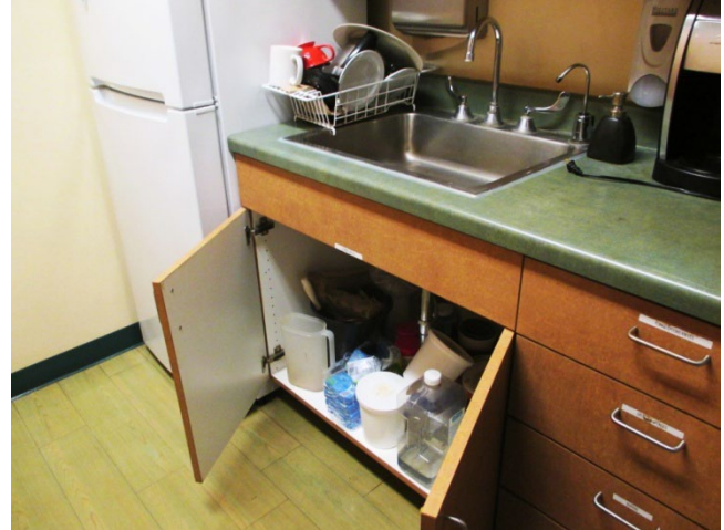
74. Main Bldg: Service sinks at several locations are inaccessible to a wheelchair occupant. Administarion area break room shown.
