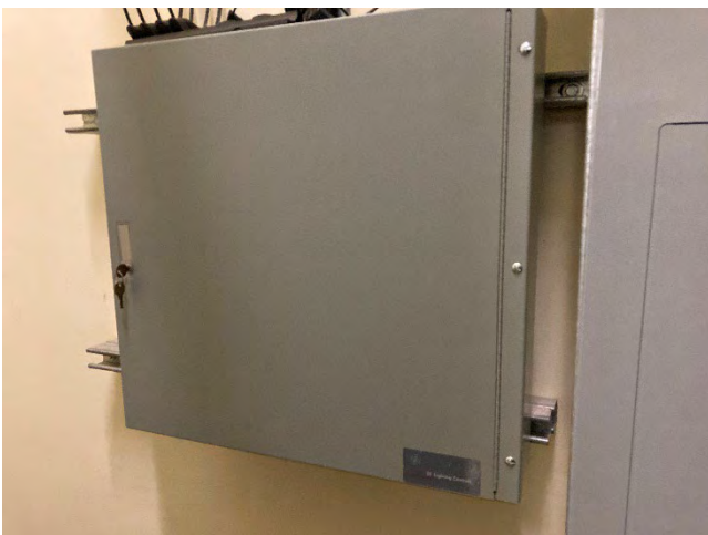
M-17. Main Bldg: Lighting control panel.
