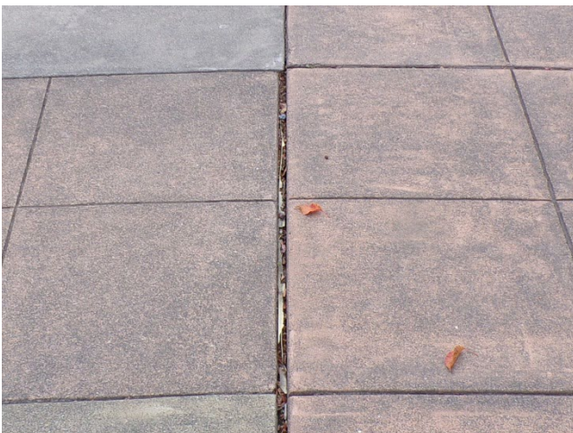
23. Degraded plastic control joint caps are recommended for replacement.
