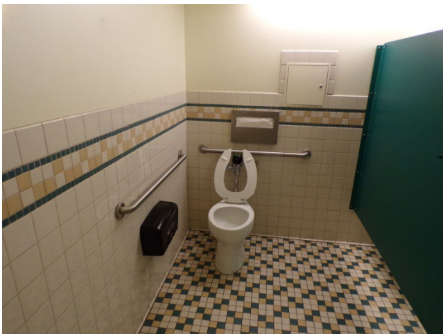
71. Accessible toilet stalls generally meets code requirements; Main Bldg restroom shown.
