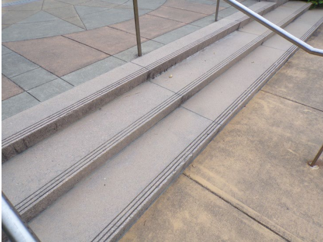
85. Main Bldg: Grooved stripes in stair treads are no longer compliant with current Accessibility codes.
