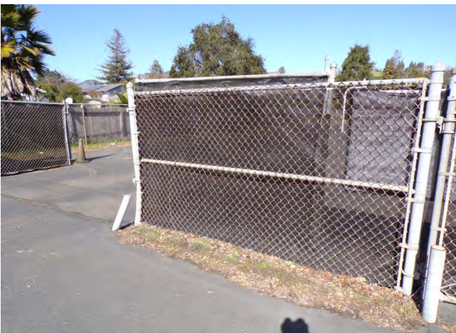
113. The perimeter chain-link fencing is in a degraded condition. Bent pole and rusted chain-link shown.
