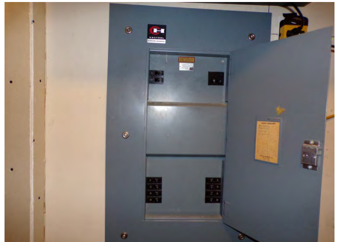
100. Rectory: Two main service panels, each rated at 100 amps, are installed (one shown).
