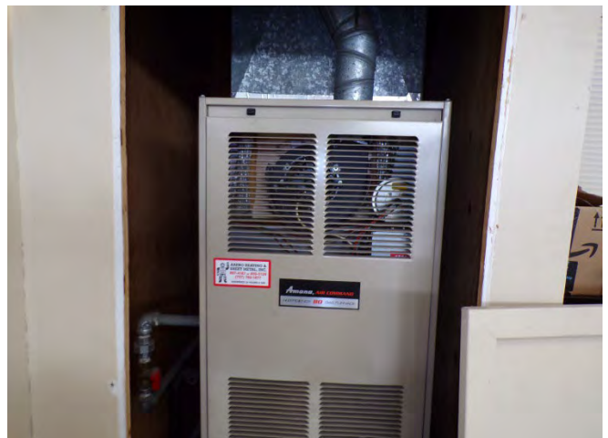
96. School: Each of the eight classrooms has a natural gas-fired furnace for space heating.
