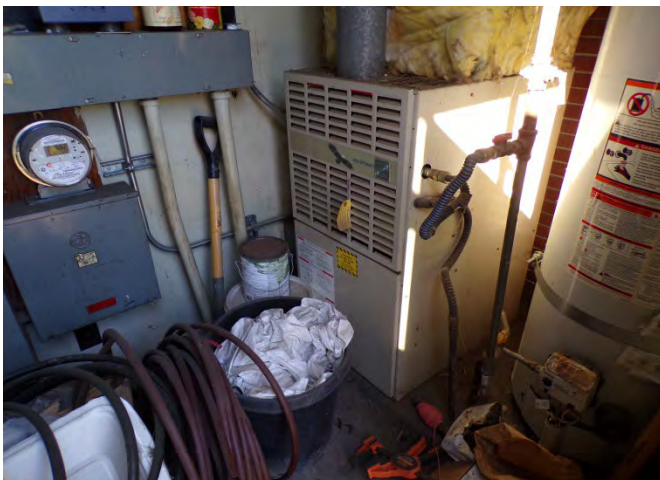
95. School: One natural gas-fired furnace provides heat to the office area.
