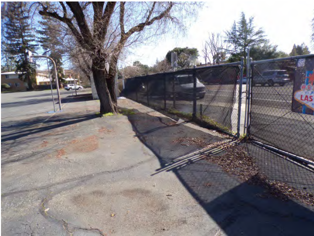
29. Upheavals and depressions in asphalt paving.
