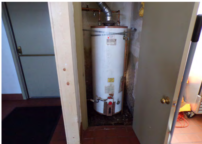
107. Hall Bldg: The 50-gallon natural gas-fired water heater was manufactured in January of 1982.
