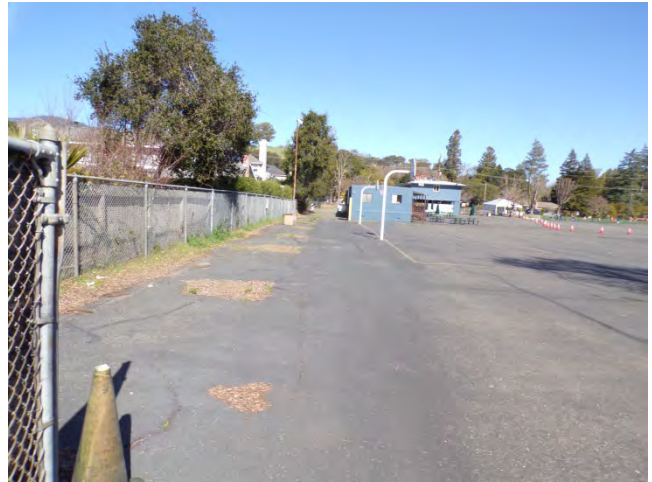
28. Along the west site perimeter, voids in the asphalt paving were observed. AllWest presumes that plants were once installed in these voids.
