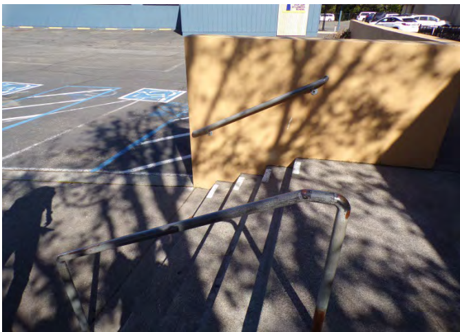
119. Railings at exterior stairs are not compliant with current Accessibility requirements. (Church shown.)
