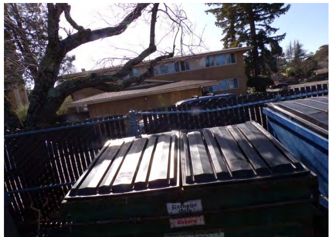
114. Bent chain-link fencing horizontal support at trash enclosure.
