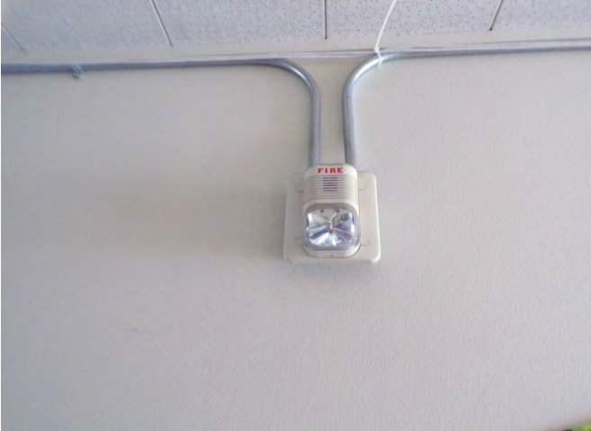
109. Convent: Horn/strobe alarm devices are installed in this building.
