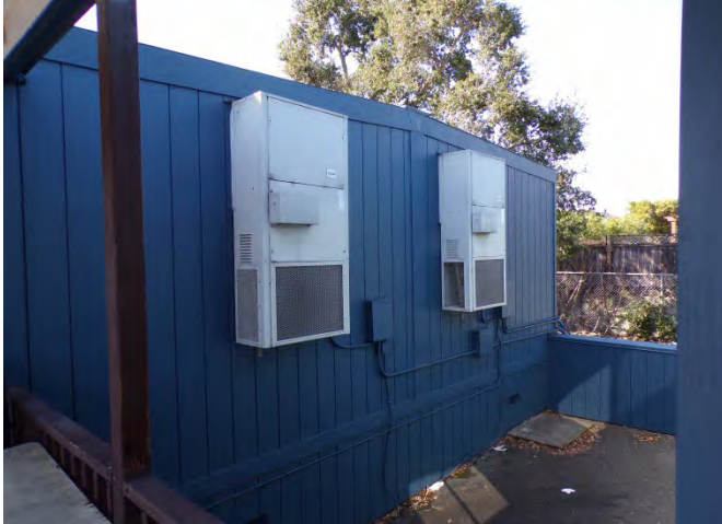
97. Mod Bldgs: Each Mod Bldg has two ZoneAir electric furnaces. Age and heating capacity are unknown.
