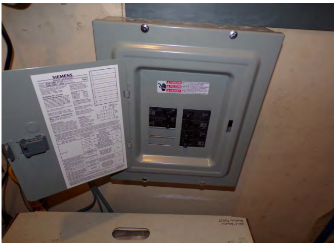
101. Rectory: A sub-panel rated at 125 amps is also installed in this building.
