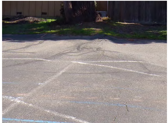
30. Upheavals and depressions in asphalt paving.
