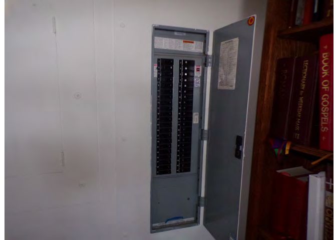
98. Church: The main electrical service entrance panel is rated at 225 amps.
