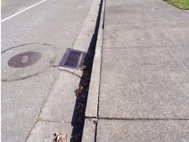
19. Changes in elevation in excess of ¼" create tripping hazards.
