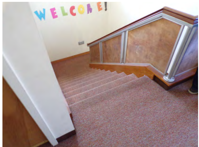
66. Convent: Two sets of interior stairs are provided. Stairs lack compliant visually contrasting striping at top and bottom treads. Compliant handrails are not provided.
