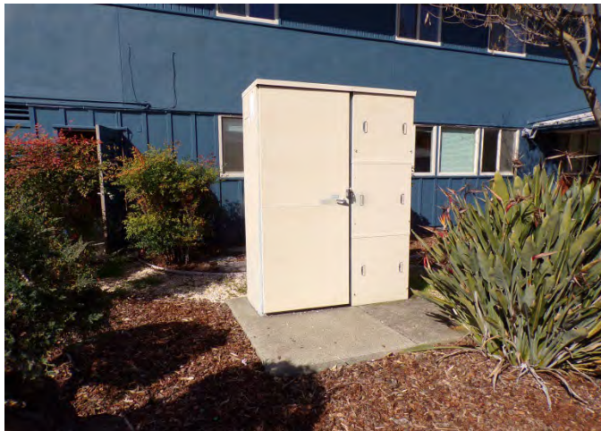
105. Convent: A locked PG&E enclosure near this building presumably contains the main electrical switchgear for the property.
