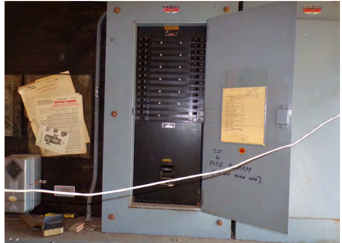
104. Convent: The main electrical service entrance panel is rated at 200 amps.
