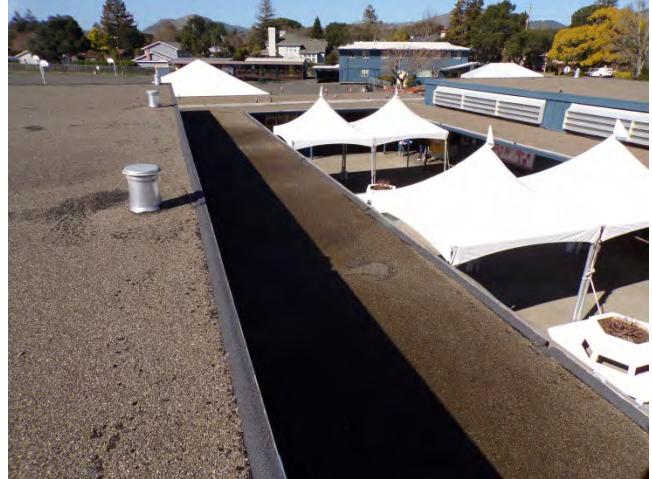
44. School: Replacement of this roofing sytem—and those on all other buildings—is recommended during the reserve term.
