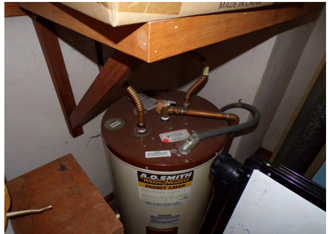
106. Church: The 20-gallon electric water heater has seismic strapping. This unit was manufactured in December of 1995.
