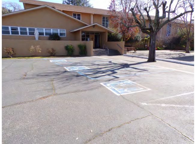
32. Accessible parking stall striping and pavement markings are in a degraded condition. Accessible stalls also lack required signage.
