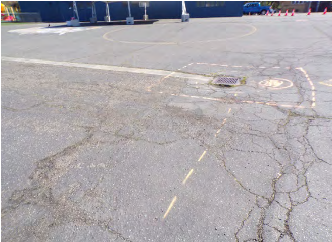
111. Flooding in the parking lot was reported during recent heavy rains at this area drain.
