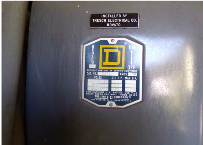
103. School: The main electrical service entrance panel is rated at 200 amps.
