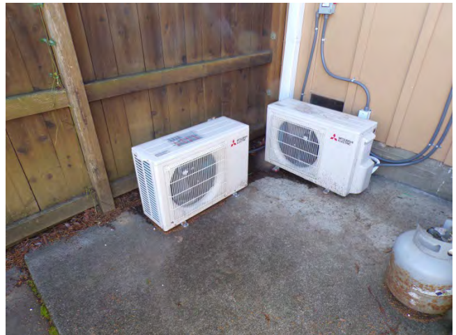
90. Rectory: Three split-system heat pumps were manufactured by Mitsubishi in 2022 (two shown). They provide heated and cooled air.
