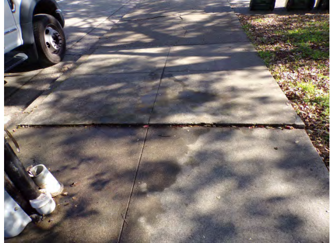
20. Changes in elevation in excess of ¼" create tripping hazards.
