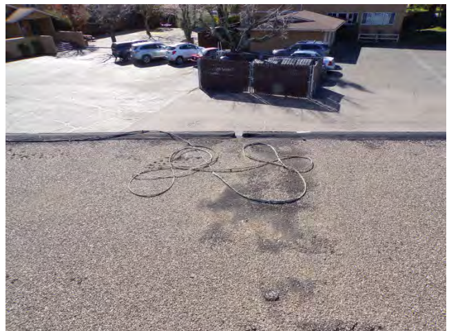
42. School: A modified bitumen roofing system with pea gravel ballast is installed. Area where ballast is absent shown.
