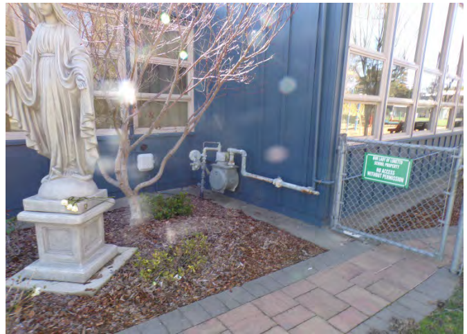
118. Each of the five primary buildings has a gas meter; automatic seismic shutoff valves are not installed at any meter. (School shown.)
