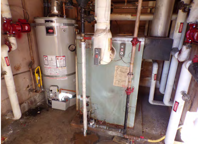
91. Rectory: A natural gas-fired boiler provides hot water to a hydronic loop heating system. The boiler has a rigid gas line connection.
