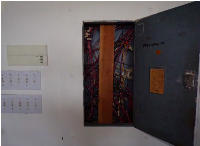
99. Church: This electrical panel is lacking an interior cover plate.
