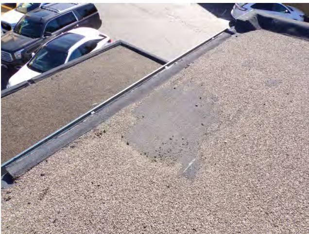
41. School: A modified bitumen roofing system with pea gravel ballast is installed. Area where ballast is absent shown.
