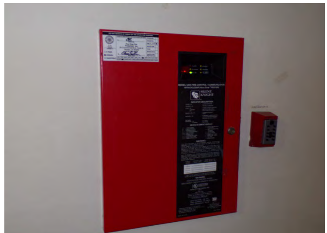
108. Convent: This is the only building to have a fire alarm panel installed.
