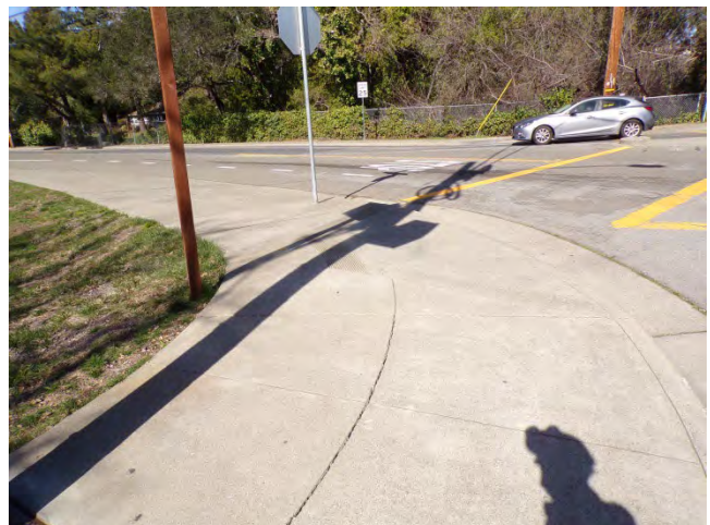
24. Truncated domes are not installed at the curb ramp at the intersection of Grant and Virginia Avenues.
