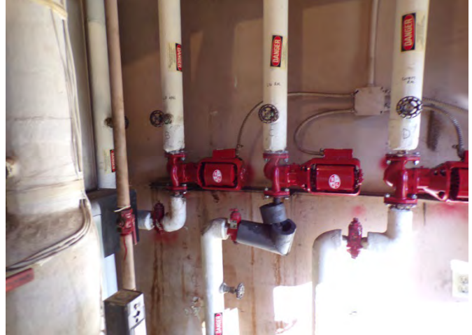
92. Rectory: Five circulation pumps for the hydronic loop system were replaced in December 2022 (three shown).
