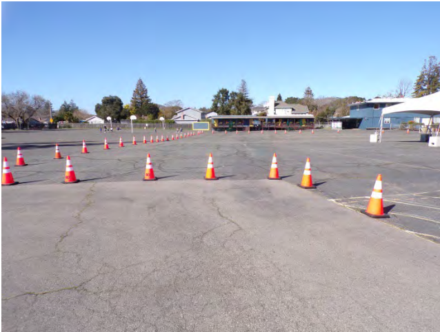
27. The asphalt paving is in a generally degraded condition.
