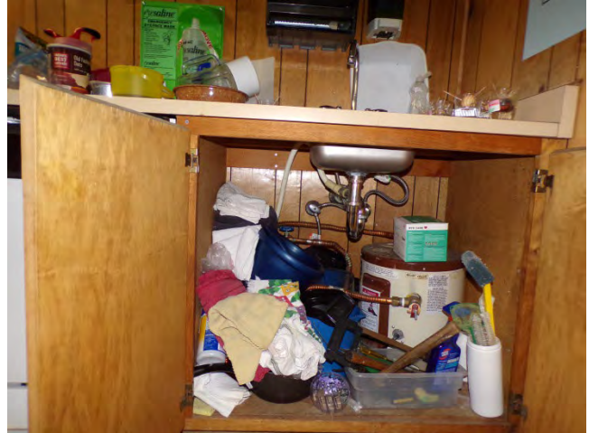
68. Mod Bldg N: An electric water heater of unknown age is installed in this modular building.
