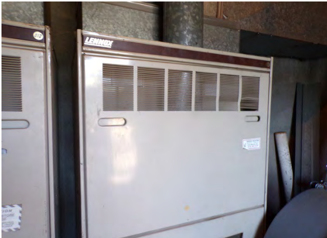
93. Hall Bldg: Two Lennox natural gas-fired furnaces provide heat.
