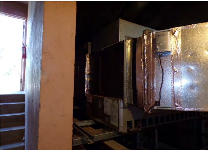
89. Church: Two Reznor natural gas-fired furnances, manufactured in November of 2011, provide heat.
