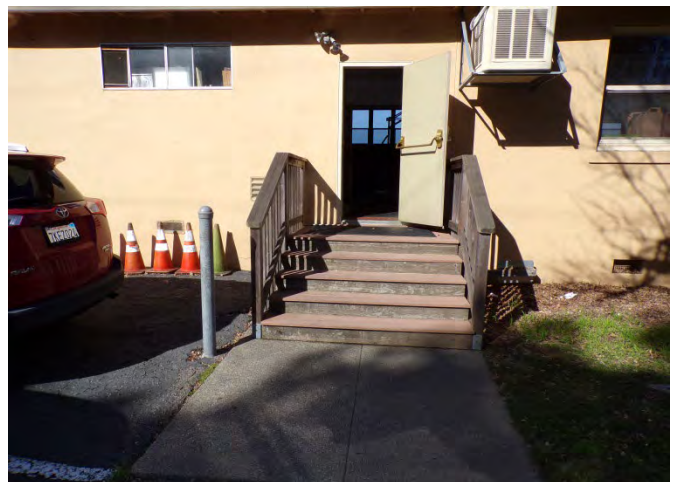
120. Railings at exterior stairs are not compliant with current Accessibility requirements. (Hall Bldg shown.)
