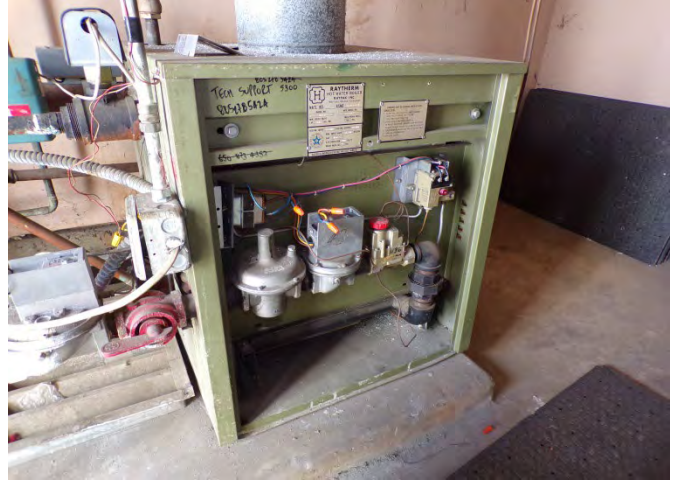
116. Convent: The hot water boiler likely dates to original construction in 1958. It has a rigid gas line connection.
