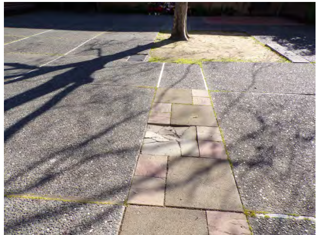
22. Degraded courtyard paving.
