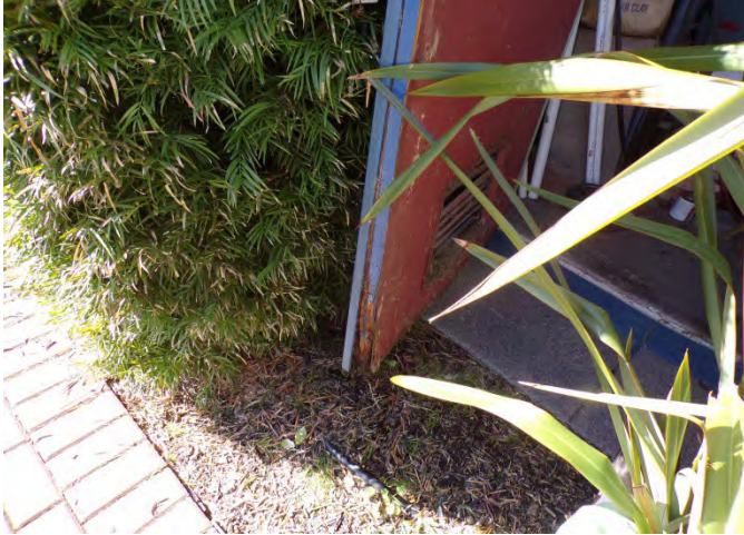
115. Some exterior doors are in a degraded condition and should be replaced. (School shown.)
