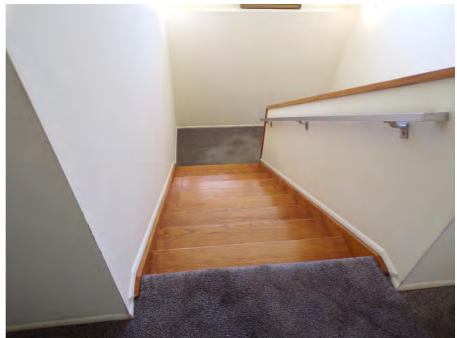
54. Rectory: Two sets of interior stairs are provided. Stairs lack compliant visually contrasting striping at top and bottom treads. Non-compliant handrails are installed.
