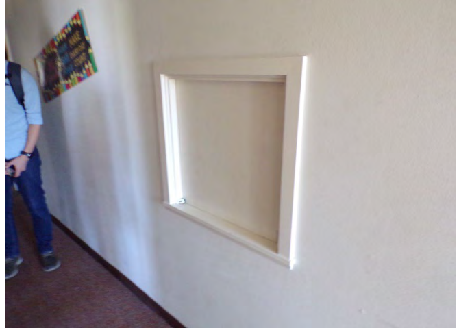
110. Dumbwaiters, which have been taken out of service, are installed in the Convent (shown) and the Rectory.
