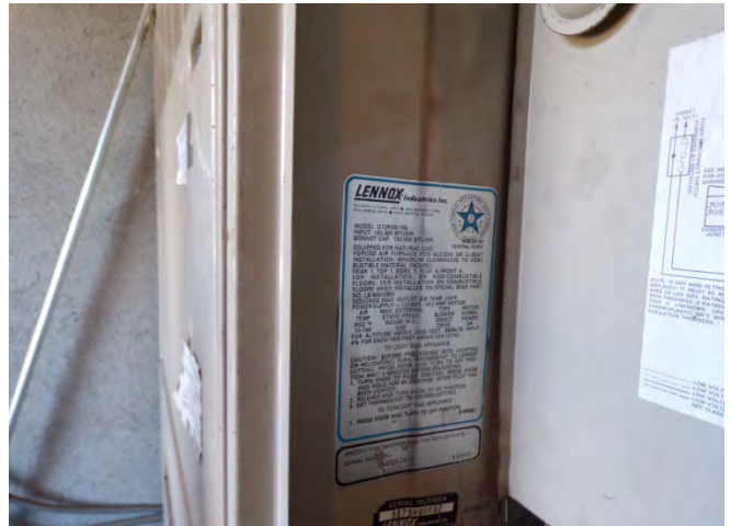
94. Hall Bldg: The Lennox furnaces were manufactured in October of 1975.
