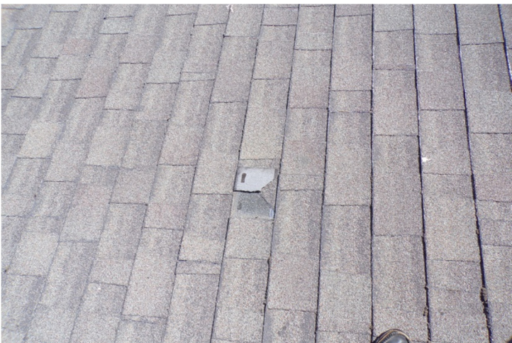
47. Asphalt composite shingles are provided above main level spaces on north side of building. Cracked and folded shingle shown.
