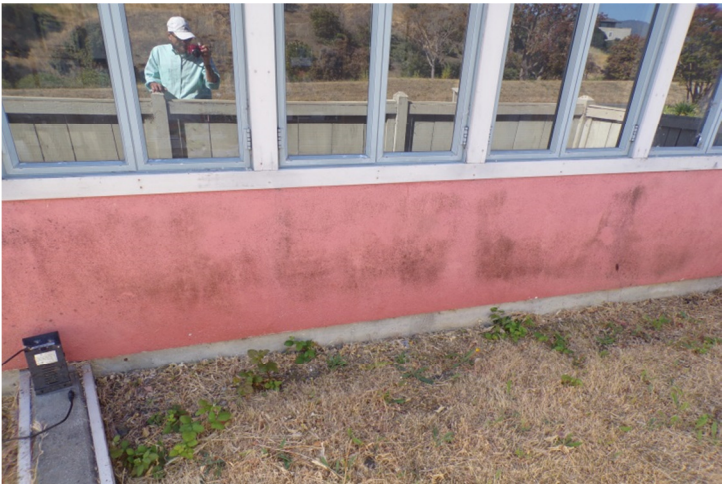
57. Exterior paint finishes will require repainting during the reserve term.
