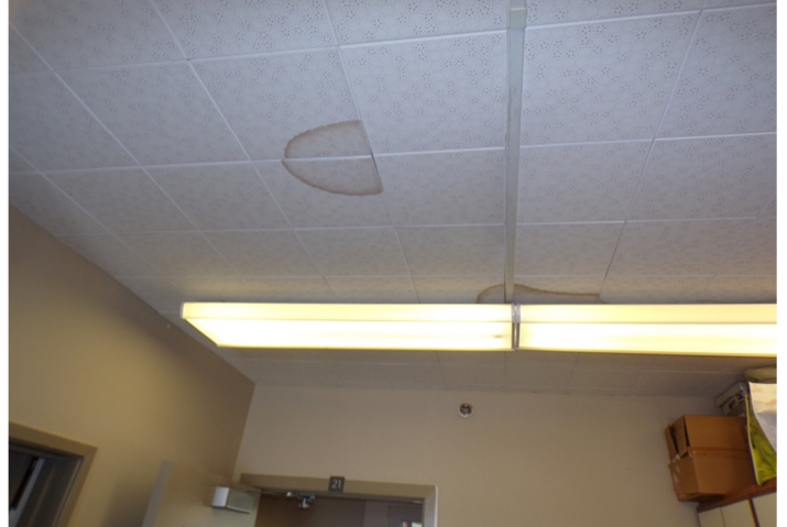
32. Water stained ceiling tiles were observed in a few locations.
