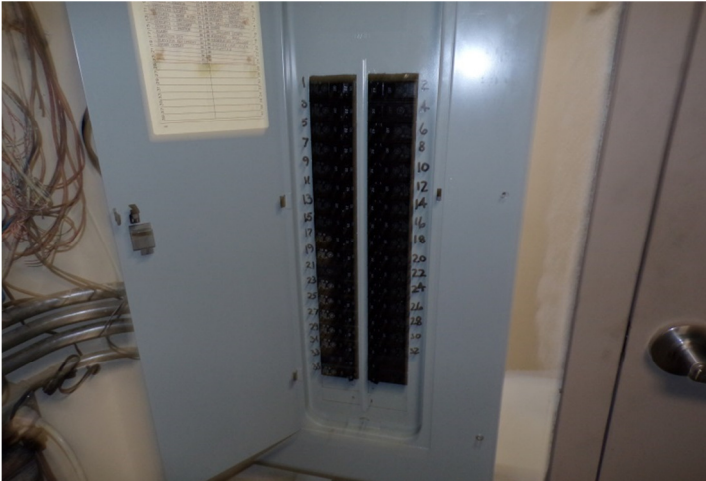
73. Infrared scanning of the electrical distribution system is recommended.
