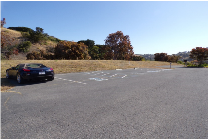
63. Path of travel pavement markings from north Accessible parking stall are lacking.
