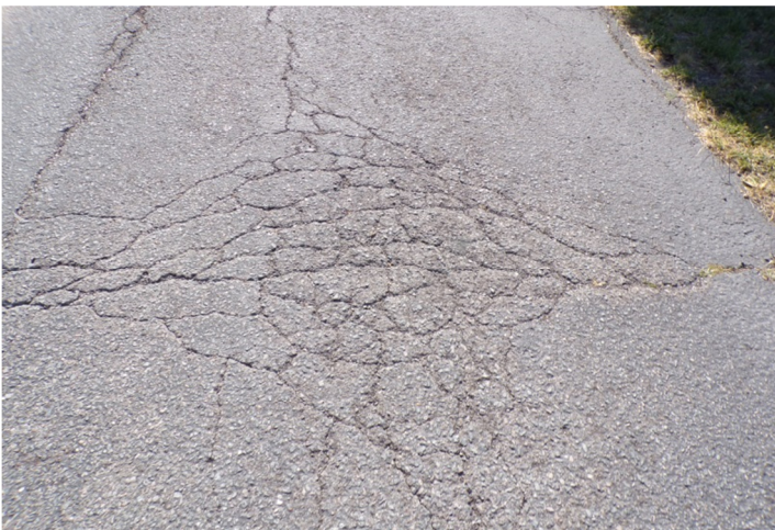
11. Degraded condition of asphalt surface of parking lot and drive aisles.
