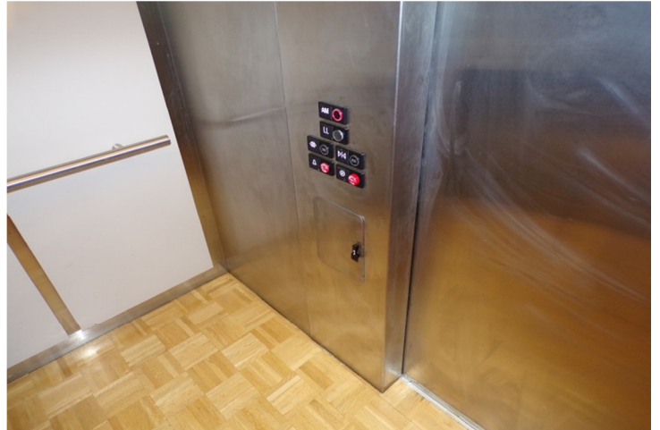
62. A hydraulic elevator is installed and serves the main and lower floor levels.
