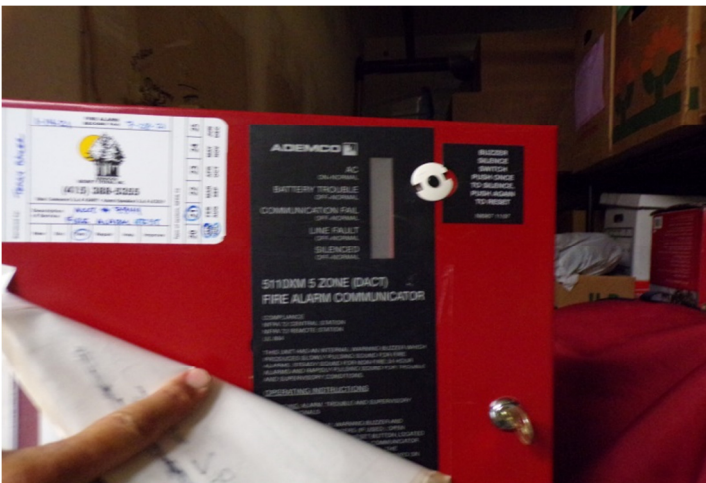
77. The fire alarm system was last inspected in April 2023.
