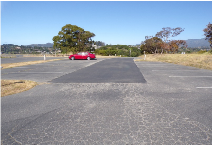
9. Typical view of parking lot, looking west. Large area of repair at center (darker asphalt). Alligator cracking in foreground.
