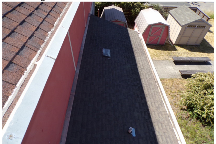
48. Asphalt composite shingles on lower-sloped pitched roofs are in a degraded condition. West side of building shown.
