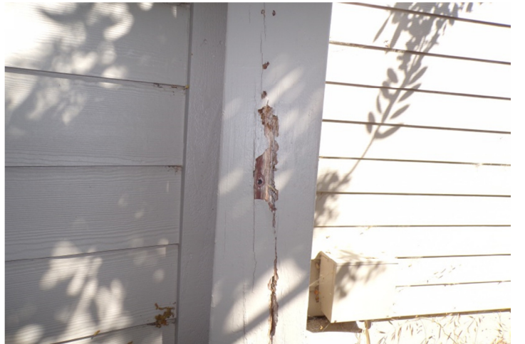
58. Rotten exterior wood building elements, such as the glulam columns pictured here, require repair or replacement.
