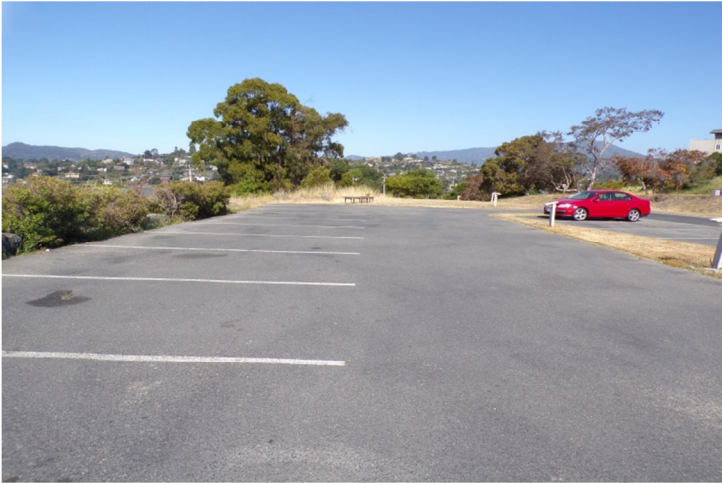
55. Non-Accessible parking stalls will require restriping during the reserve term.
