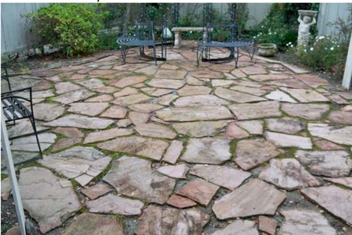
53. Tripping hazards were observed in flagstone paved courtyard (2016 photo).
