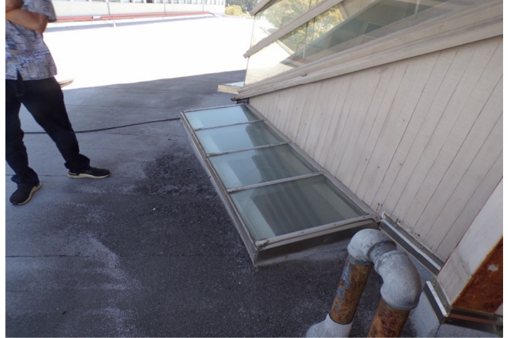
44. Two sets of aluminum framed skylights are installed in the vicinity of the Sanctuary on the roof above the main floor. Second pane from bottom is cracked.
