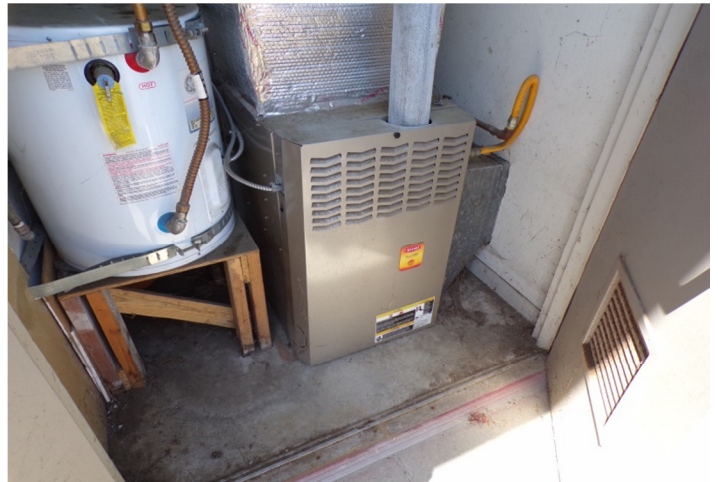
70. The older Bryant furnace dates to 2005.
