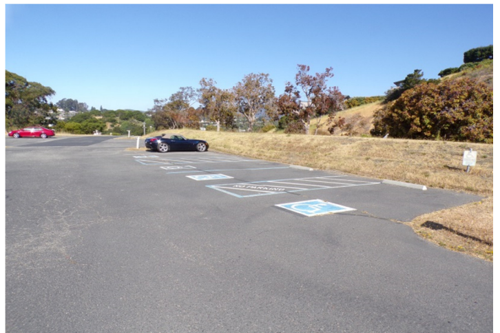
54. Accessible parking stalls will require new pavement markings and restriping during the reserve term.
