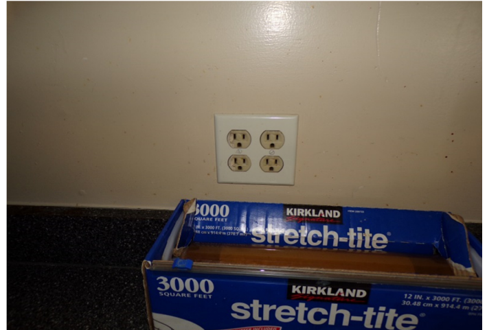
74. GFCI receptacles should be installed in required wet areas (kitchen on lower level shown) where conventional receptacles are currently provided.
