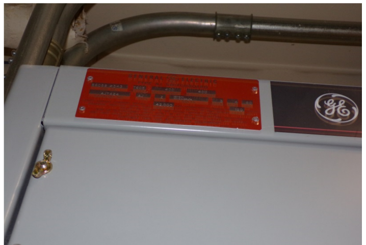
72. The GE main electrical service entrance panel is rated at 400 amps.
