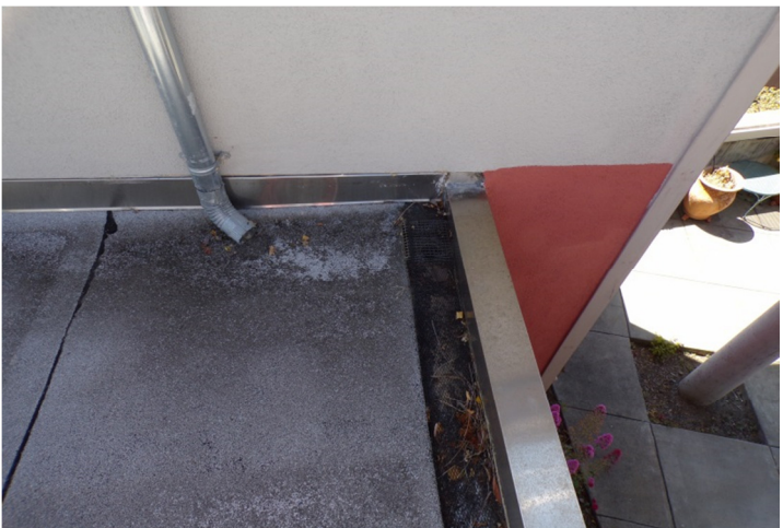
41. A drainage problem was described at this location adjacent to the elevator shaft (in background).
