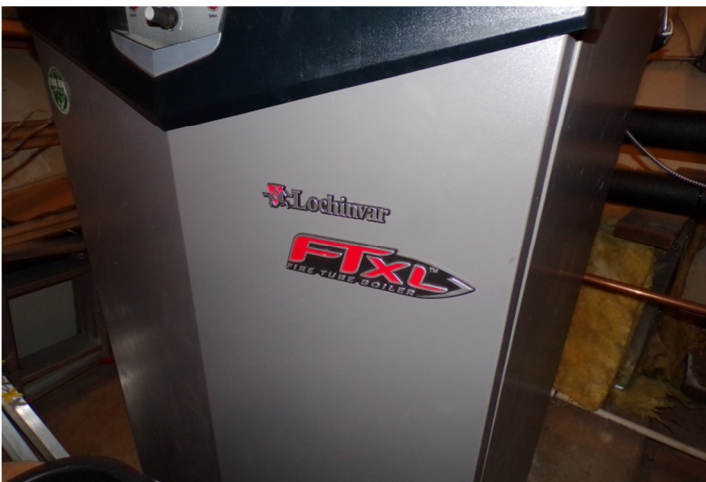
71. The Lochinvar boiler was installed in the main level mechanical room in 2017.
