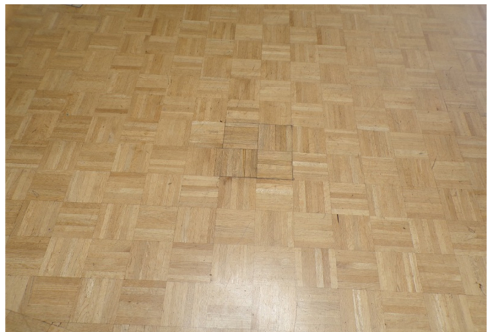
36. Degraded condition of parquet wood flooring at main corridor.
