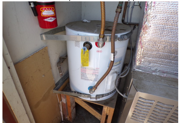
76. We recommend that all water heaters be replaced during the reserve term. Electric water heater in exterior service closet shown.
