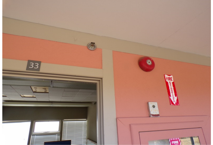
80. The building is fully fire sprinklered.
