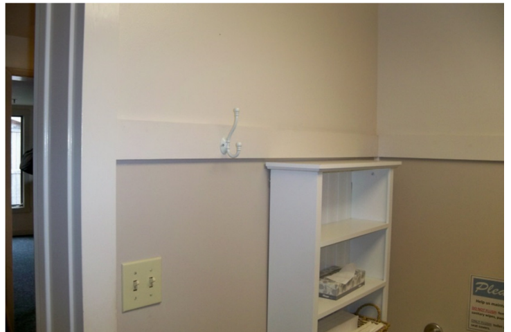
66. The coat hooks in the Accessible restroom are mounted too high (2016 photo).
