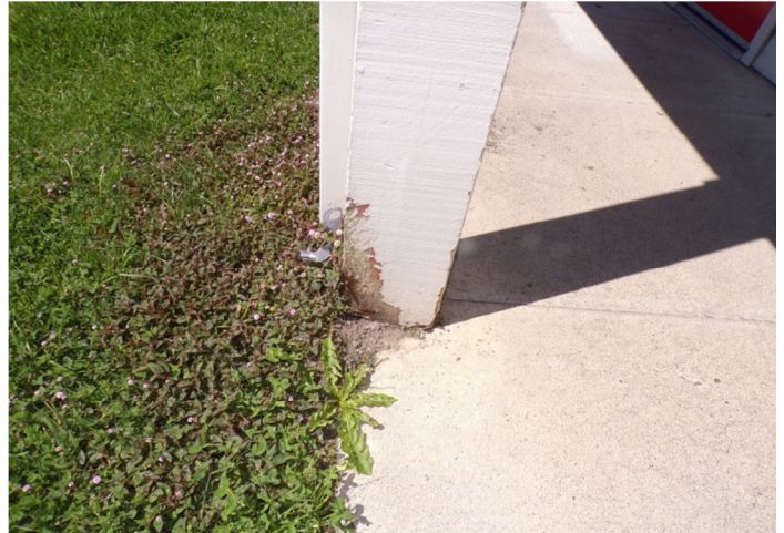
86. Degraded exterior wood was observed in several locations.
