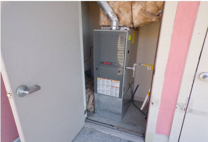
69. One 60,000 BTU/hr Trane furnace was installed in an exterior service closet in 2017.
