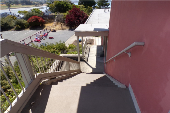
61. Both sets of exterior concrete stairs no longer comply with current building and Accessibility codes.
