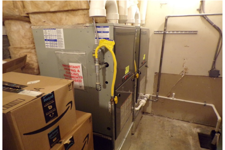
68. Two 100,000 BTU/hr Trane furnaces were installed in 2017 in an interior utility room on the lower floor.
