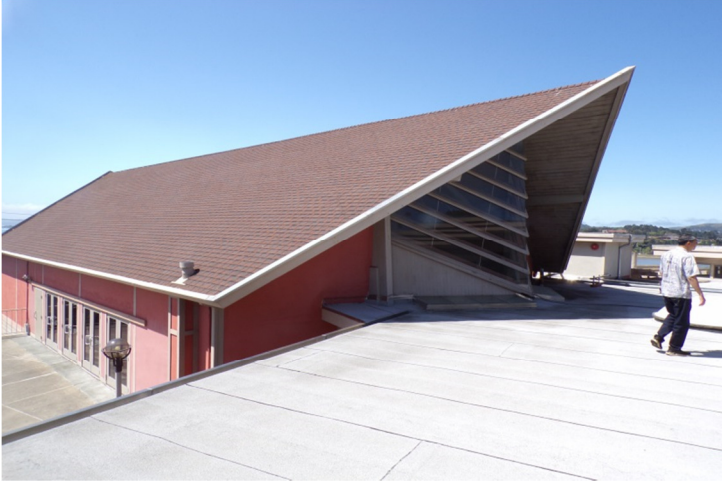
49. Asphalt composite shingles are provided as the roofing system above the Sanctuary.
