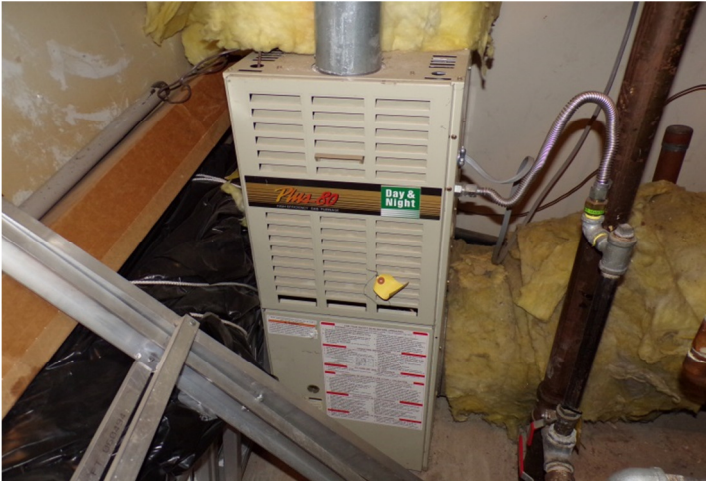
67. The older Day & Night furnace dates to 1996.
