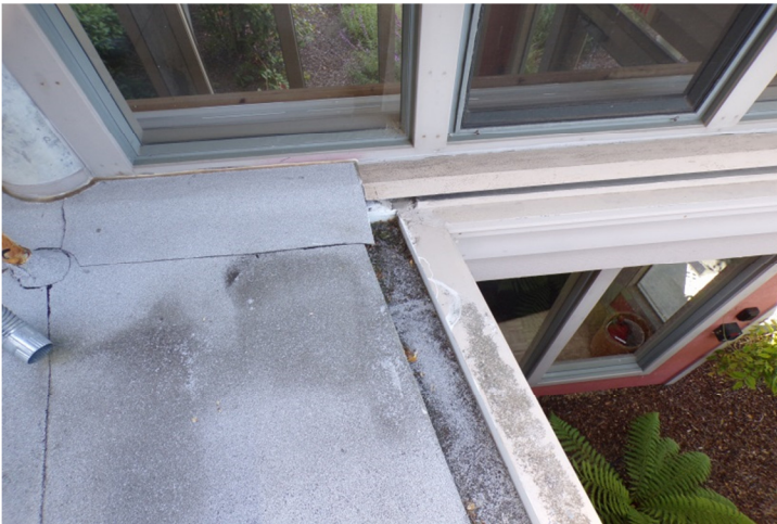
39. New BUR roofing systems were installed in September 2017. Mineral granule separation has already occurred.
