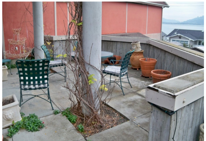
84. Possible differential settlement was reported at concrete-paved patio on west side of building (2016 photo).
