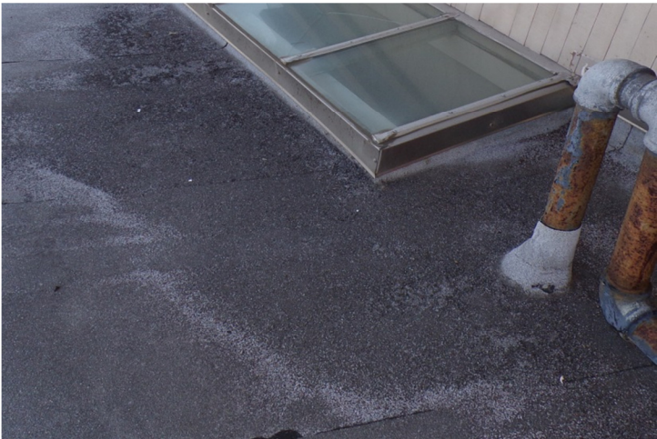
45. Roof adjacent to south end of Sanctuary: Evidence of past ponded water was observed.
