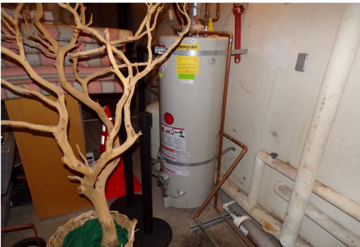
75. We recommend that all water heaters be replaced during the reserve term. Natural gas-fired water heater in main level mechanical room shown.
