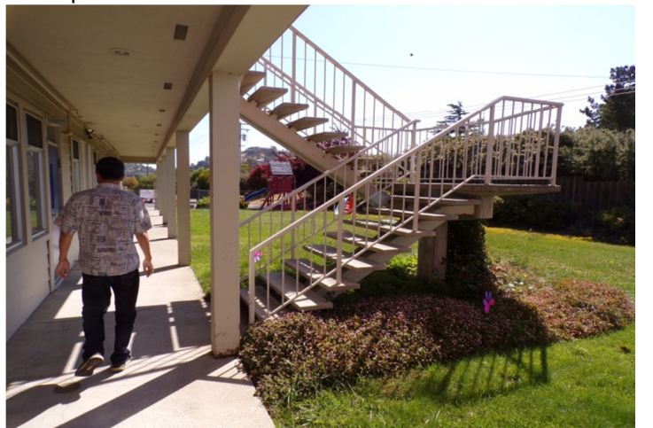
60. Both sets of exterior concrete stairs no longer comply with current building and Accessibility codes.
