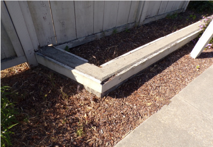
85. Degraded exterior wood was observed in several locations.
