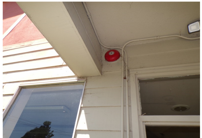
78. Exterior local fire alarm bell shown. Fire alarm device placements are not compliant with current Accessibility codes.
