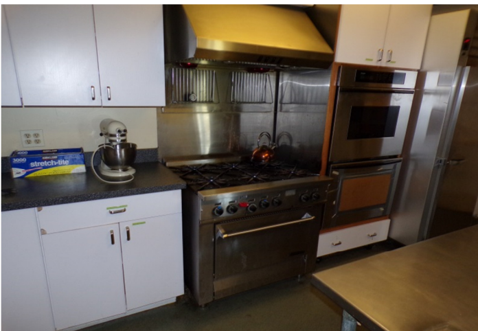
89. The vent hood over the gas stove is not fitted with an Ansul fire protection system.
