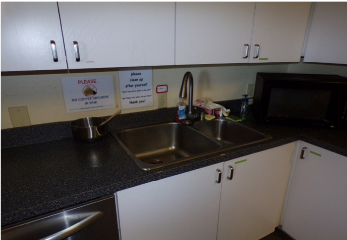
87. We recommended that low-flow restrictors be installed on sinks.
