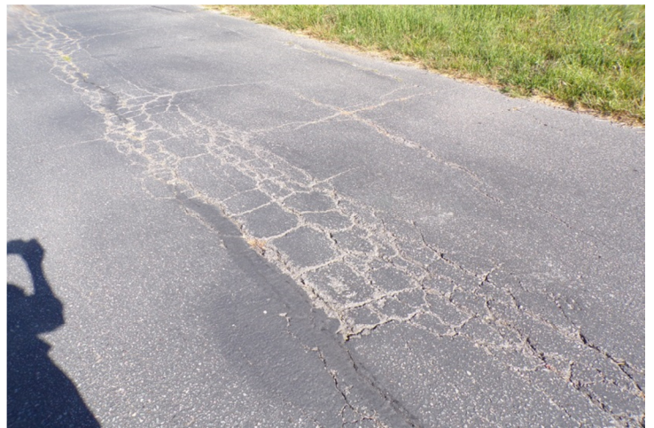
12. Degraded condition of asphalt surface of parking lot and drive aisles.
