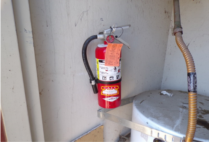
79. Several fire extinguishers were observed with expired inspection tags. The inspection date on this tag is July 29, 2021.
