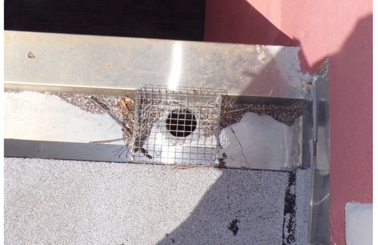
38. Roof drains are provided with wire screens; some were partially blocked with accumulated dead vegetation and other debris.
