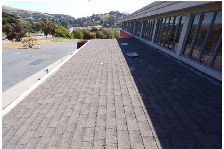
46. Asphalt composite shingles on lower-sloped pitched roofs are in a degraded condition. North side of building shown.
