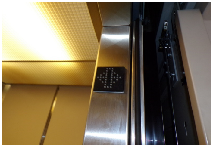
90. Elevator is not provided with Accessibility compliant audible tones.
