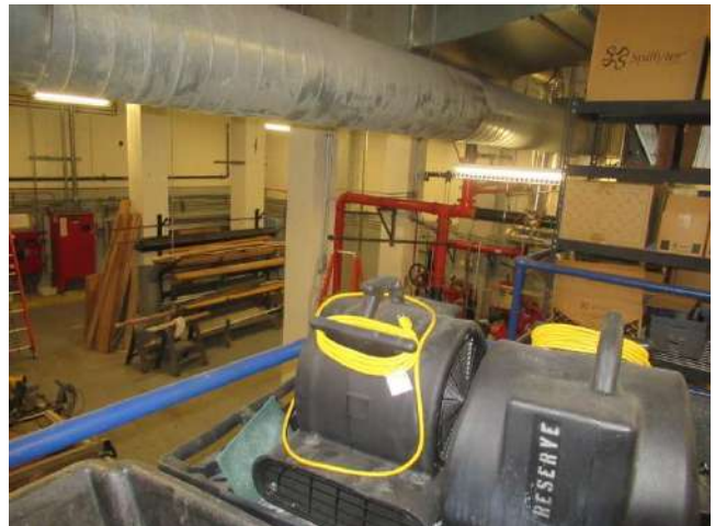
54. Main mechanical room at basement.
