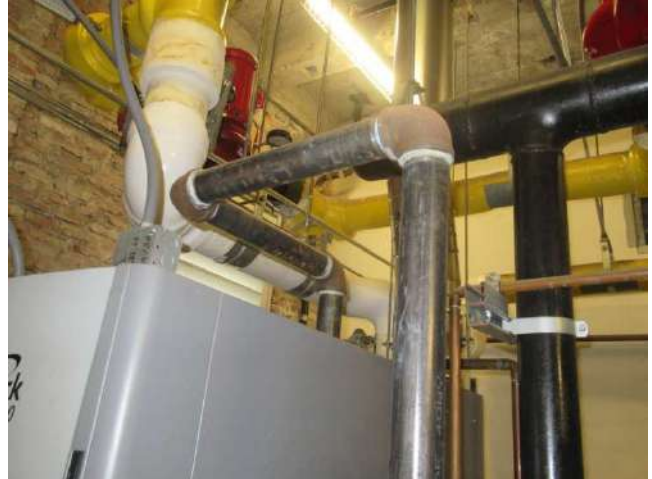
68. The gas supply to the boilers is the 2 1/2" diameter pipe in the foreground. A flexible connection to the boiler is not provided.
