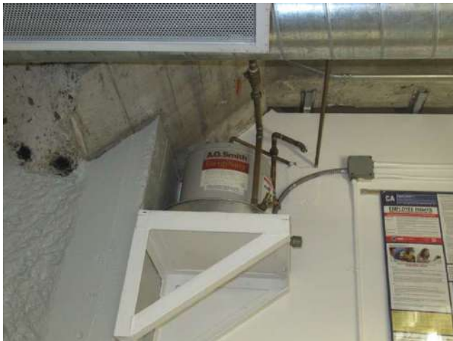
63. Small water heaters are provided for each sink in the building.
