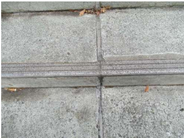
65. Elastomeric seals at the building stair entrances at east and west sides of building. No cracks or breaks were visible, but leaks were reported after power washing was done.
