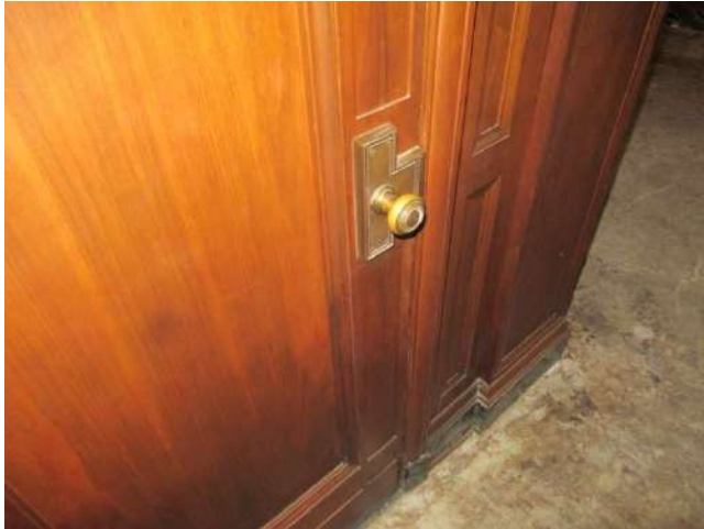
61. Non-compliant conventional door knobs are still installed at historic interiors.
