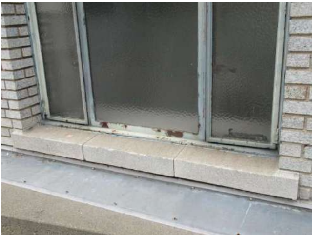
21. Window frames show considerable deterioration in some areas.
