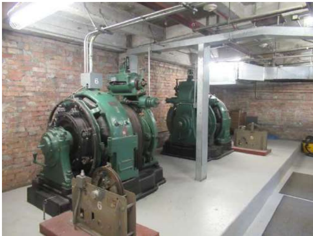
57. Traction elevator equipment at the penthouse level.
