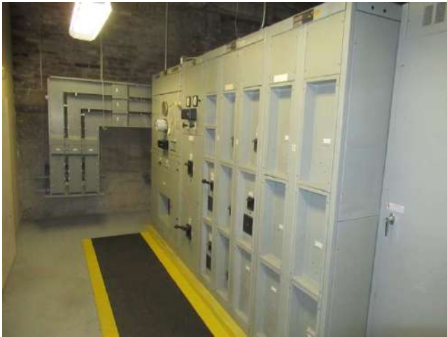
69. The main electrical panel for the building.
