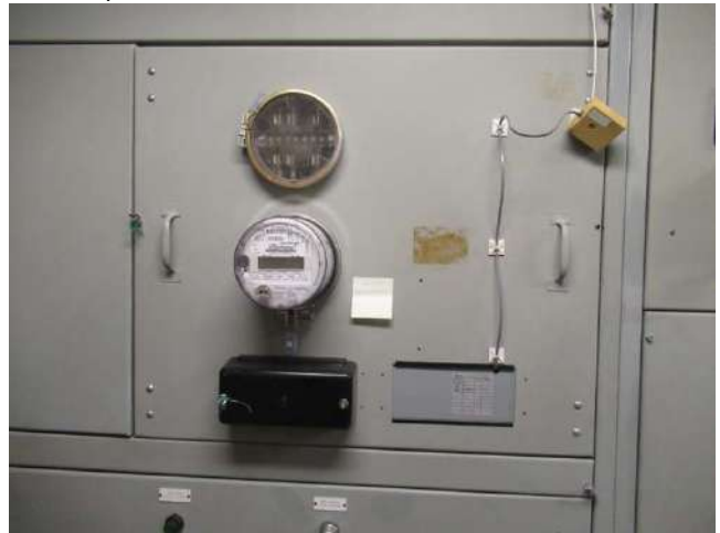
70. The main electrical panel for the building.
