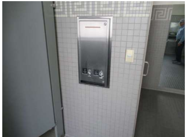
64. Non-compliant sanitary napkin dispensers that require grasping and turning motions to operate are still installed in women's restrooms.
