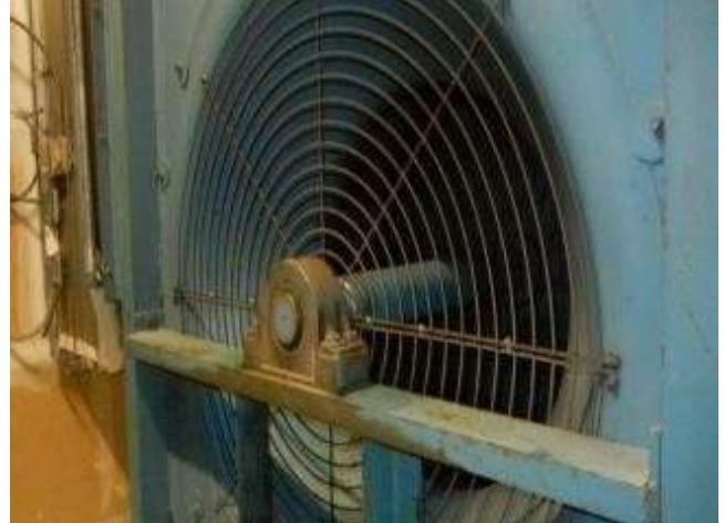
74. One of two supply air fans serving floors 1 through 7. Due to the age of the fans, shaft replacement should be anticipated during the reserve term. (2019 photo)
