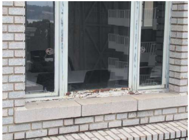
22. Steel window frames require refinishing in some locations.
