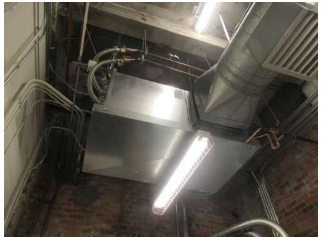
46. A water source heat pump was replaced in the penthouse in 2021.
