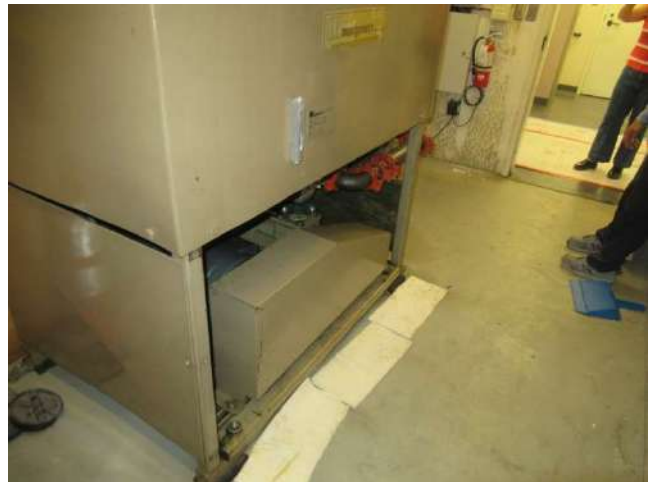
58. Hydraulic elevator equipment in the basement.
