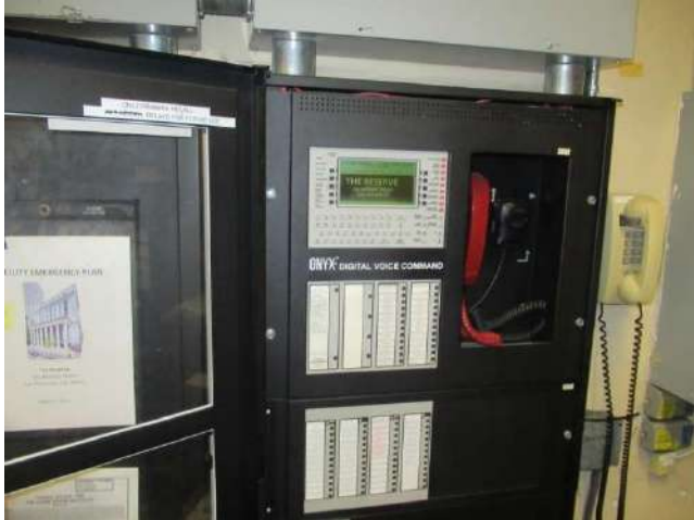
73. The building Fire Alarm Control Panel (FACP).
