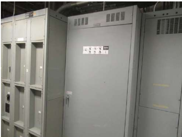
71. An Automatic Transfer Switch (ATS) is provided adjacent to the main electrical entrance. If the power supply goes out it starts the building generator.
