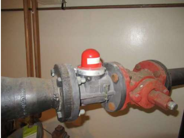
67. The automatic seismic shutoff valve is provided at the gas service entrance.
