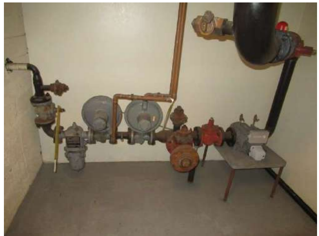
66. Gas service entrance in the basement.
