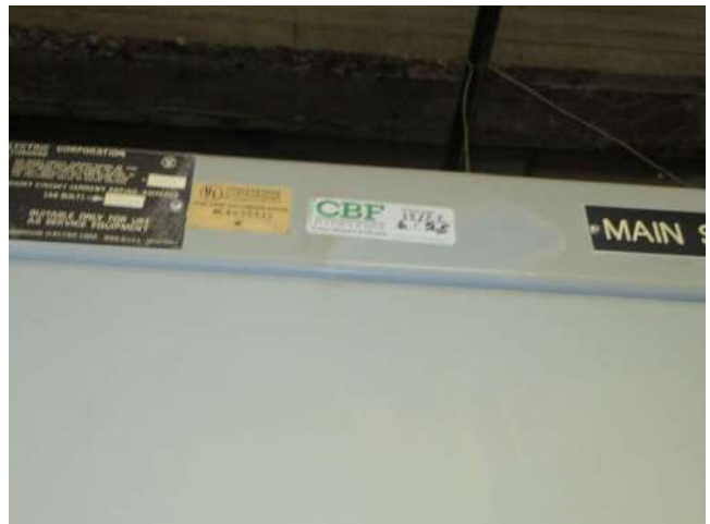
72. CBF provides infrared scanning of electrical systems on a triennial basis.
